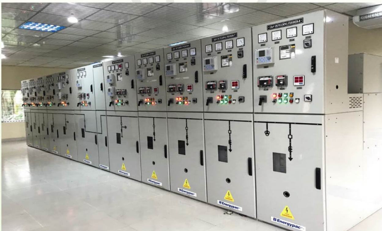
Control Room of Newly Constructed Bhola 33/11 kV Substation
