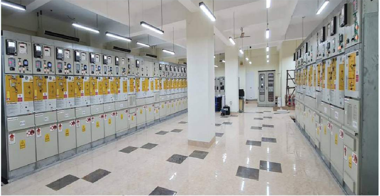
Newly Constructed Kushtia Campus, Kushtia 2*20/26.66 MVA 33/11KV GIS Substation under "Expansion & Upgradation of Power Distribution System Project"
