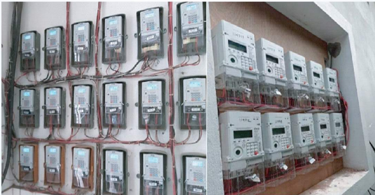
Installed Pre-payment Meter under "Smart Prepayment Metering Project for West Zone Power Distribution Company Ltd. (WZPDCL) Area" project.
