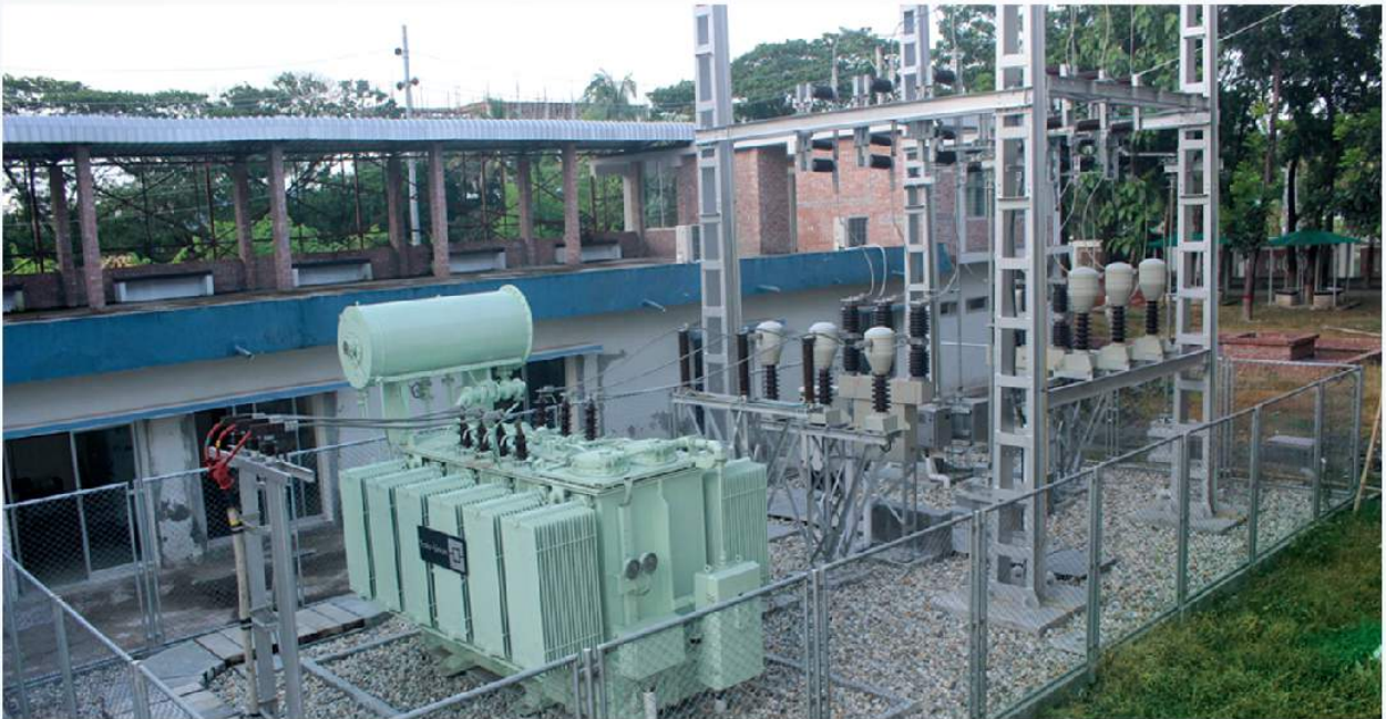
Newly Constructed Model Substation at WZPDC Training Institute, Khulna.
