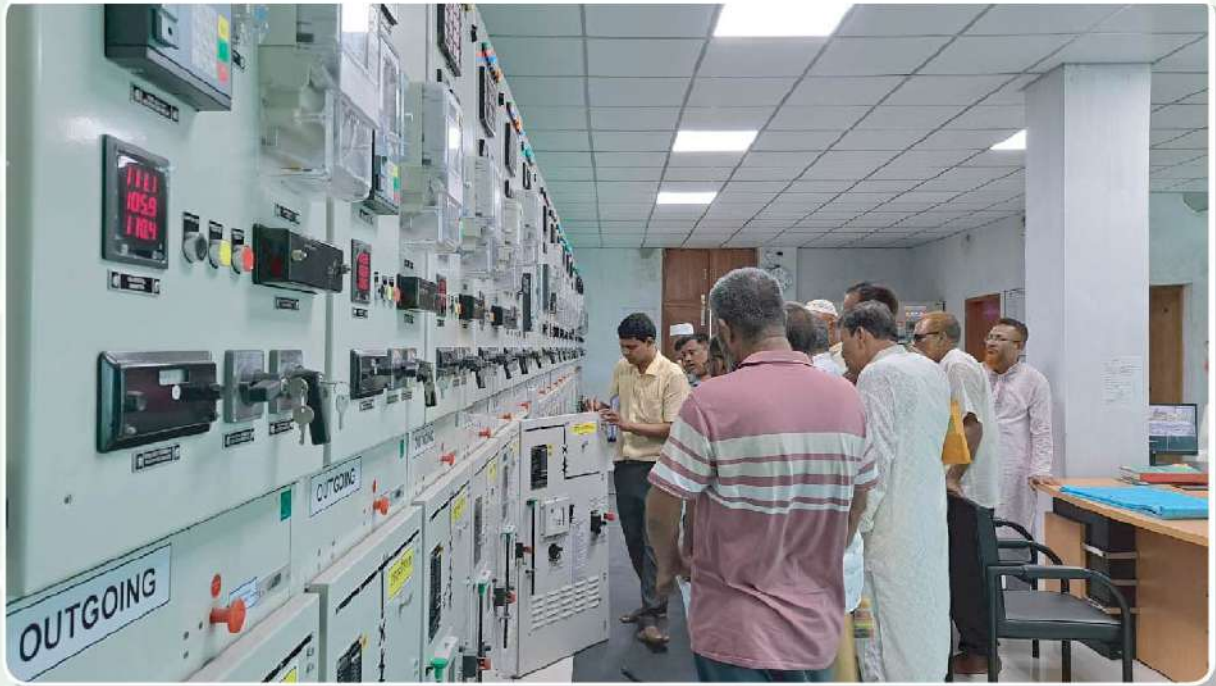
Practical training at Central Sub-Station, Khulna.
