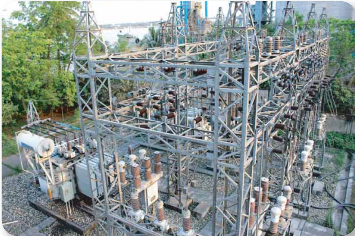
33/11 KV, 2x10/13.33 MVA Labanchara Sabsation
