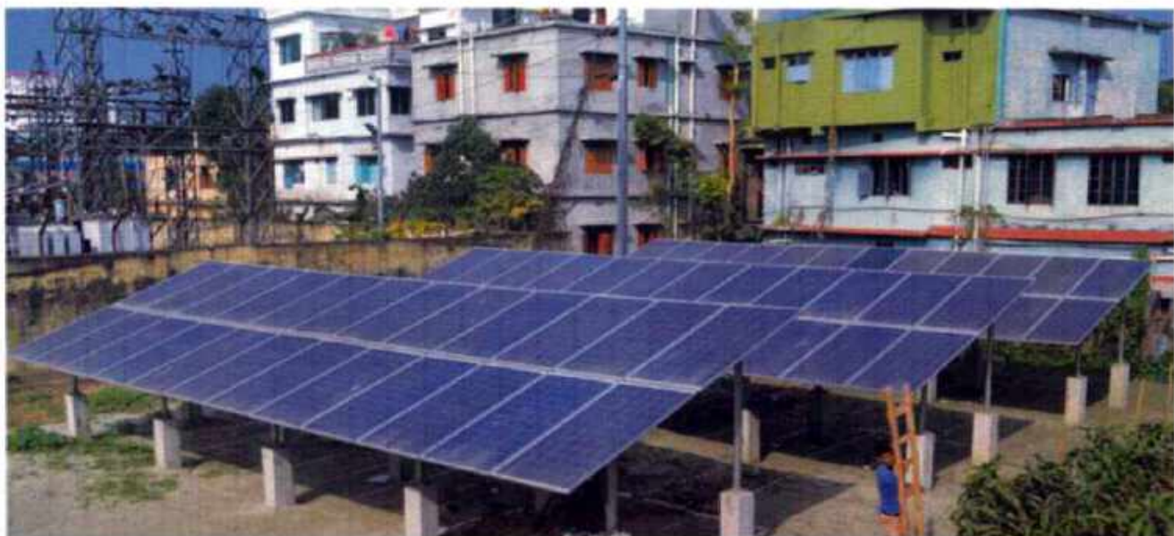
21 kWp Easybike Solar Charging Station, Jashore
