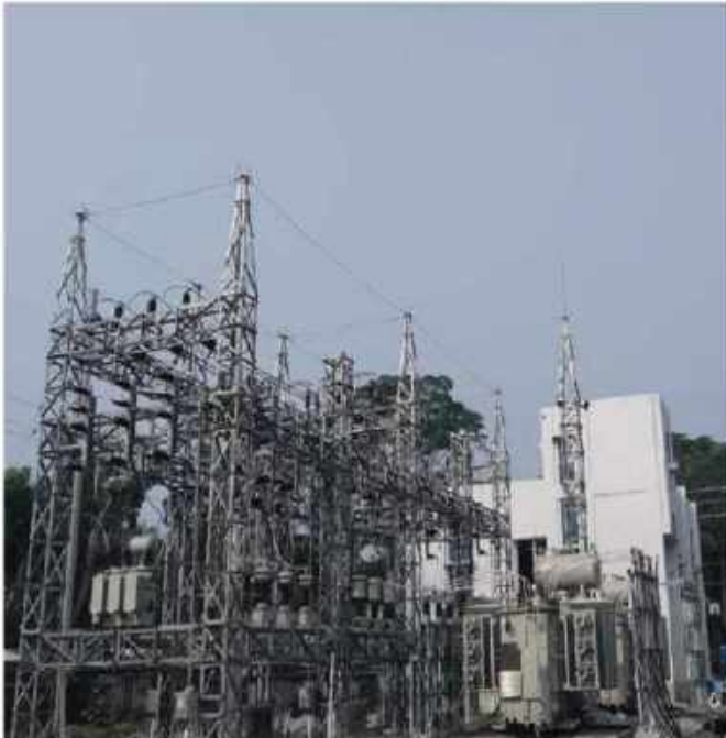
Newly constructed Chadkathi 33/11 kV 2x10/13.33 MVA SS, Jhalokathi
