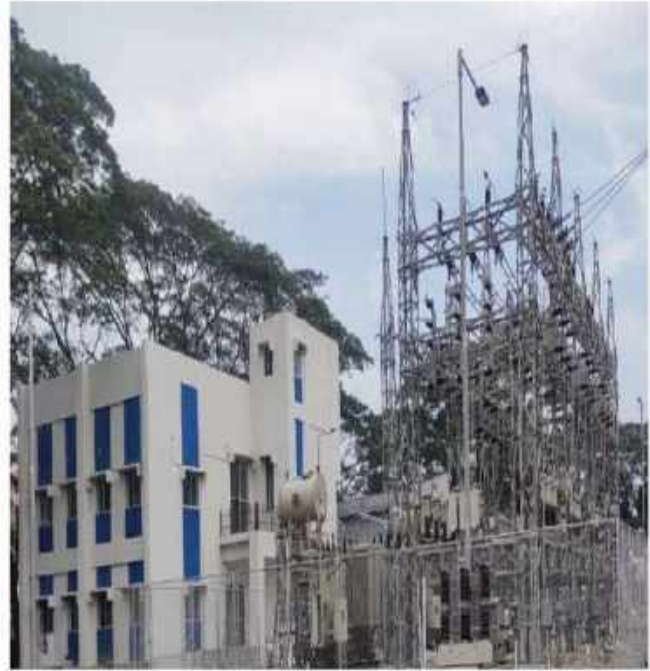
Newly constructed Chadmari 33/11 kV 2x10/13.33 MVA SS, Barishal
