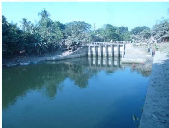
Photograph 4.7: The newly constructed regulator (BWDB design) close to water structure (British design) at the mouth of Kata Khal joining the Kobadak River at Jhikargacha.
