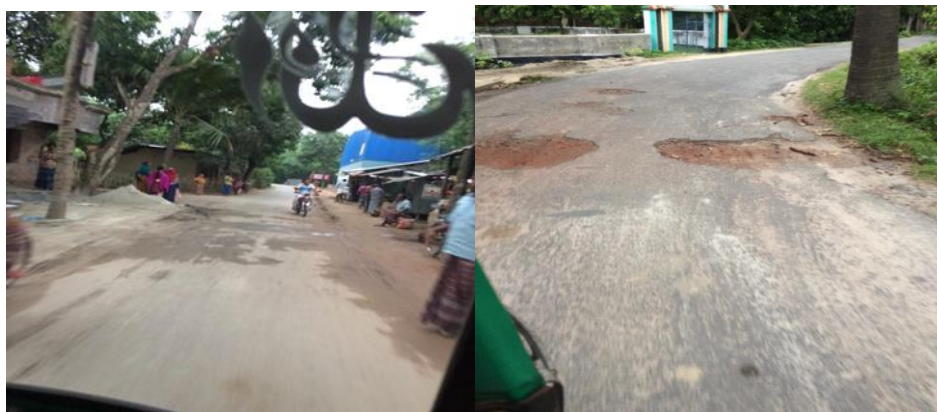
Photo 3-37: Poor Conditions of Roads (Source: Field Visit, 2015)
