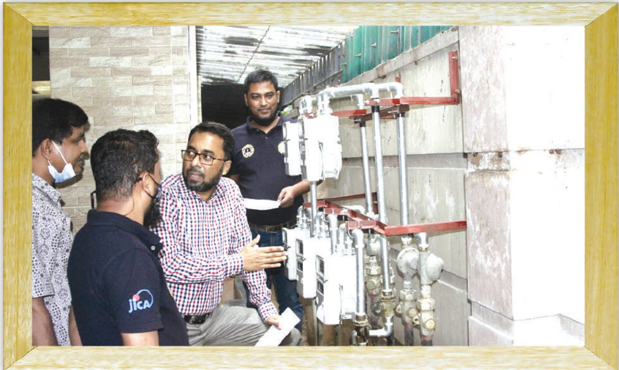
Demonstrating Pre-paid Gas Meter to the Customers
