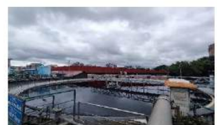
Fig. 13 Secondary clarifier/ Sedimentation
