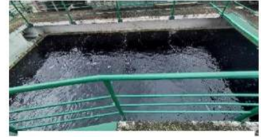
Fig. 27 Post aeration tank
