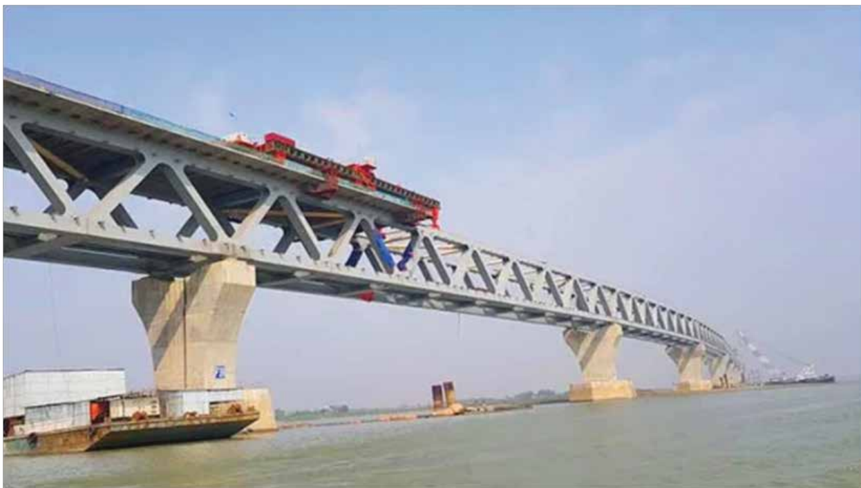
The construction of the Padma Bridge linking southwest Bangladesh to northern and eastern regions and other major projects are contributing to the country's economic growth.
