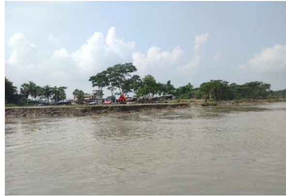
Fig. 2. Present right bank erosion situation of the Tetulia River in the upstream of Dhulia Launch Ghat area.
