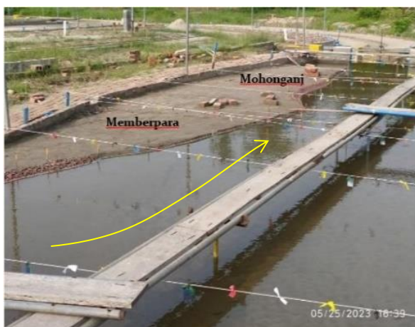
Fig. 7. Placement of existing bank protection works at Memberpara and Mohonganj (T1 2.33yr ).
