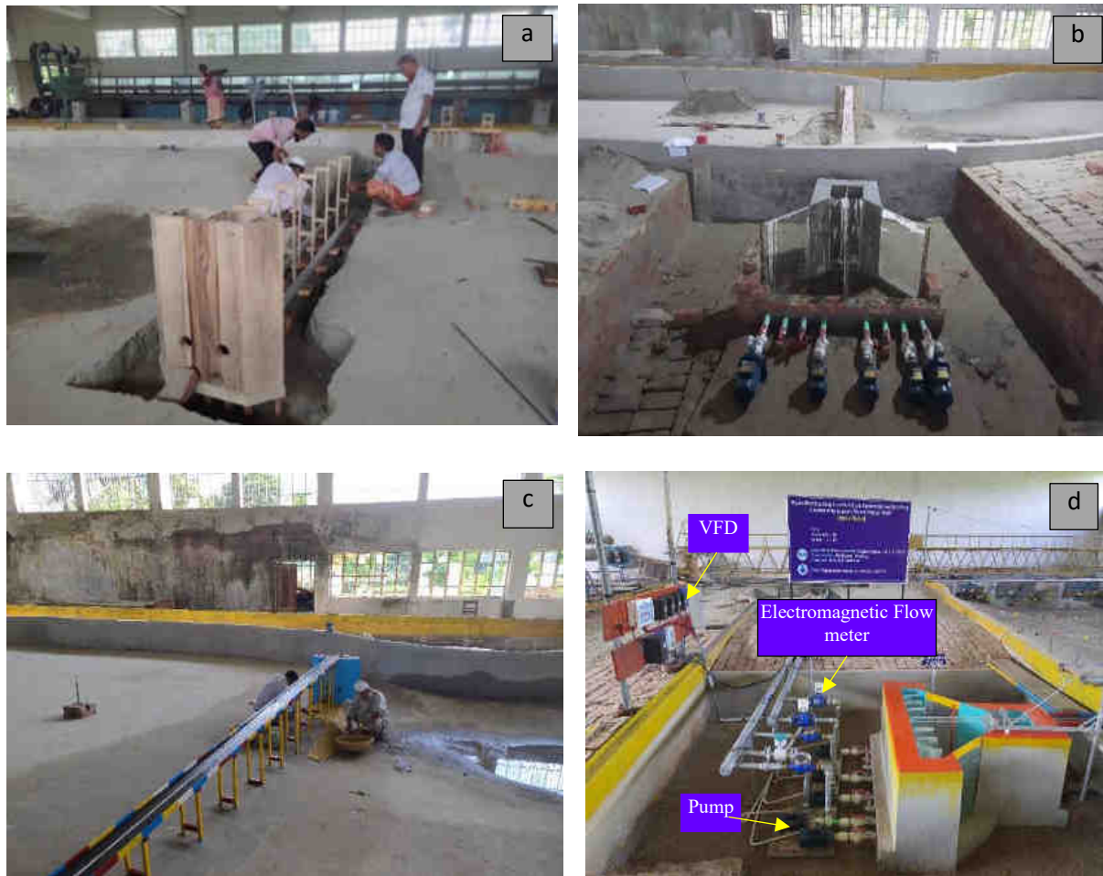
Fig. 6. a) Bedding of Conveyance pipe & Access bridge support column b) Construction of distribution chamber c) Placing of concrete armour unit & CC block and d) Installation of pump, VFD & Electromagnetic Flow meter.
