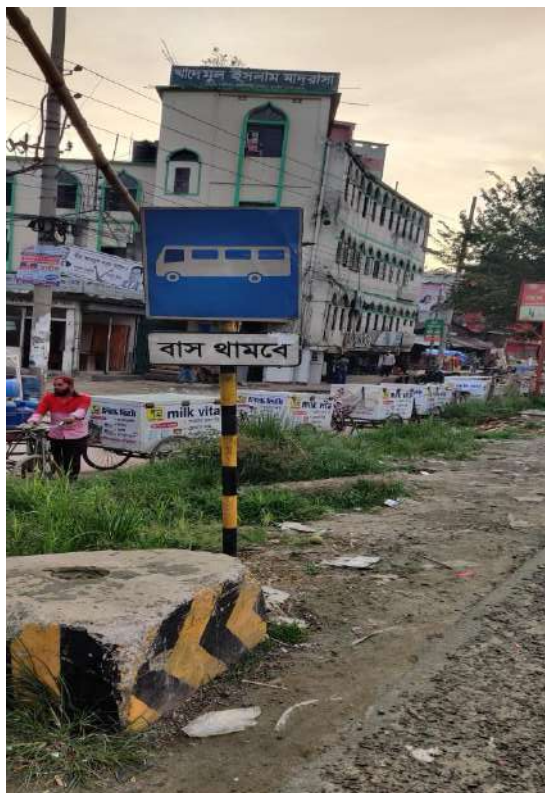
Risky edge structure within Ch.+ 2 to Ch.+4
