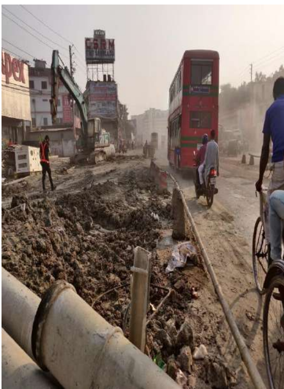
Side road activity without proper marking at Airport to Jaydevpur Under-construction zone
