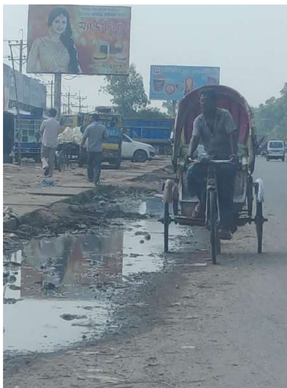
waterlogged shoulder within Ch.+ 74 to Ch.+78
