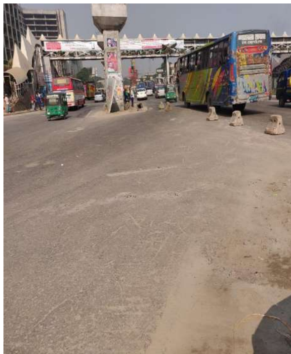
Risky column and boulders without safety barrier at Airport to Jaydevpur Under-construction zone
