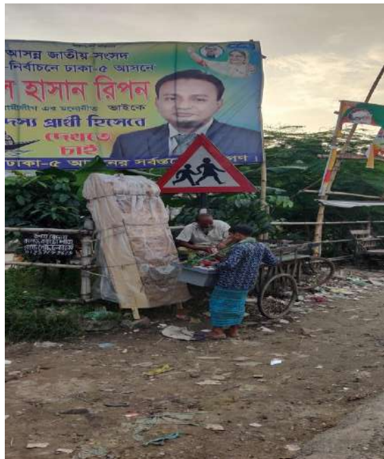
Disturbed Shoulder and sign within Ch.+ 2 to Ch.+4
