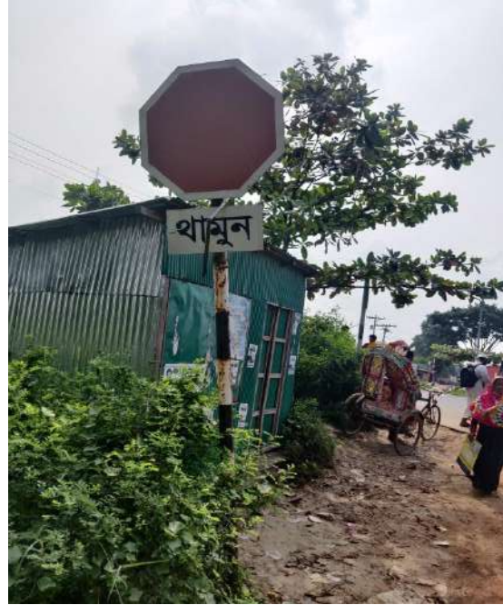
Disturbed Shoulder and sign within Ch.+53 to Ch.+54
