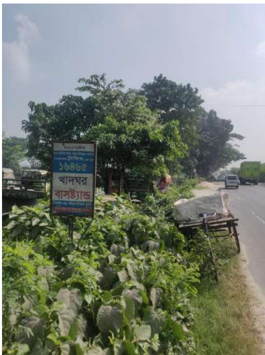
Poor visibility of road signs within Ch.+59 to Ch.+60
