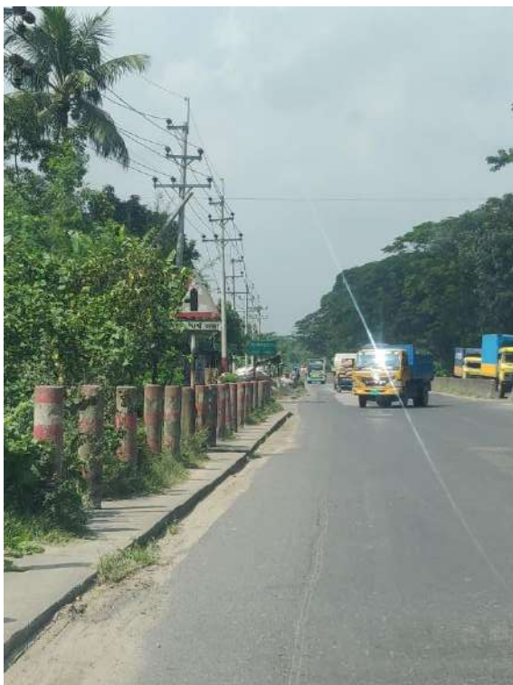
Risky shoulder edge at Ch.+103 to Ch.+106
