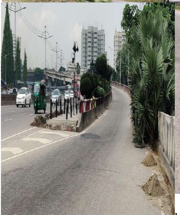
Abrupt ending of sidewalk at a very risky zone in front of Radisson
