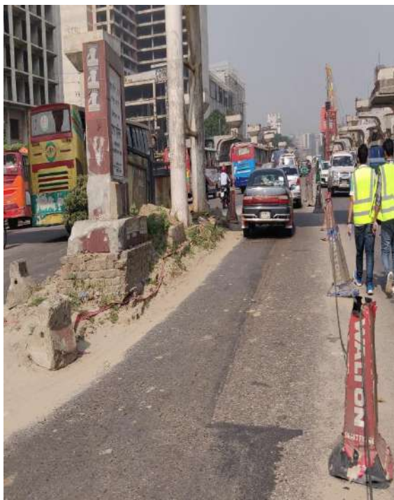
Risky broken median in Airport to Jaydevpur Under-construction zone
