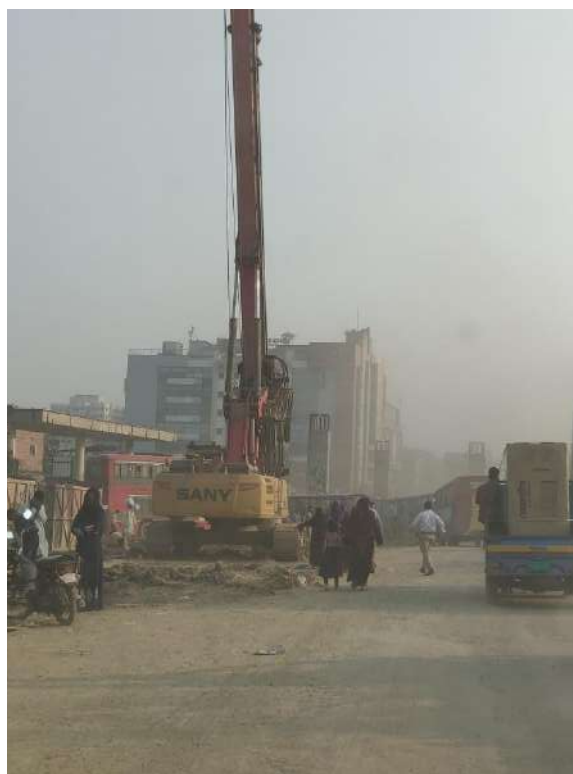
Construction equipment without safety provision at Airport to Jaydevpur Under-construction zone
