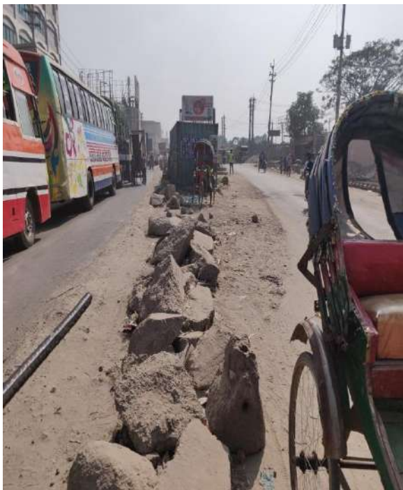
Broken Boulders used as median at Airport to Jaydevpur Under-construction zone
