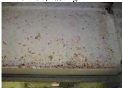
Photo18-1 Surface area of 10~20% rusting
