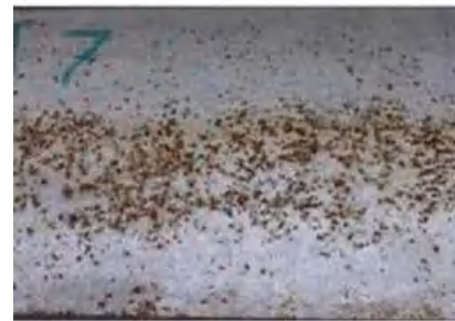
Photo4-2 Surface area of 20~30 rusting
