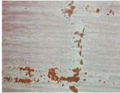
Photo18-3 Less severe corrosion
