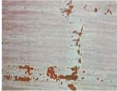
Photo4-3 Less severe corrosion
