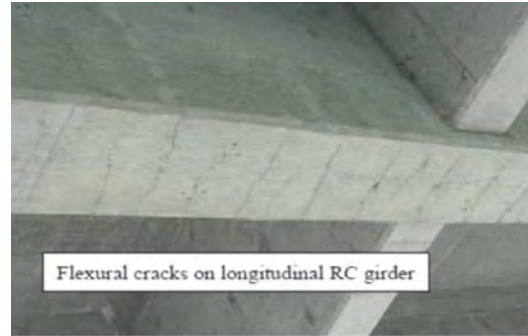
Photo 10-2 Example of Flexural Crack
