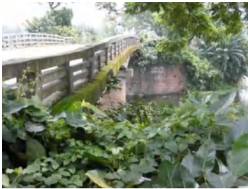
Fig.2-17 Harmful weed around the bridge
