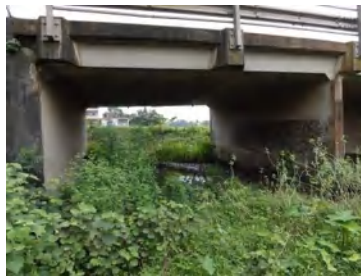
Fig. 2-18 Harmful weed under the bridge
