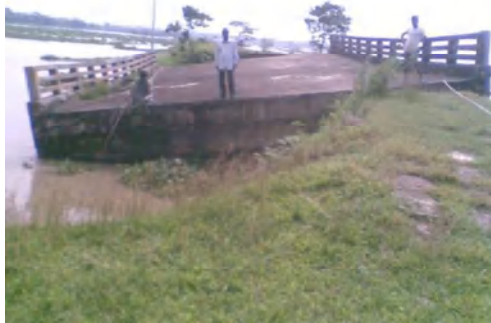
Photo 3-14-1 typical Bridge scour
