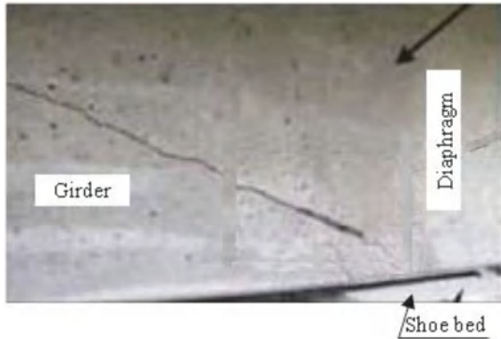
Photo 9-1 Example of Shear Crack
