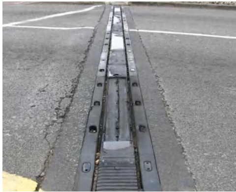
Figure 4-7 damaged Expansion Joint
