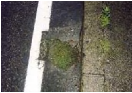
Fig.2-3 Blocked catch basin at surface
