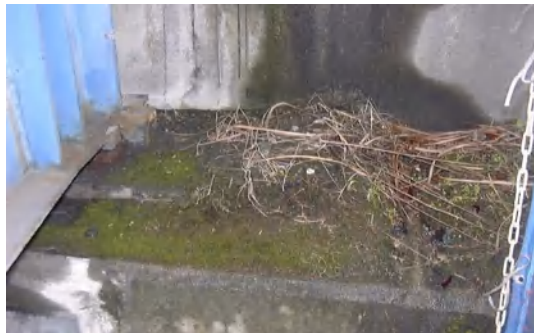
Fig.2-10 Bearing with Debris
