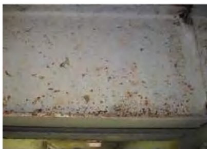
Photo4-1 Surface area of 10~20% rusting
