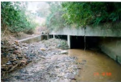
Fig. 2-16 Culvert with flow obstruction
