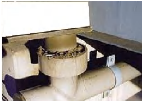
Fig.2-5 Blocked drain pipe with bird's dung
