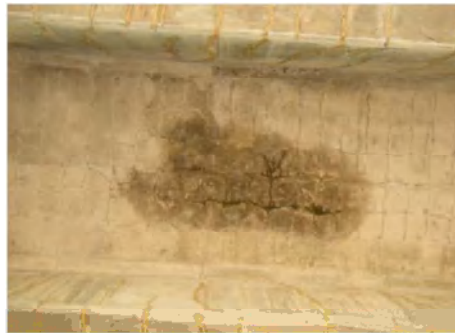
Damaged Deck Slab with water leakage
