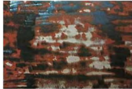
Photo18-4 More severe corrosion
