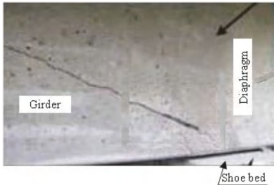
Photo 10-1 Example of Shear Crack
