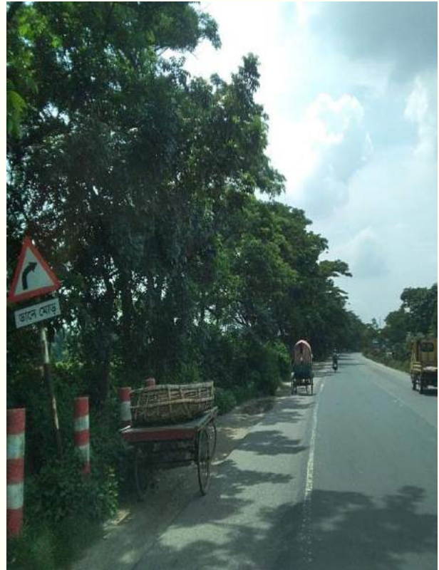
Disturbed sign within Ch.+15 to Ch.+17
