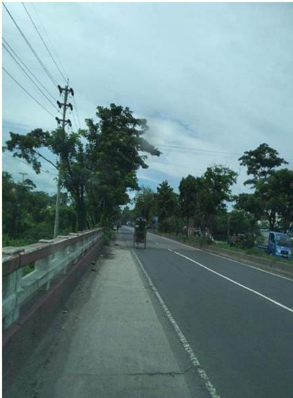
Unprotected pedestrian facility on bridge within Ch.+29 to Ch.+31
