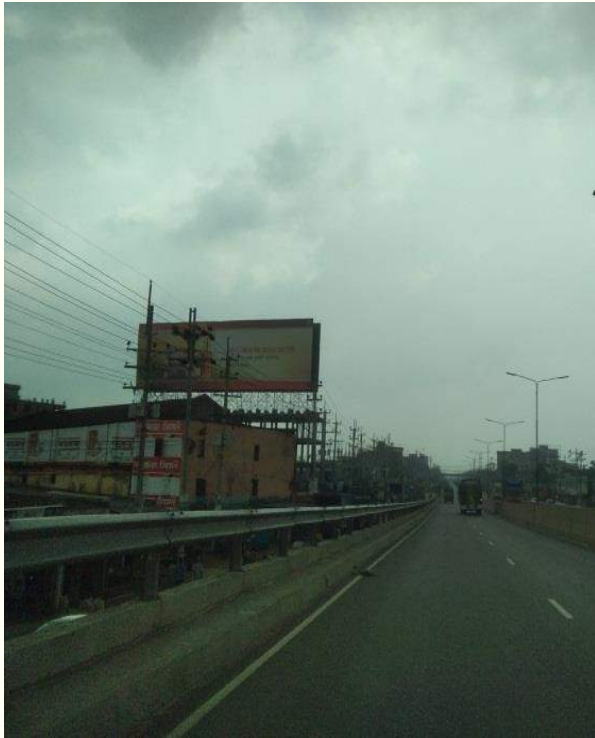
Wrong placement of guard rail within Ch.+47.8 to Ch.+49.8
