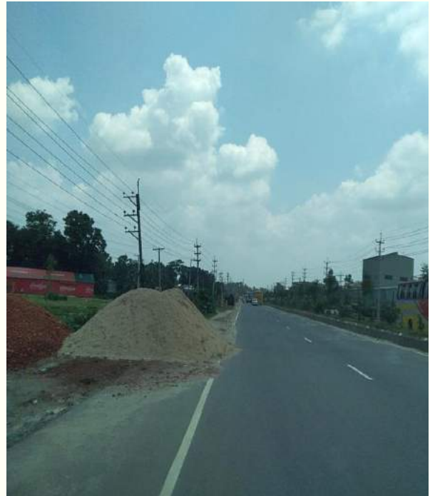
Unauthorized occupancy by construction materials within Ch.+67.5 to Ch.+69.5
