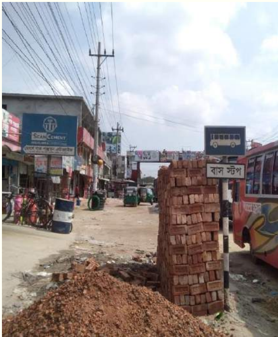
Construction materials kept on roadside area illegally within Ch.+89.5 to Ch.+91.5
