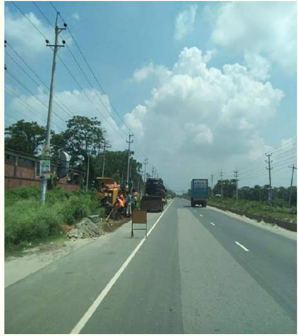
Road construction work along roadside area within Ch.+63.6 to Ch.+65.6 causing high risk
