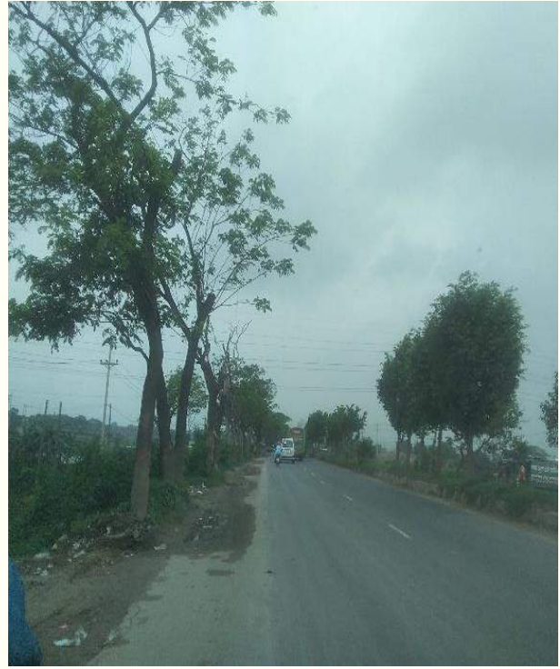
Earthen shoulder within Ch.+2 to Ch.+4 is at risk due to roadside tree
