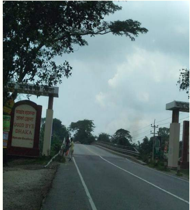
Risky structure at earthen shoulder within Ch.+42 to Ch.+44
