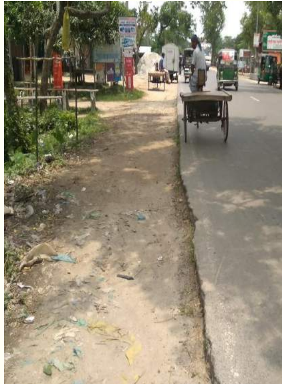
Risky shoulder drop within Ch.+26 to Ch.+28
