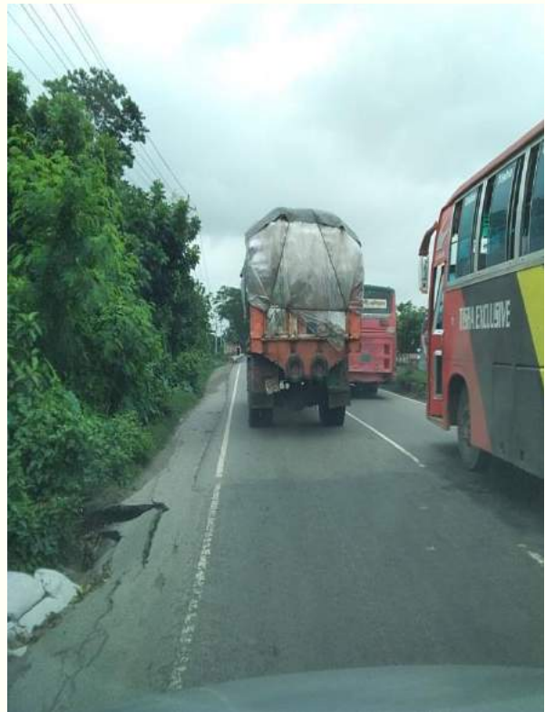
Risky edge drop within Ch.+31 to Ch.+33
