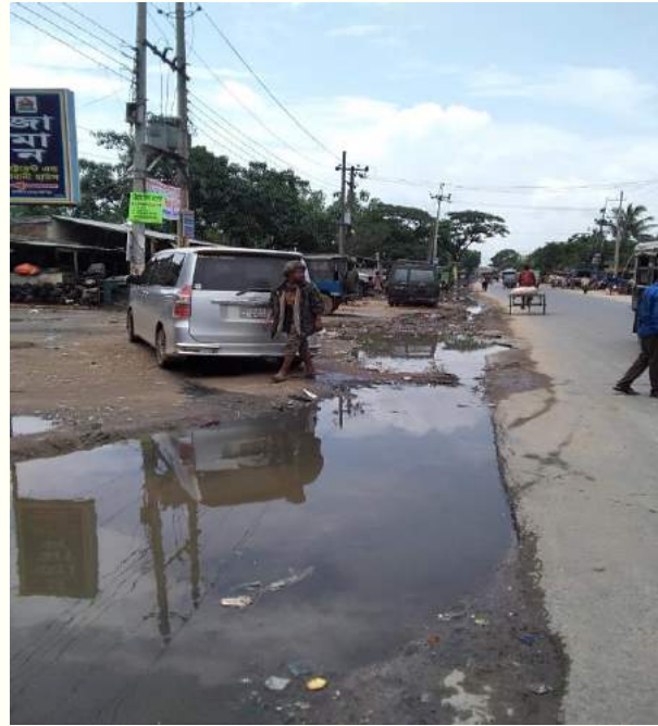
Water logging at Ch.+ 331 to Ch.+333
