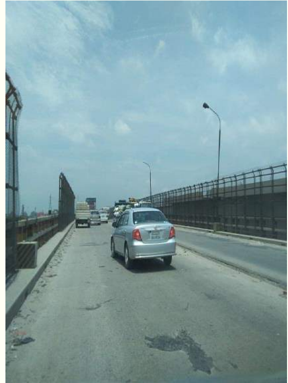
Blocks causing risk for pedestrian movement within Ch.+7 to Ch.+9
