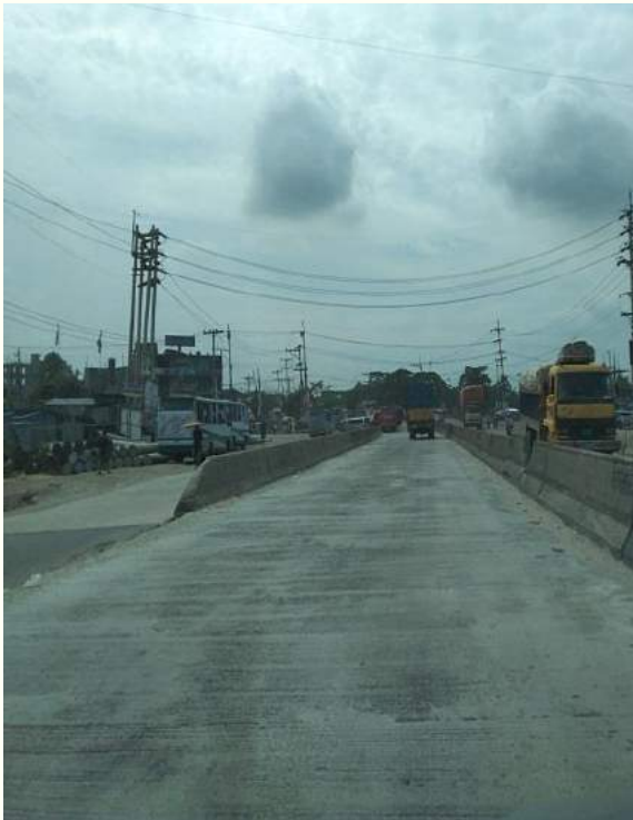
Median without proper protection within Ch.+11 to Ch.+13
