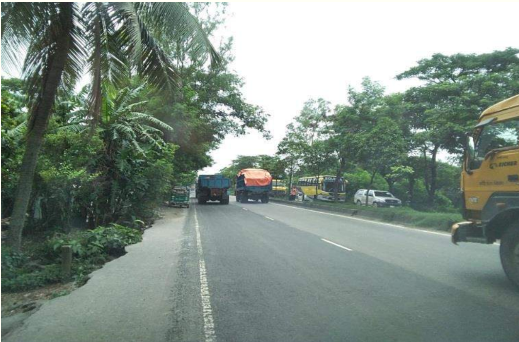
Risky edge drop within Ch.+35 to Ch.+37
