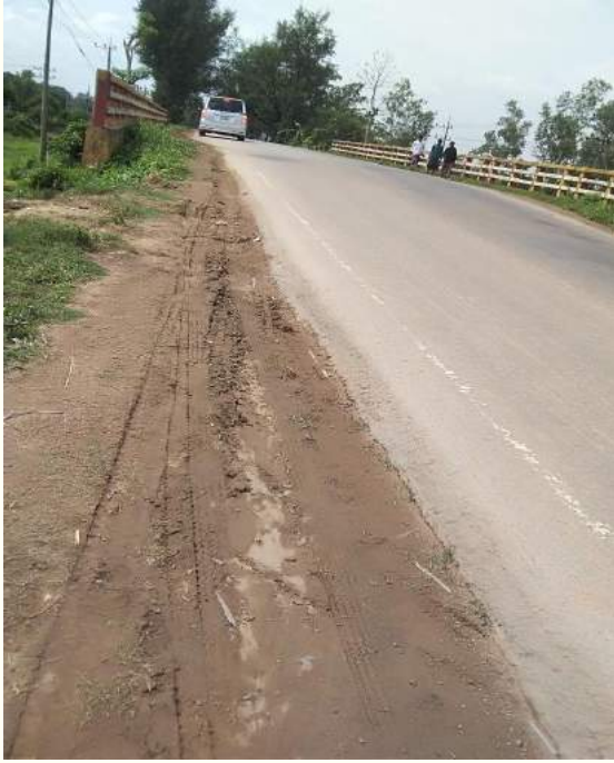
No warning sign and marking across the bridge within.Ch.+287 to Ch.+289
