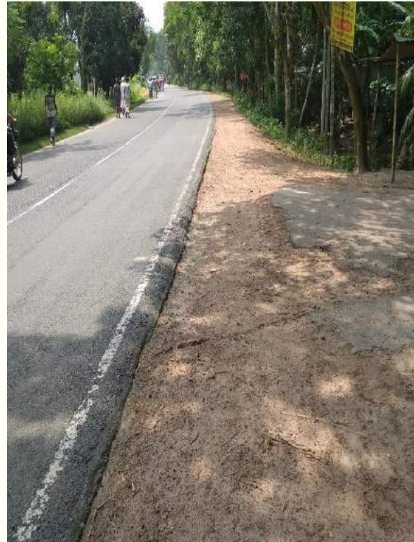
Lack of shoulder forcing pedestrian to walk on carriageway within Ch.+18 to Ch.+20
