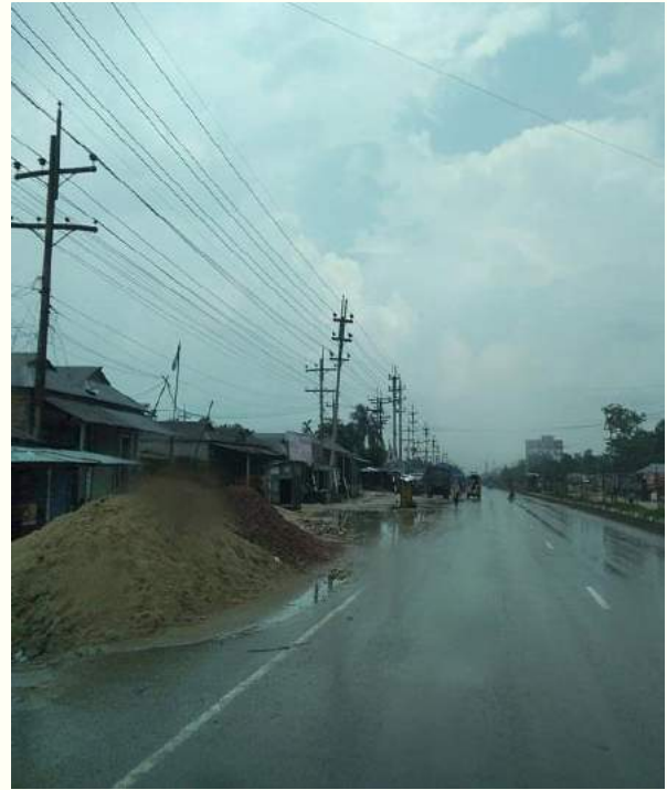
Construction materials kept on roadside area illegally within Ch.+51.6 to Ch.+53.6
