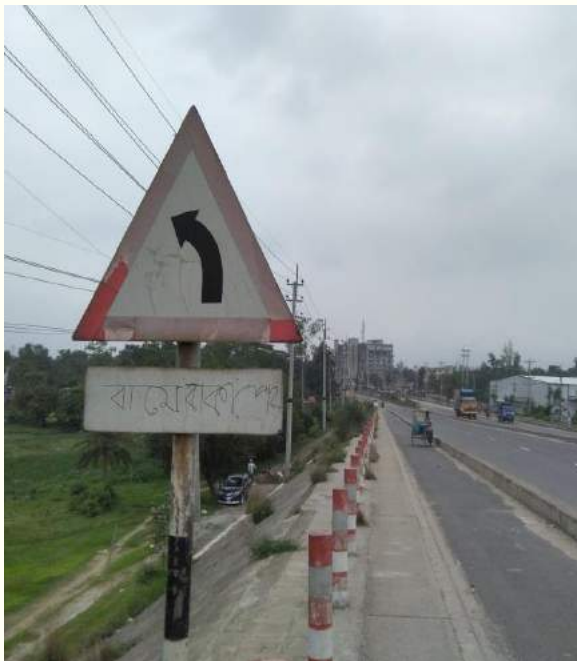
Faded and non-reflective sign within Ch.+25.8 to Ch.+27.8
