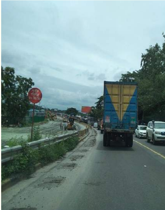
Wrongly designed sign within Ch.+23 to Ch.+25
