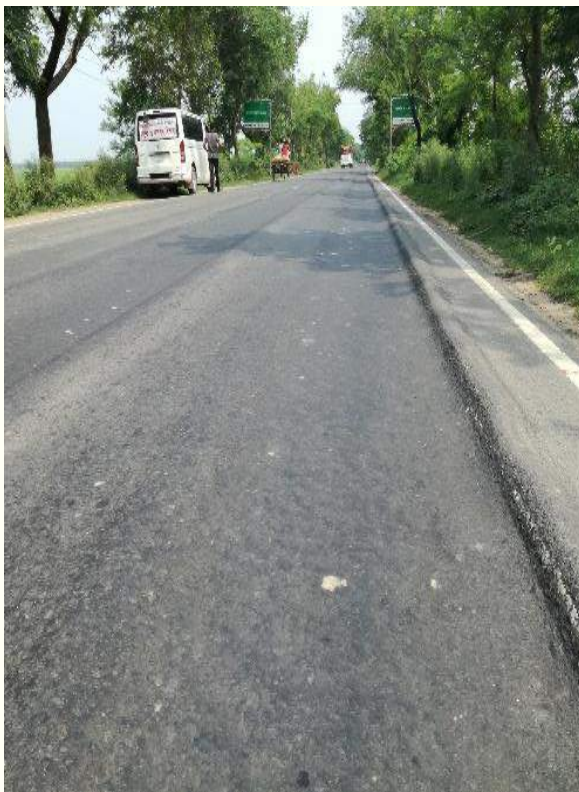
Distressed pavement within Ch.+74 to Ch.+76
