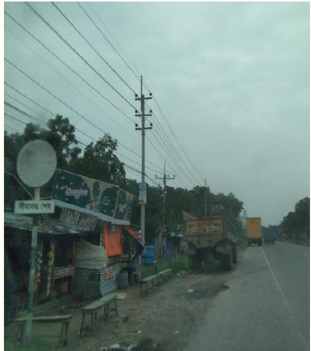
Faded sign and illegal parking within Ch.+35.8 to Ch.+37.8
