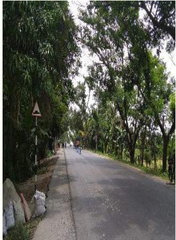
Wrong dimension of road sign within Ch.+130 to Ch.+132
