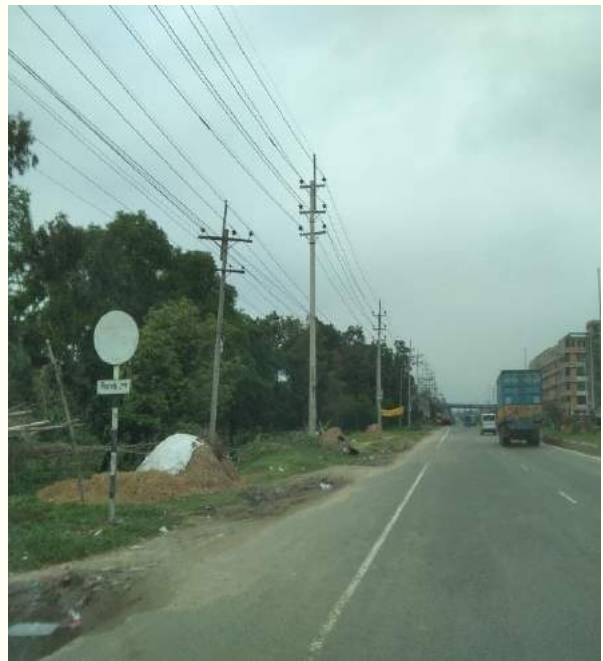
Faded road sign and marking within Ch.+25.8 to Ch.+27.8
