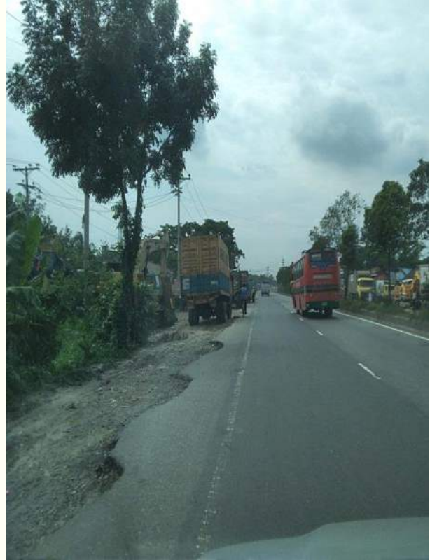
Poor and risky shoulder drop within Ch.+11 to Ch.+13
