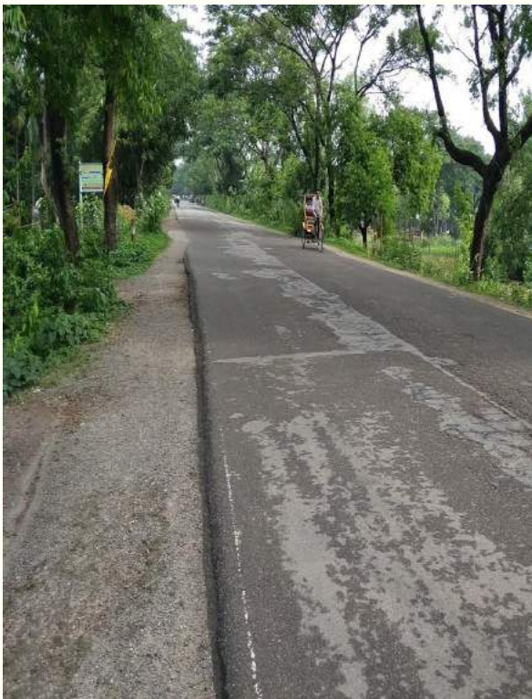
Shoulder within Ch.+46 to Ch.+48 at a risky condition
