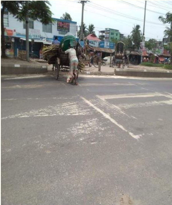
Faded pedestrian crossing within Ch.+21.8 to Ch.+23.8
