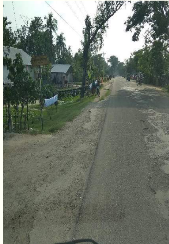
Poor pavement and shoulder within Ch.+36 to Ch.+38
