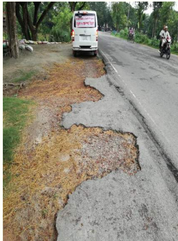
Defective shoulder at Ch.+48 to Ch.+50
