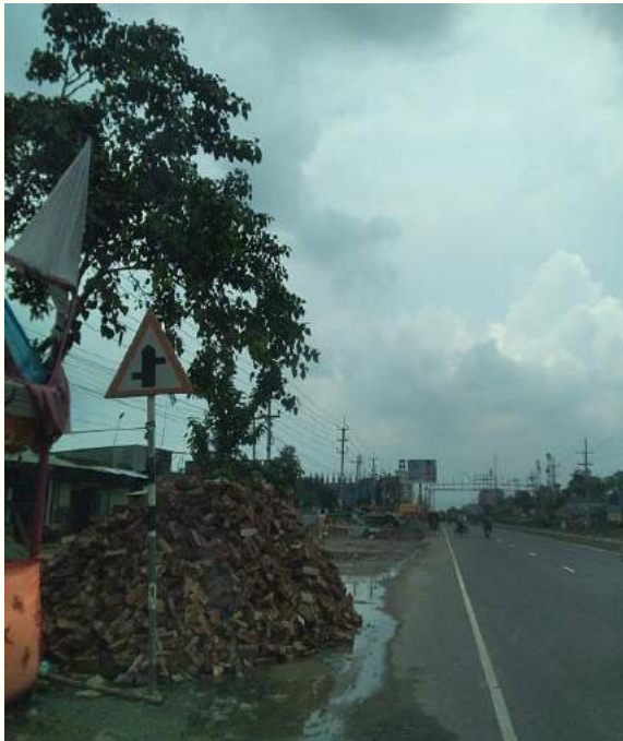
Construction materials kept on roadside area illegally within Ch.+59.6 to Ch.+61.6
