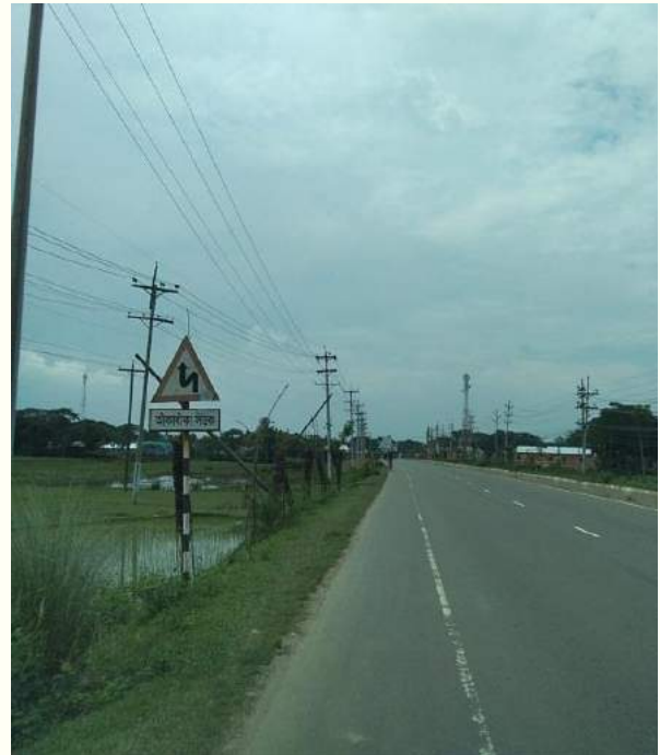
Faded road marking within Ch.+83.5 to Ch.+85.5
