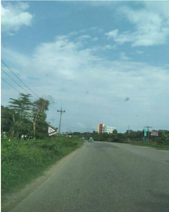
Defective road sign at Ch.+269 to Ch.+271
