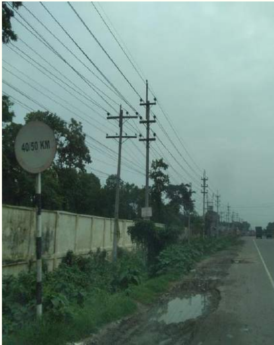
Risky edge drop and faded road sign within Ch.+35.8 to Ch.+37.8
