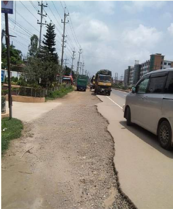
Broken hard shoulder within Ch.+65.6 to Ch.+67.5
