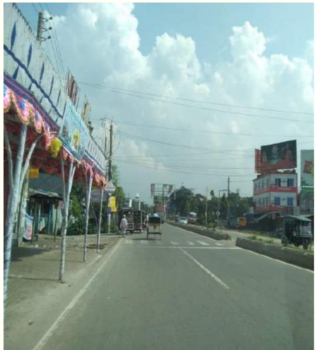
Illegal structure & faded road marking at Ch.+105.5 to Ch.+107.5
