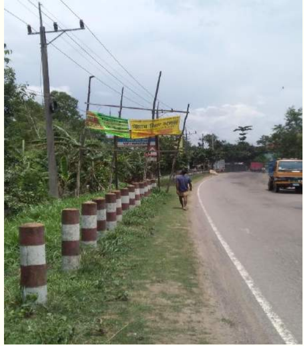
Inadequate shoulder within Ch.+293 to Ch.+295
