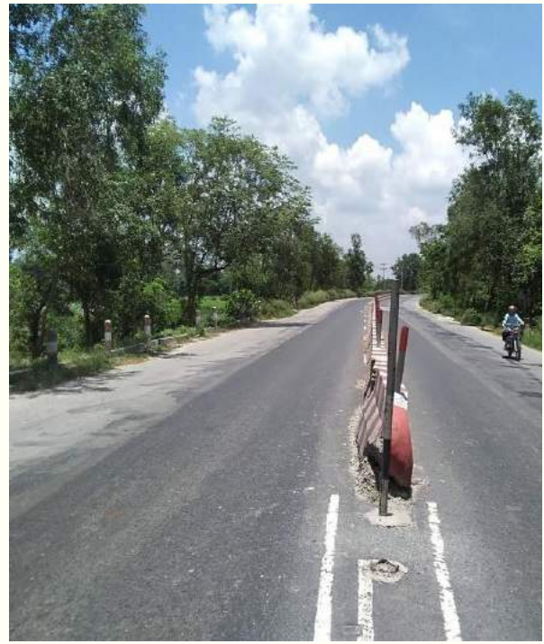
Disturbed warning sign within Ch.+66 to Ch.+68
