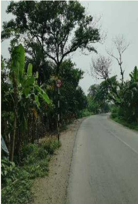
Wrong dimension of road sign within Ch.+124 to Ch.+126
