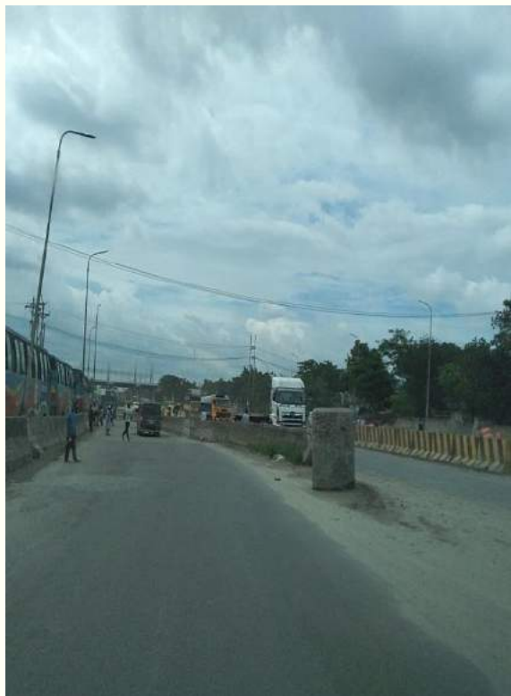
Hazardous concrete block within Ch.+23 to Ch.+25
