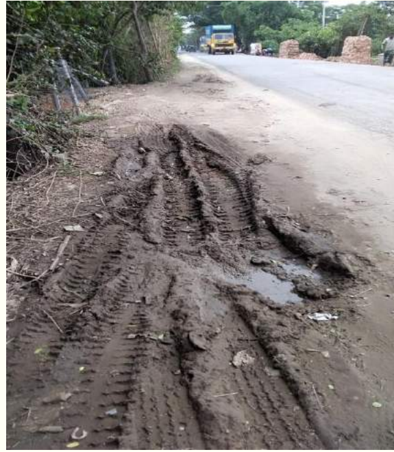
Defective shoulder due to rain within Ch.+252.5 to Ch.+255
