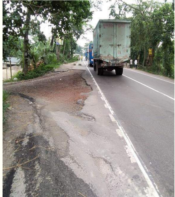
Defective roadside area within Ch.+42 to Ch.+44
