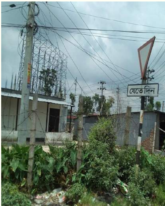
Disturbed sign within Ch.+103.5 to Ch.+105.5
