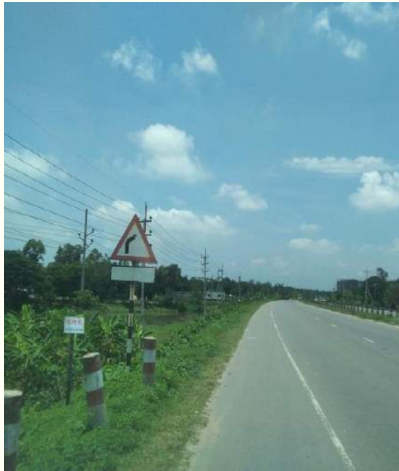
Faded sign and name plate within Ch.+81.5 to Ch.+83.5
