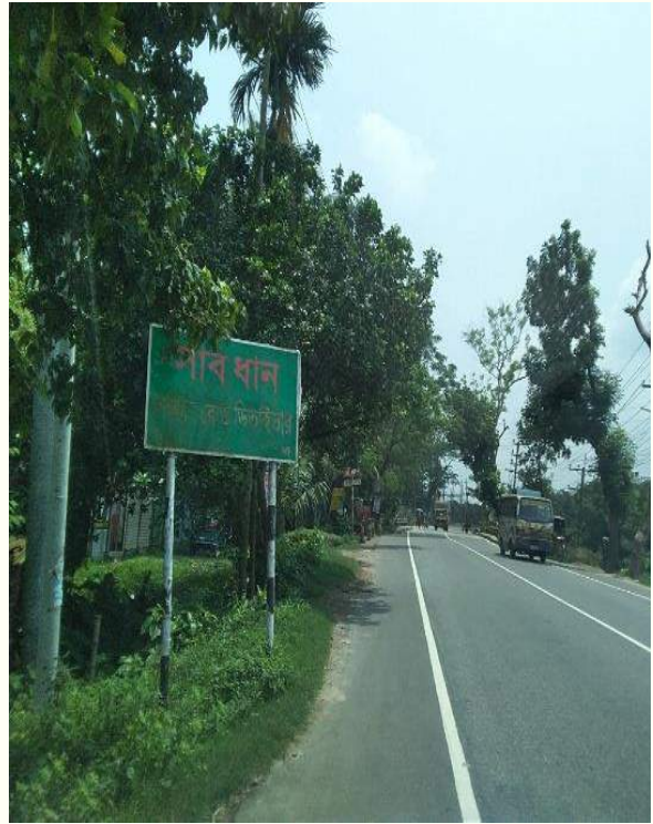
Risky sign post on shoulder within Ch.+48 to Ch.+50
