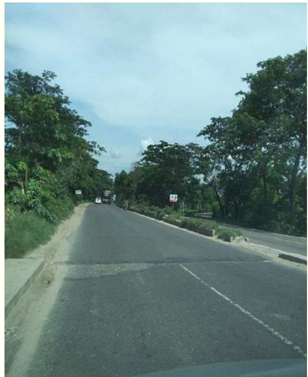
Poor and broken median within Ch.+15 to Ch.+17
