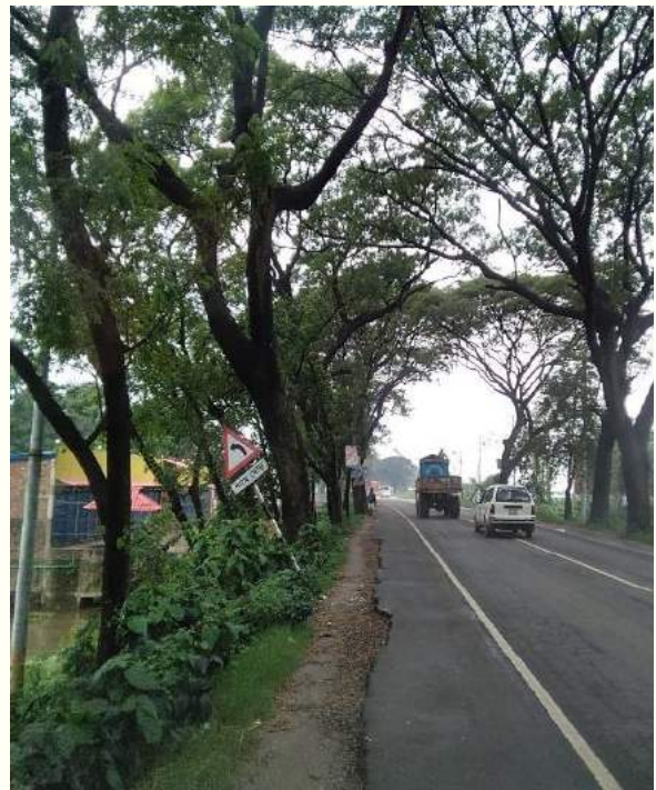
Risky edge drop within Ch.+30 to Ch.+32
