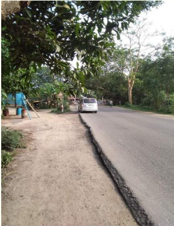
Risky shoulder drop at Ch.+299 to Ch.+301
