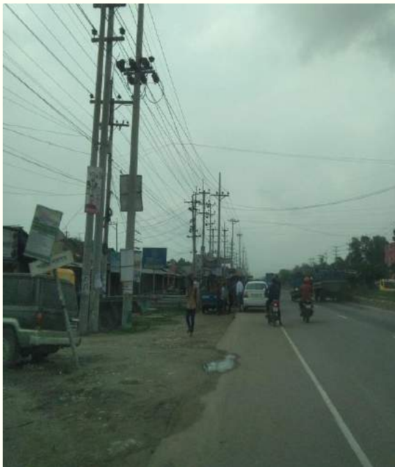
Disturbed road sign within Ch.+43.8 to Ch.+45.8
