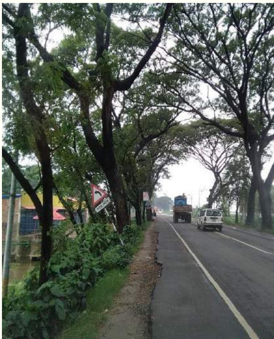
Risky shoulder drop within Ch.+46 to Ch.+48
