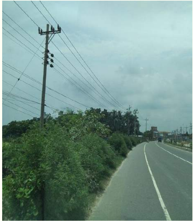
Roadside bushes & wrong marking on curve within Ch+103.5 to Ch+105.5
