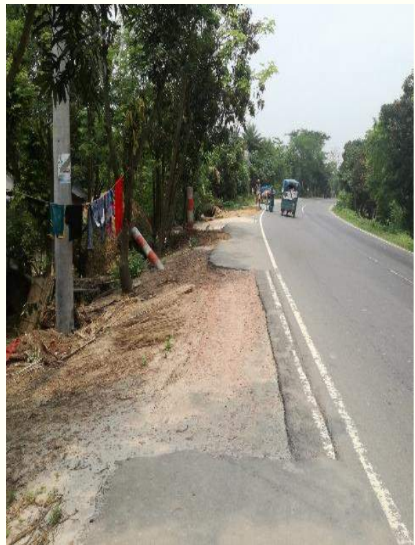
Defective and risky shoulder at Ch.+ 84 to Ch.+86
