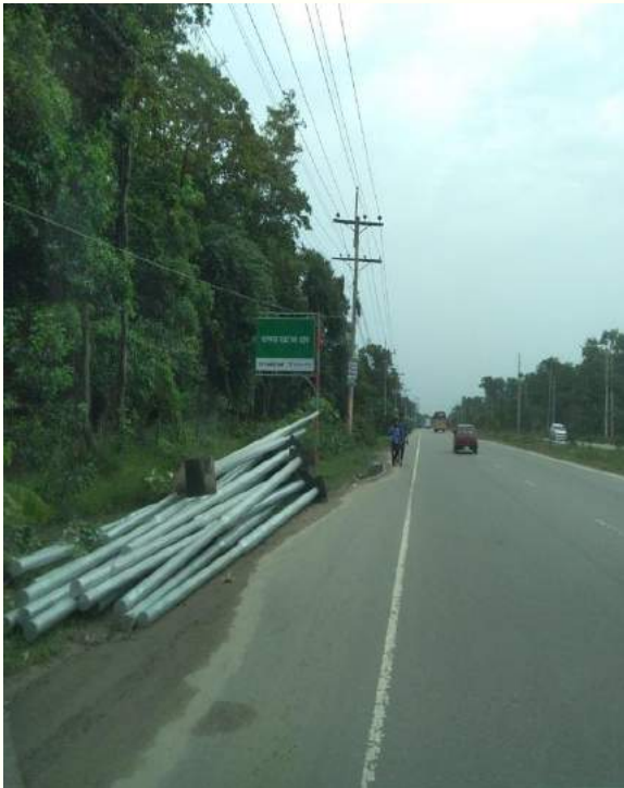
Unauthorized roadside occupancy within Ch.+29.8 to Ch.+31.8
