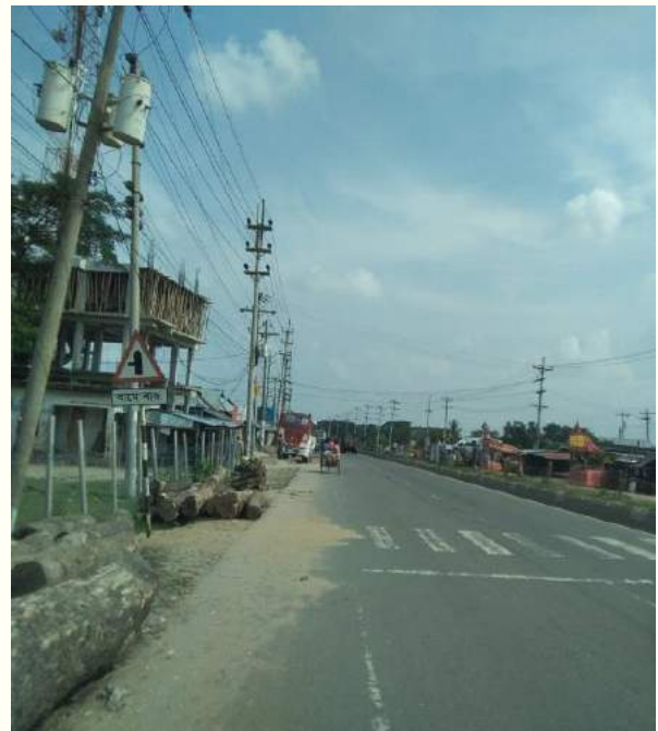
Faded road marking & unauthorized occupancy within Ch.+85.5 to Ch.+87.5
