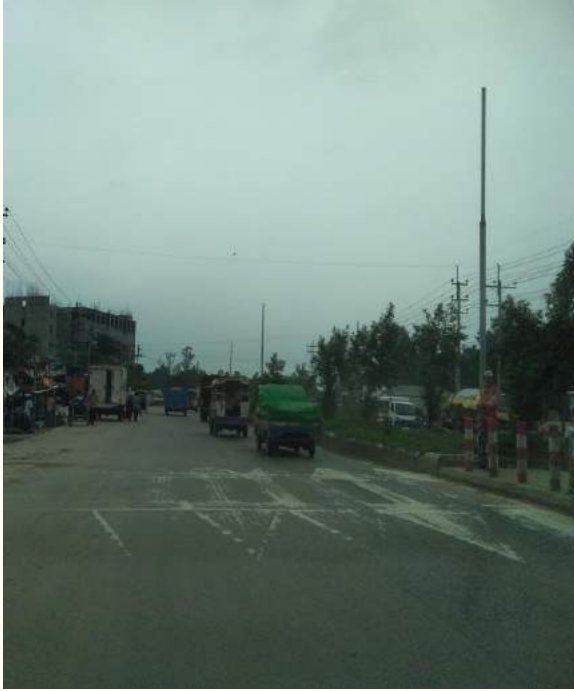
Faded zebra crossing within Ch.+27.8 to Ch.+29.8
