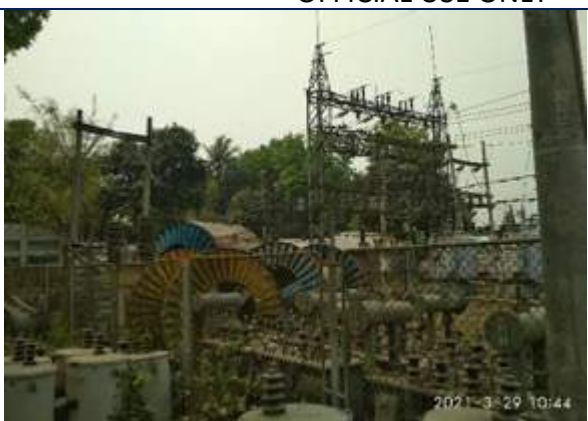
Substation Compound , Rangpur PBS-2
