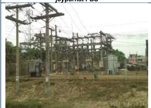
substation site at jagarnnathpur, Thakurgaon PBS
