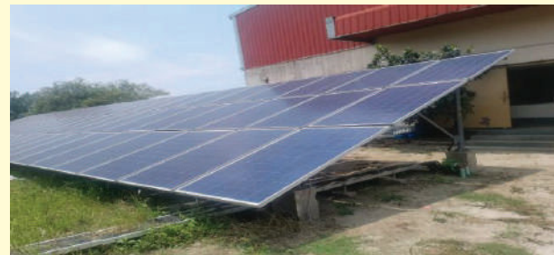
Figure:2 : 10 kWp rooftop solar plant with Net metering at Narayanganj PBS-2
