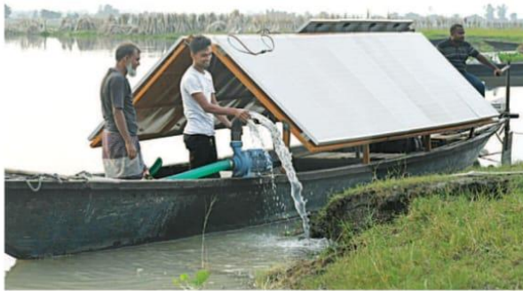
A solar-powered pump set up on a boat to act as a mobile irrigation facility for croplands in chars. The 5-kilowatt pump can irrigate 40-50 bighas of land and costs Tk 2.5 lakhs to set up. The facility came about under a one-year research project being jointly implemented by Rural Development Academy Bogura, Chars Development Research Centre and United Commercial Bank. The photo was taken at Noapara Char of Bogura's Shariakandi upazila on Wednesday.
