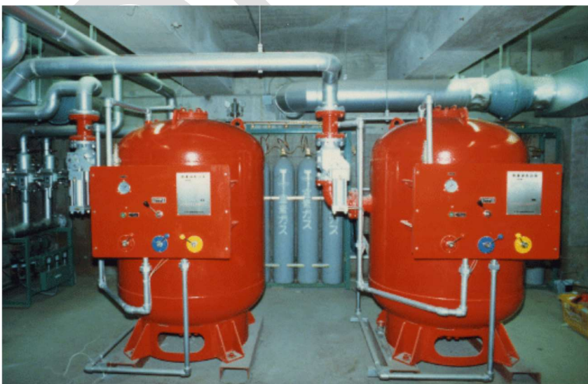
Figure-III-16 Dry powder extinguish system [Source: Yamato Protec]
