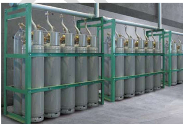
Figure-III-9 Example of Gaseous storage [Source: Yamato Protec]
