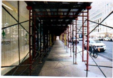
Safety canopy above walkway
