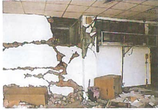
Shear failure of a short column with brick walls The source: Report on the Damage Investigation of the 1999 Chi-Chi Earthquake (Architectural Institute of Japan)
