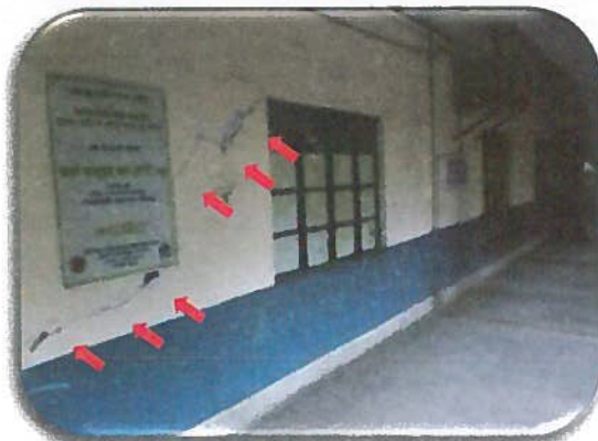
Diagonal crack in brick wall due to differential settlement
