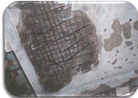
Spalling of slab concrete due to fire disaster
