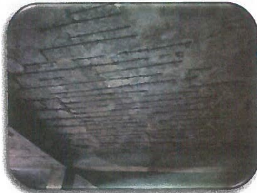
Corrosion of reinforcing bars in slab
