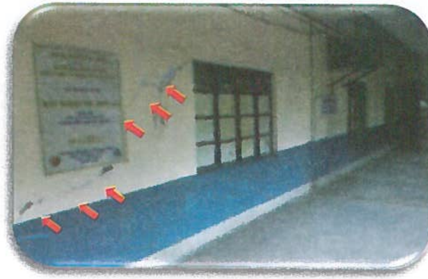
Figure 2.4.3 Inspection of Differential Settlement
