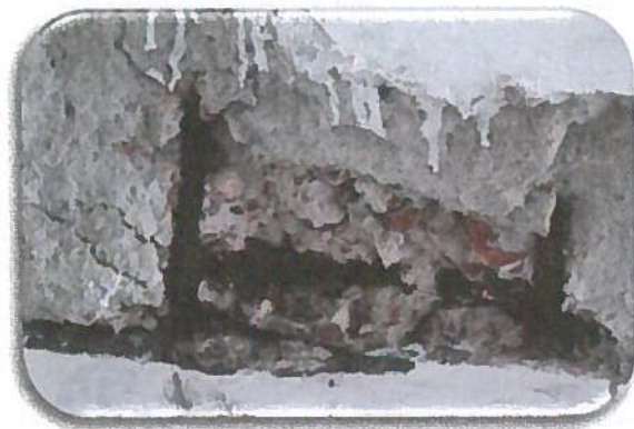
Corrosion of reinforcing bars in beam
