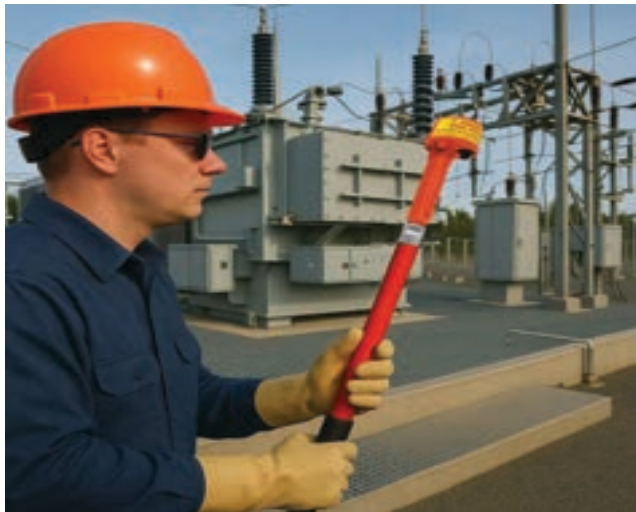
Usage of Live Line/ Voltage Detector
