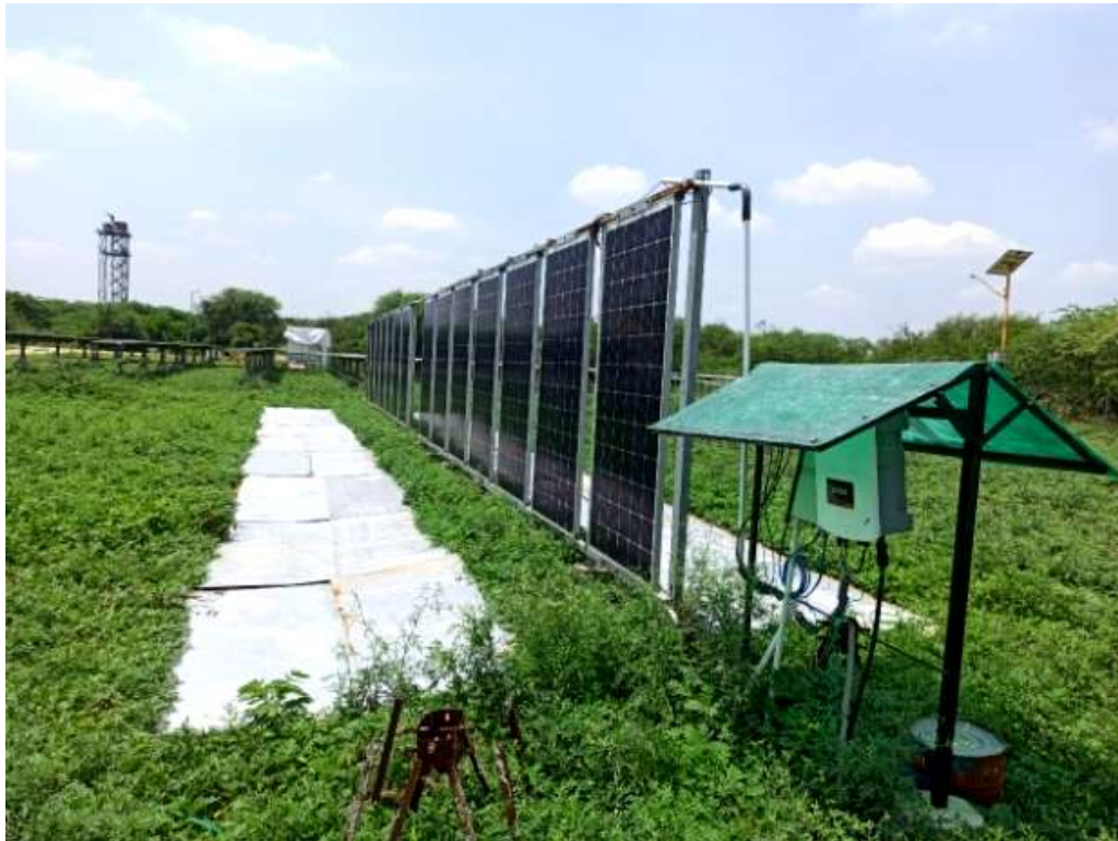
Figure10-3: Vertical solar panels at NISE
