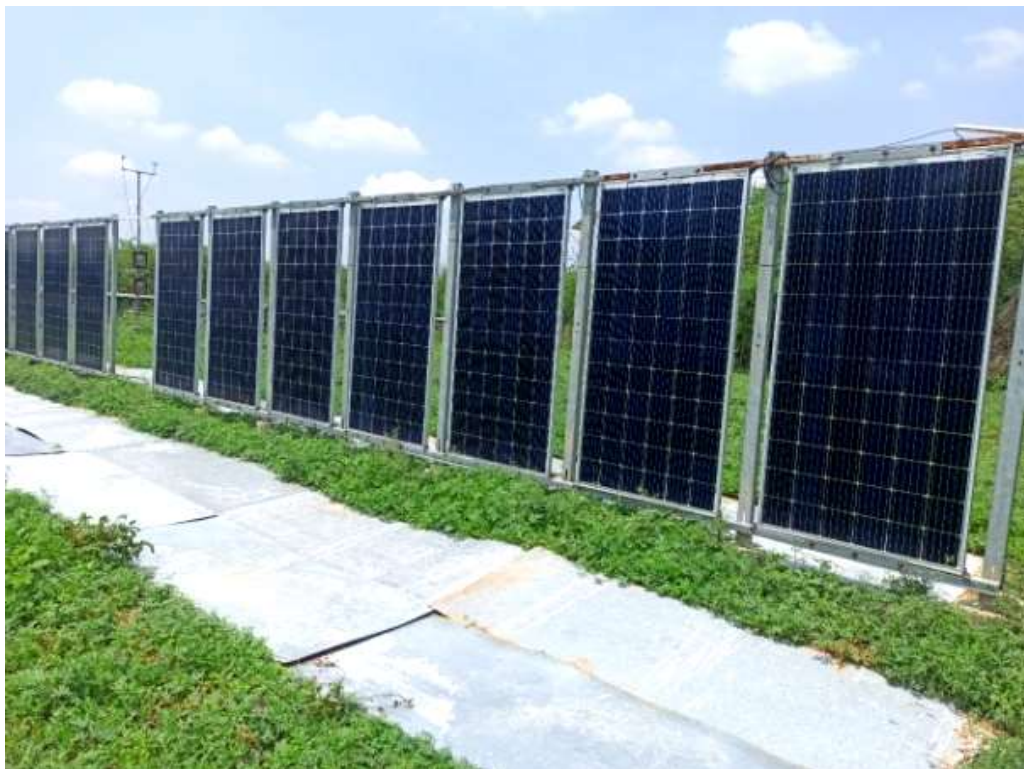
Figure10-4: Another view of vertical solar panels at NISE
