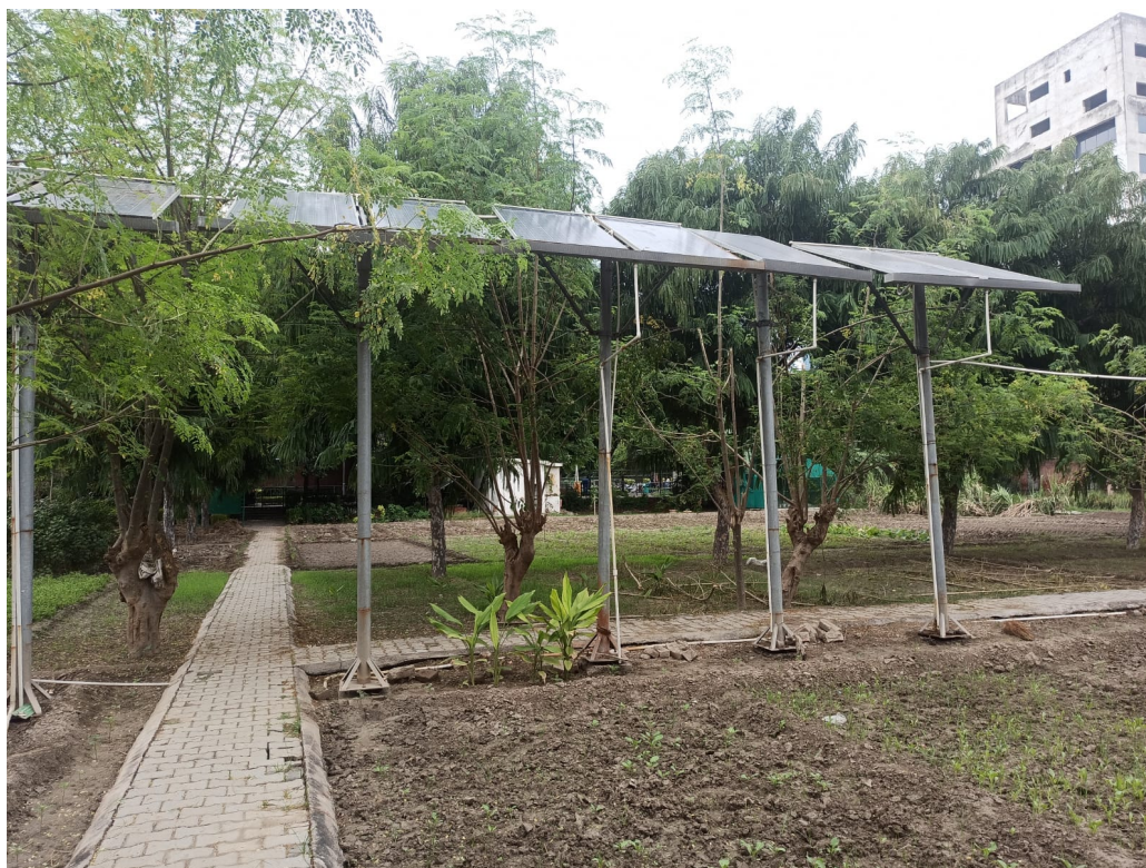
Figure 10-10: Another view of solar panels at Amity
