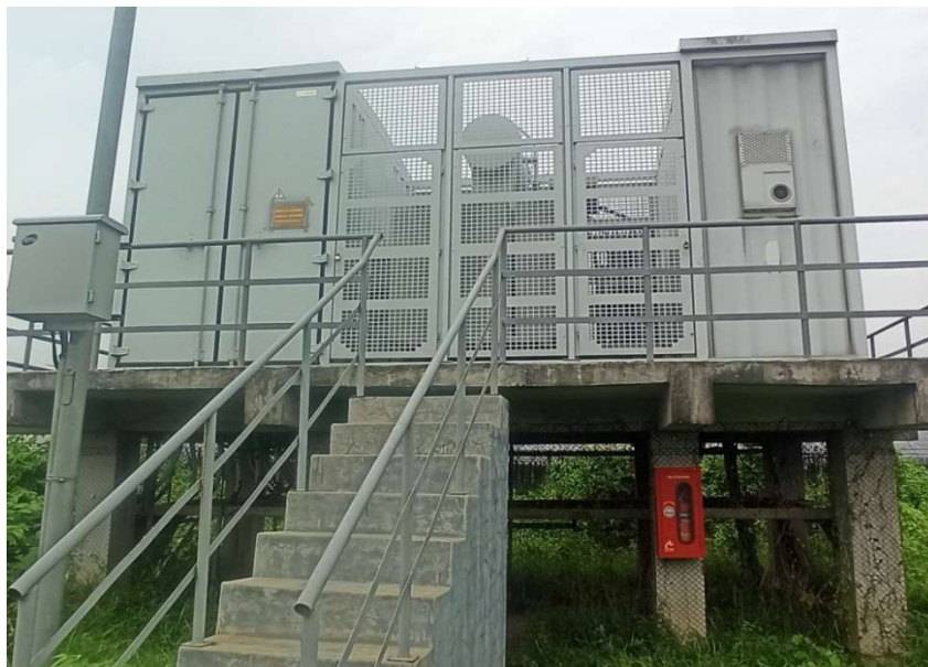
Figure9-4: Transformer on raised platform.
