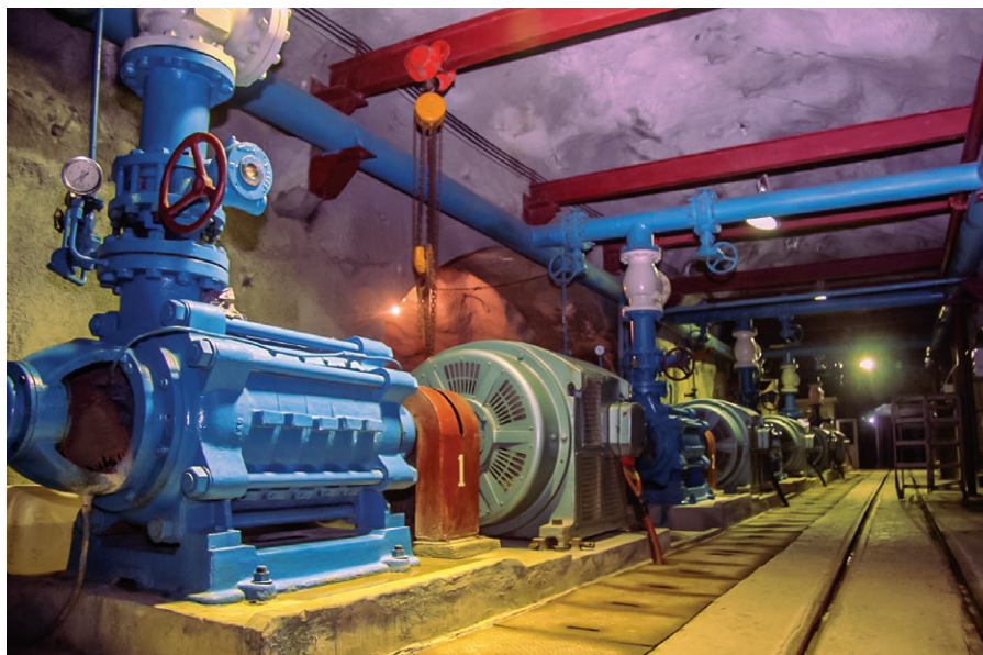
Underground Water Pump Station of MGML
