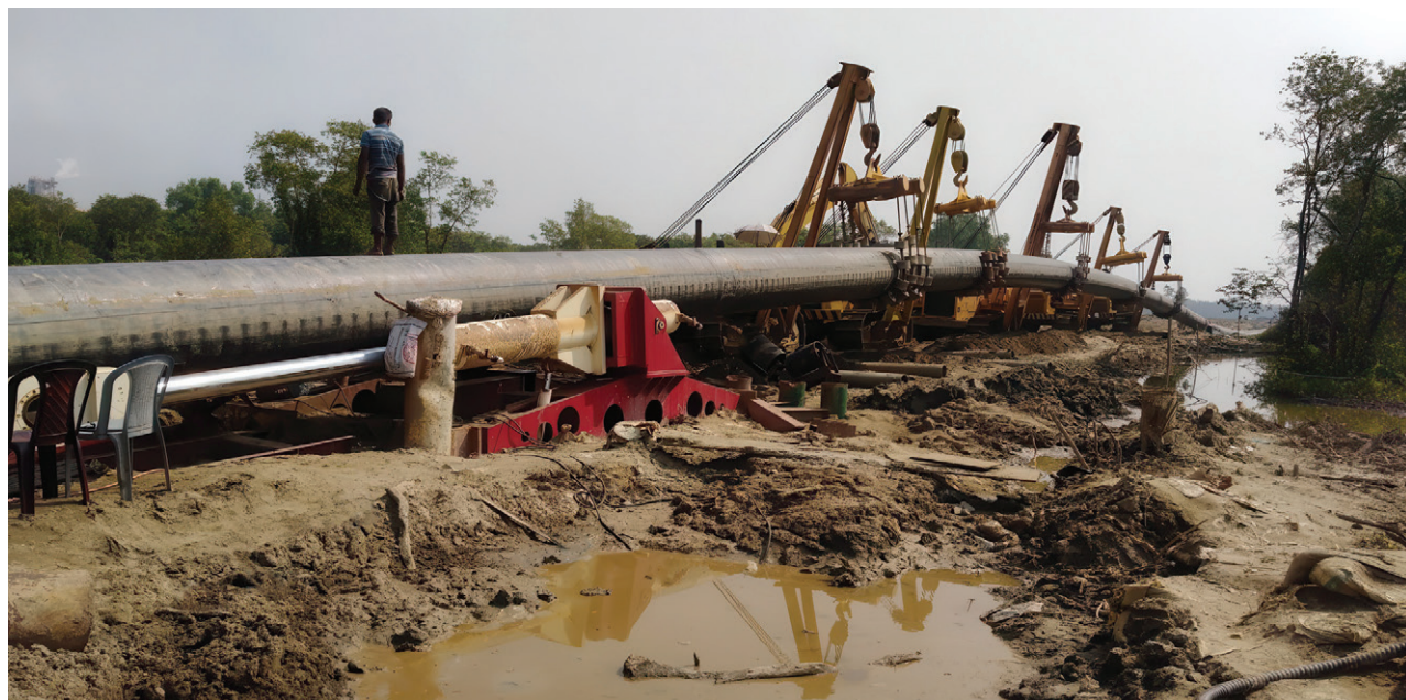
River crossing activities (HDD Method) under Bogra-Rangpur-Saidpur Gas Transmission Pipeline Project of GTCL
