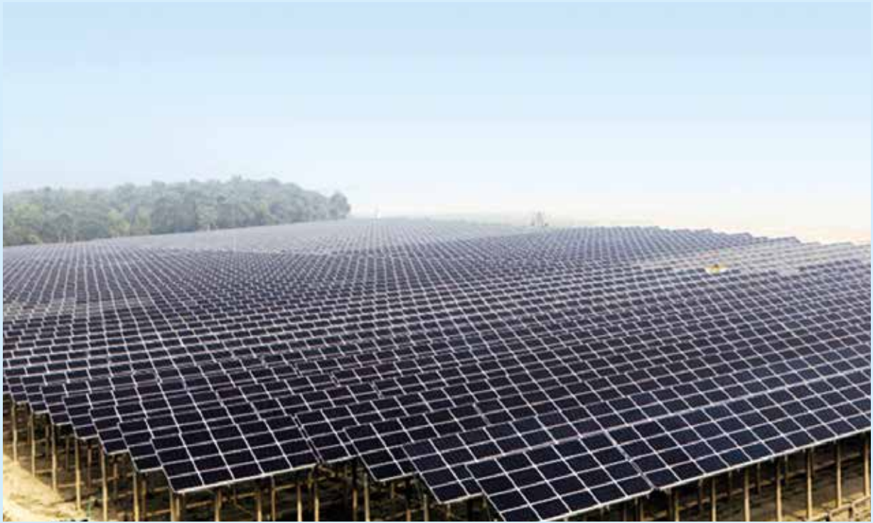
Sirajganj 6.55 MWp Grid Connected Photovoltaic Solar Power Plant
