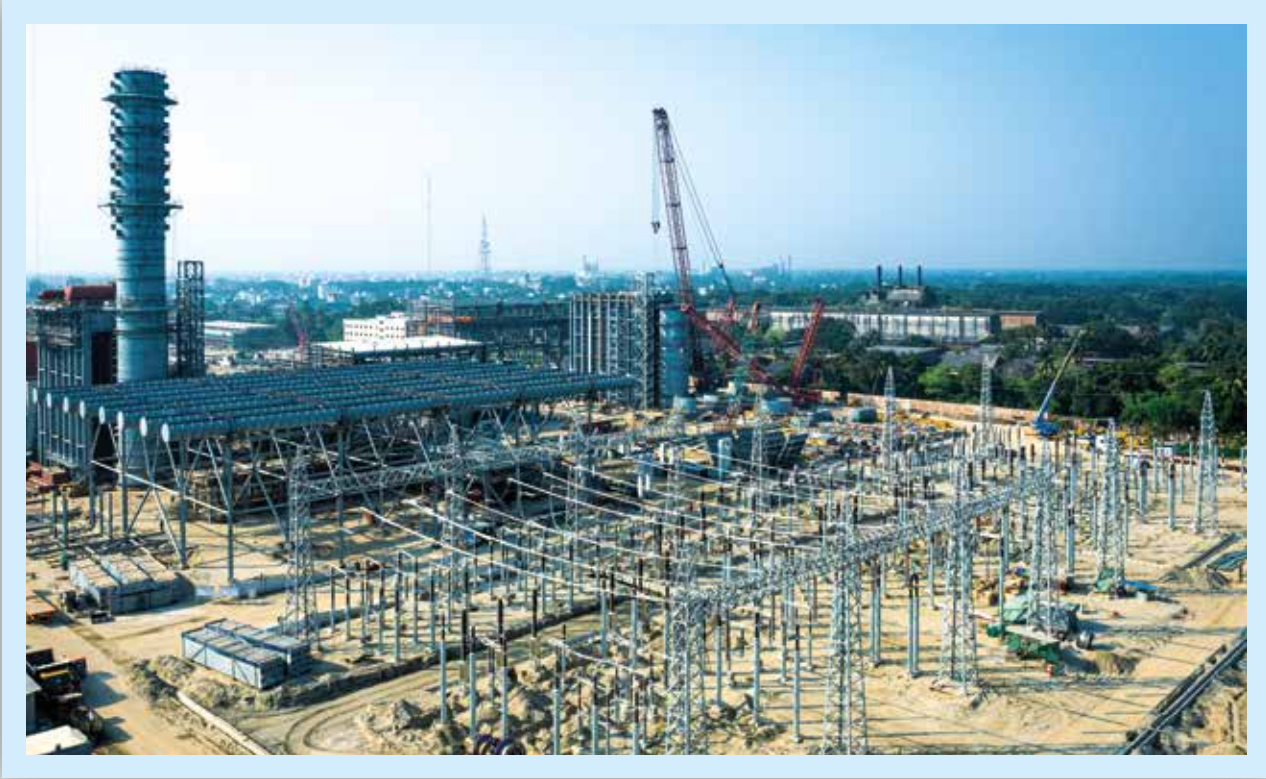
Construction work of substation at Rupsha 800 MW Combined Cycle Power Plant Project
