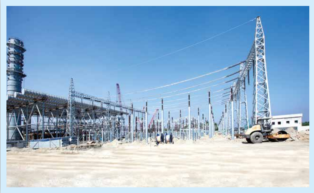
Construction work of substation at Rupsha 800 MW Combined Cycle Power Plant Project
