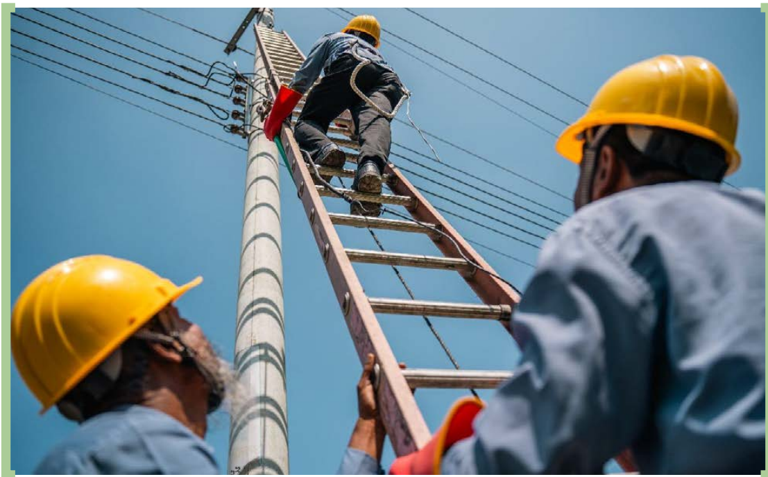
NESCO technical team performing emergency line maintenance work under Sales & Distribution Division-3, Bogura.
