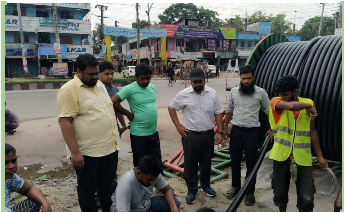
Construction of 33 KV underground line from Rangpur grid to Katkipara NESCO Sub-Station is underway.
