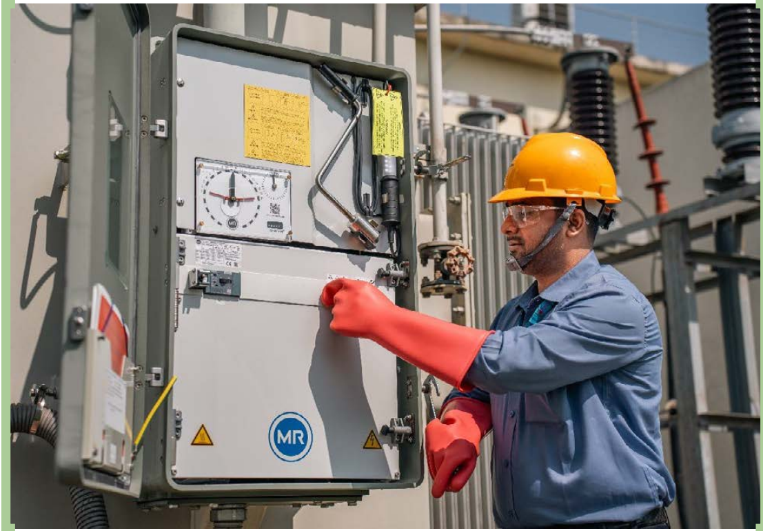
NESCO employee working for Consumer Stable Voltage Supply by Tap changer Operation at the office of Superintending Engineer, Bogura.
