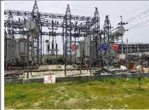
Existing Sub-station/ Proposed bay station
