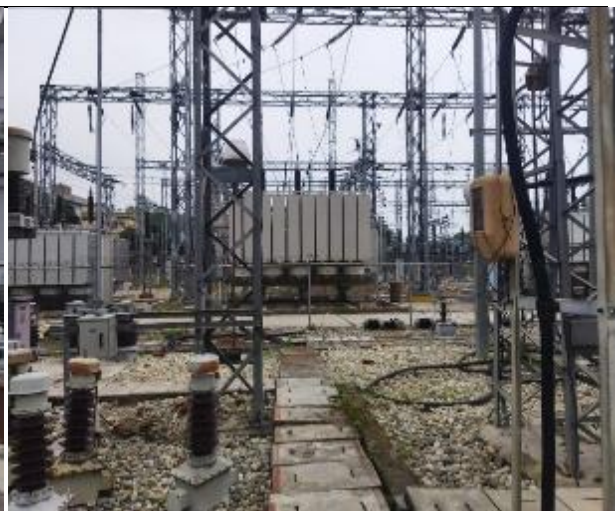
South (Existing Substation)
