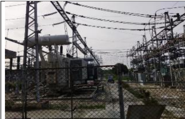
North (PGCB Substation)
