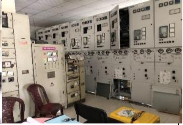
Existing and proposed switching station
