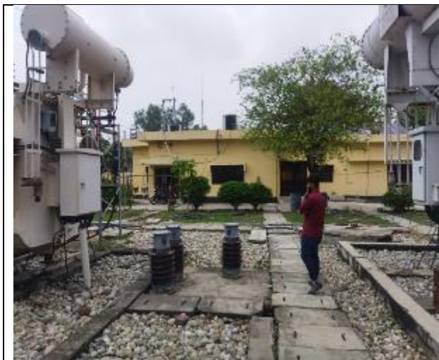
North (Control room)
