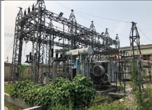
Existing substation picture
