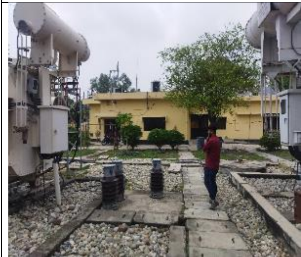
Existing Structures/ substation
