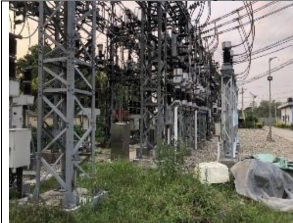
North (Power grid)
