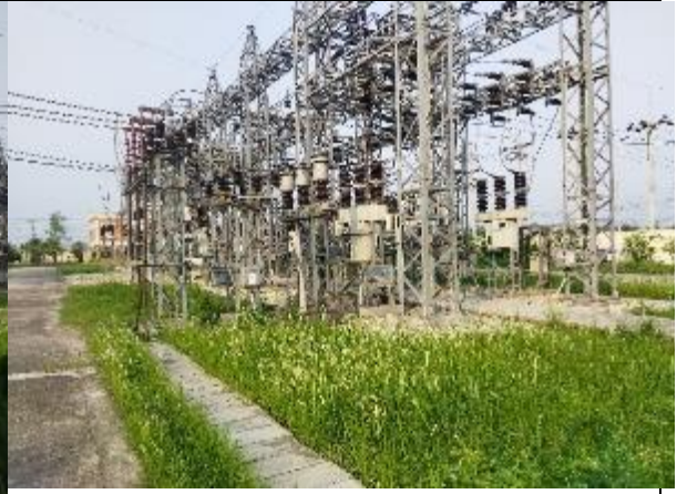
Existing sub-station/ Proposed bay station
