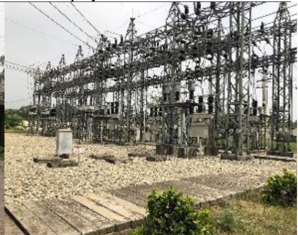
South (PGCB grid, Power plant)
