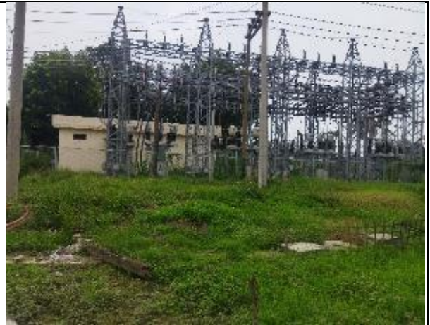
Existing Sub-station/ Proposed bay station
