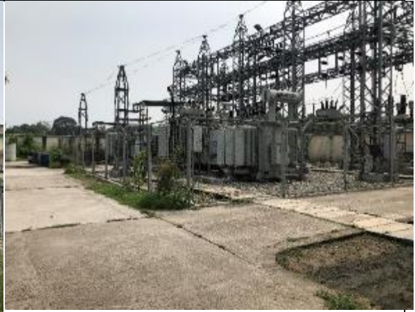
Existing substation picture
