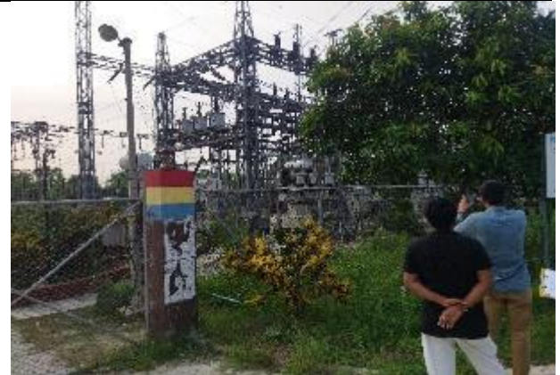
Existing sub-station and proposed switching station
