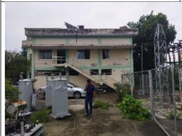
East (Control Room)
