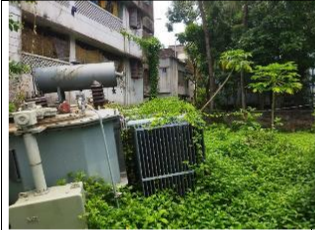
Proposed substation picture
