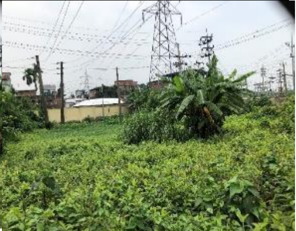
Existing substation picture
