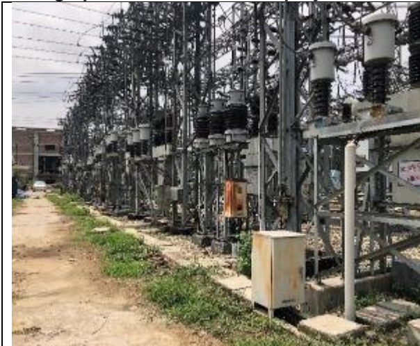
North (PGCB sub station, Access Road)
