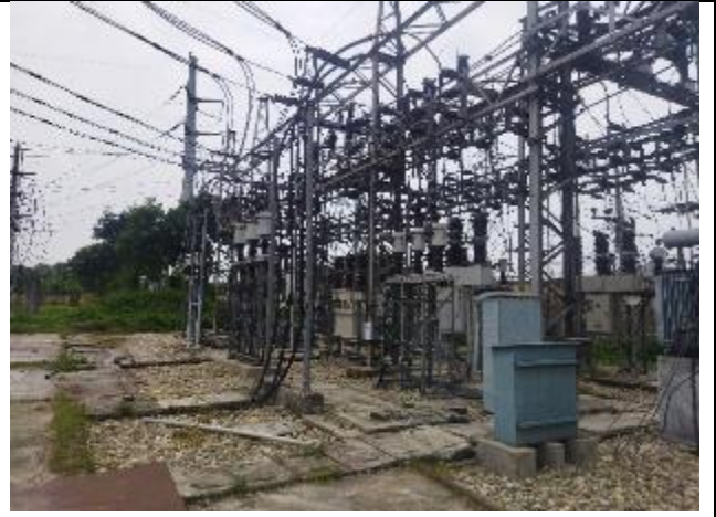
Existing Sub-station Proposed bay station
