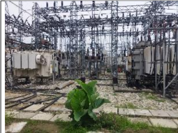
Existing Sub-station/ Proposed bay station
