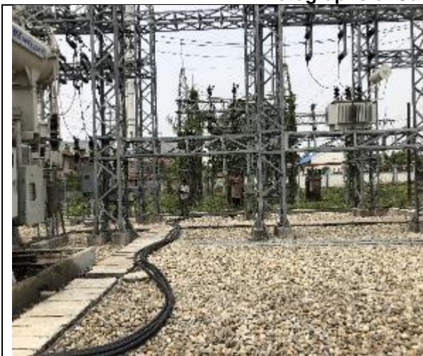
North (Nesco Sub Station grid)
