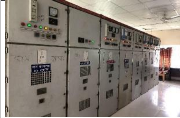
Existing and proposed switching station
