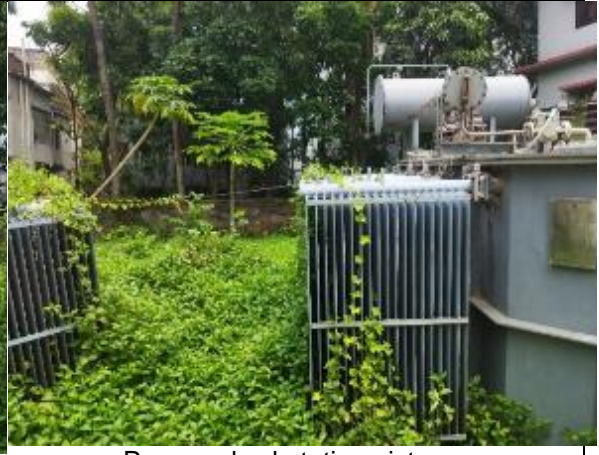
Proposed substation picture
