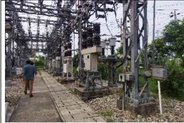
Existing sub-station and Proposed Switching station
