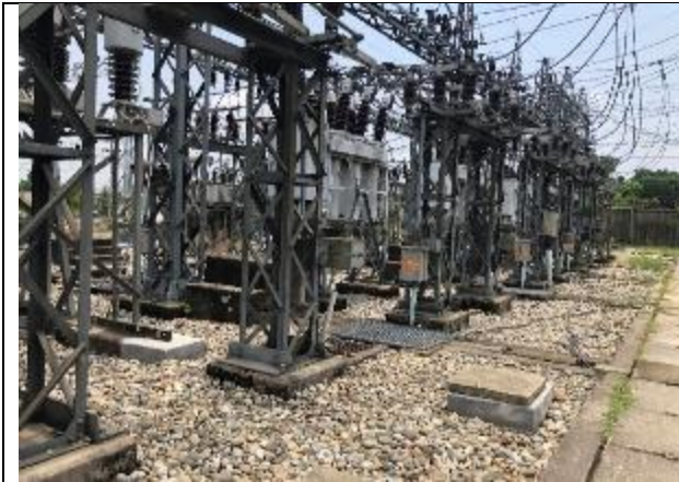
Existing substation and proposed switching station
