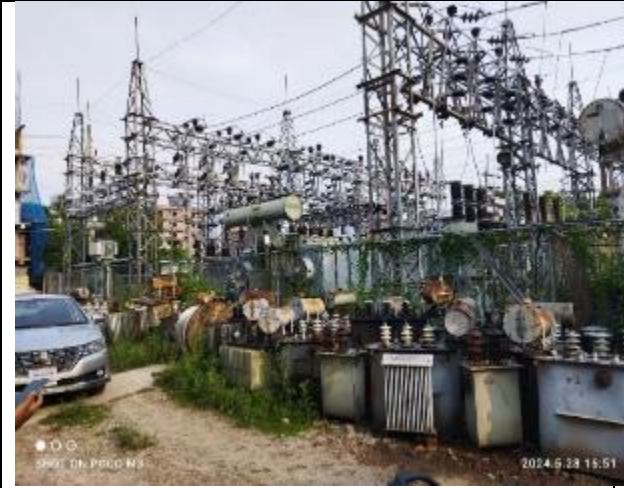
Existing substation picture
