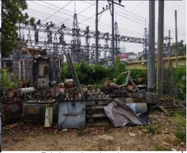
Existing substation picture
