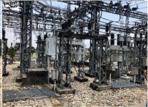
Existing substation and proposed switching station
