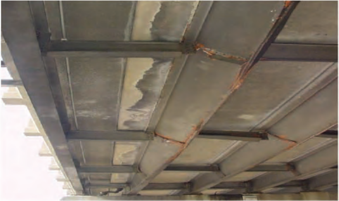
Figure 9.48: Impact Damage to Fascia and First Interior Girder
