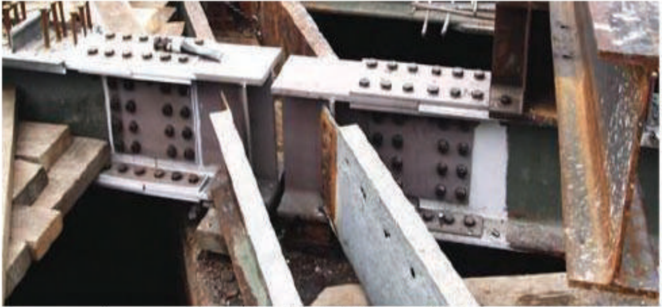
Figure 9.24: Example of a Girder End Repair Utilizing Bolted Splice of a New Full Section
