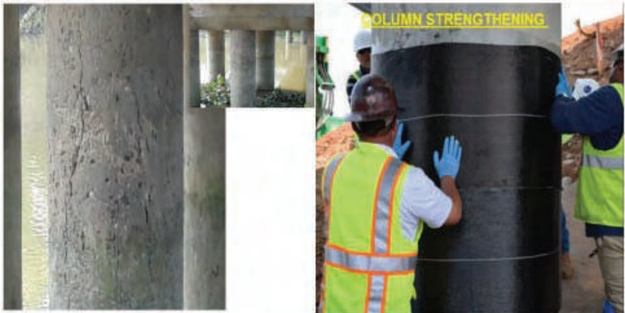
Figure A6.2: Deteriorated Reinforced Concrete Pier Column and Repair using Carbon Fibre Wrap
