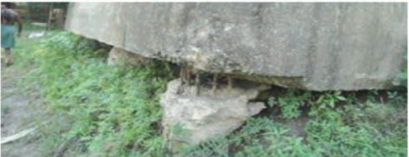
Photo 10.39: Missing concrete and Exposed rebar
