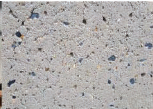
Figure A.8.2: Void and coarse aggregate exposure in concrete surface.
