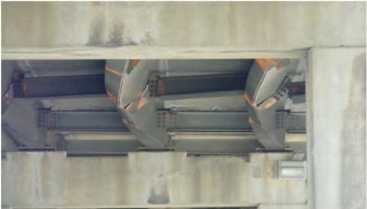
Figure 9.49: Impact Damage that can be Repaired with Heat Straightening
