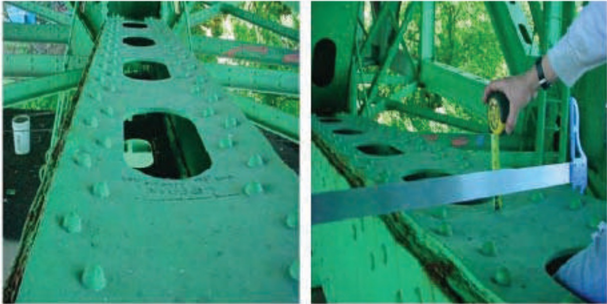
Figure 9.30: Built Up Box Member Corrosion
