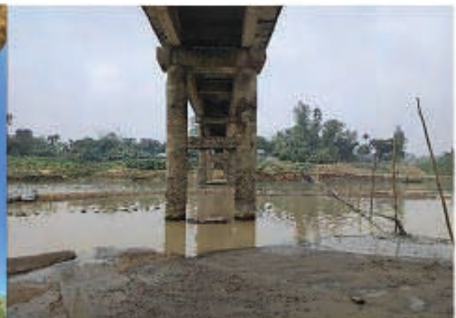
Figure A7.3: Very Poor concreting at the Pier (Scalling)
