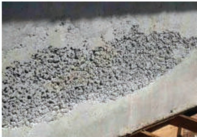
Figure A.8.1: Honeycomb in concrete surface.
