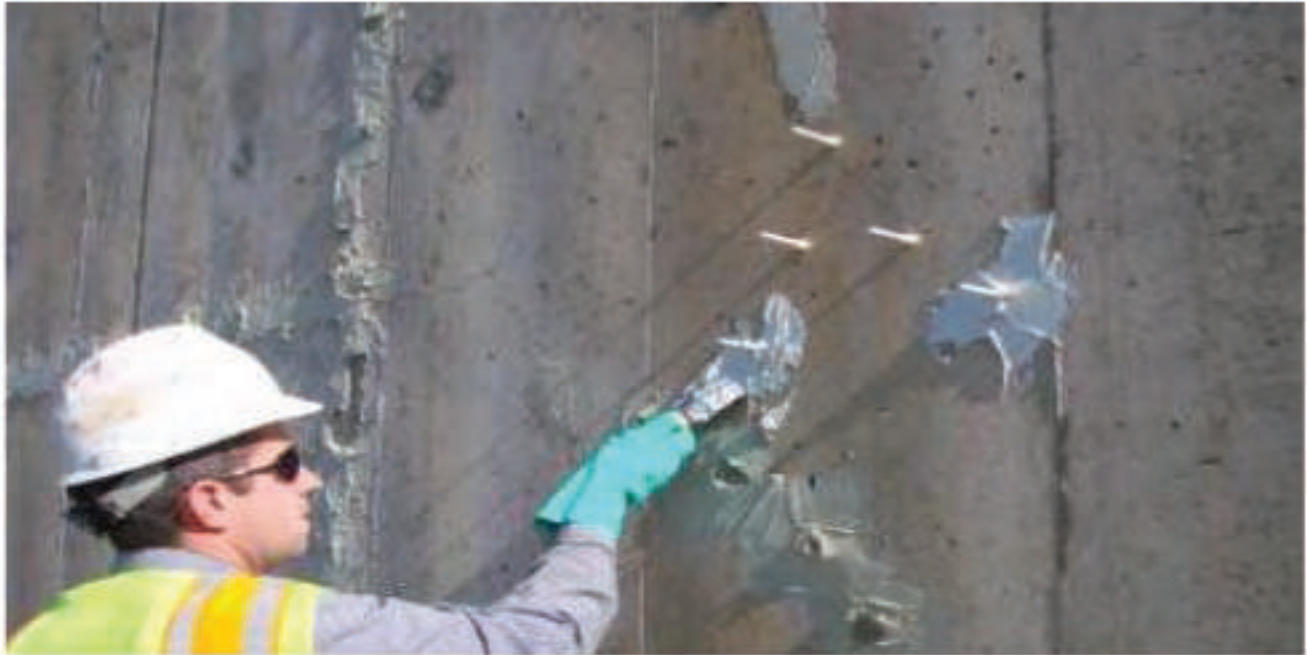
Figure 10.20: Application of Epoxy Resin over Cracks Prior to Injecting (Courtesy of MDOT)
