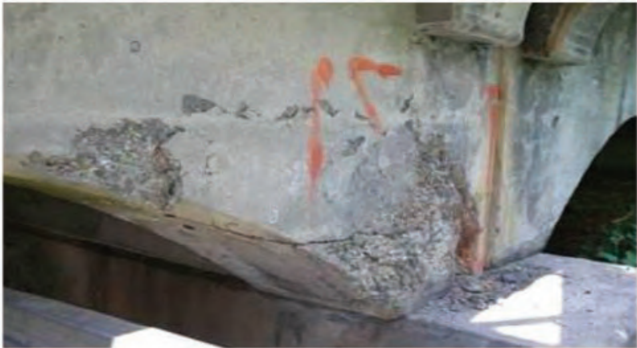
Figure 9.13: Beam End Deterioration
