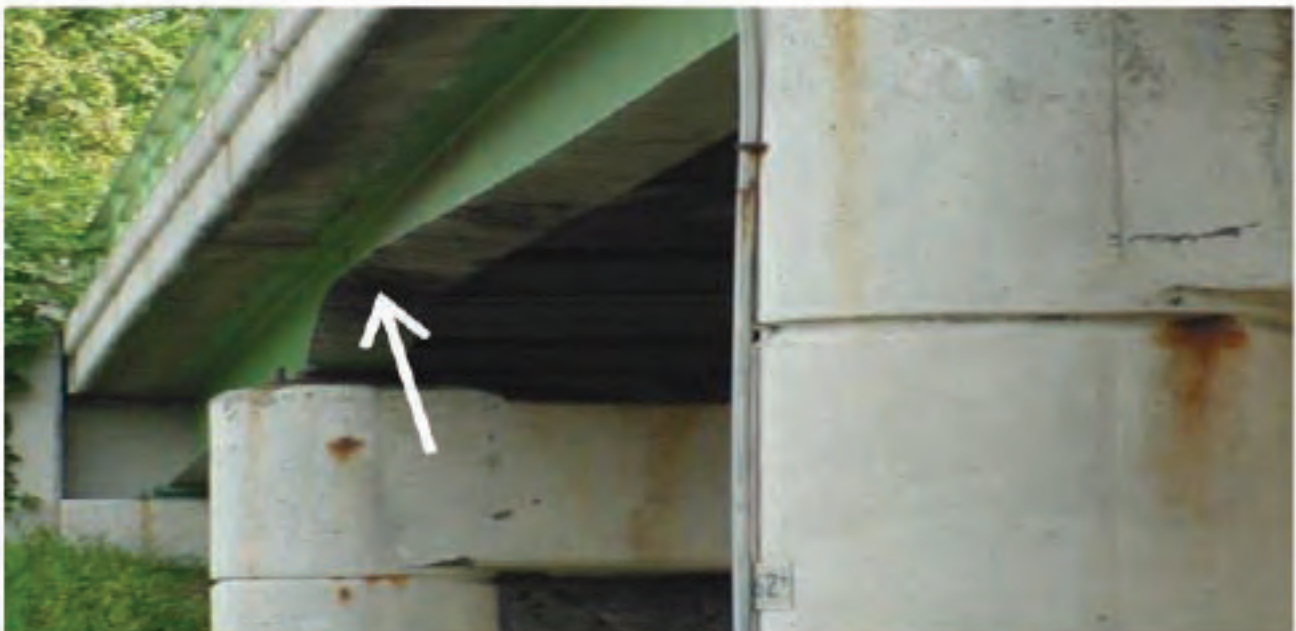
Figure 9.47: Bridge Fascia Girder Damage Caused by Under Passing Vehicle
