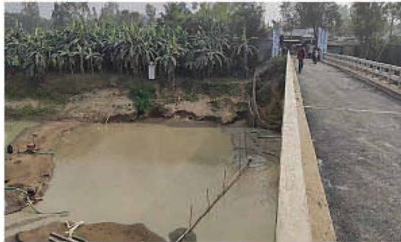
Figure A7.5: Heavy Scour near Abutment
