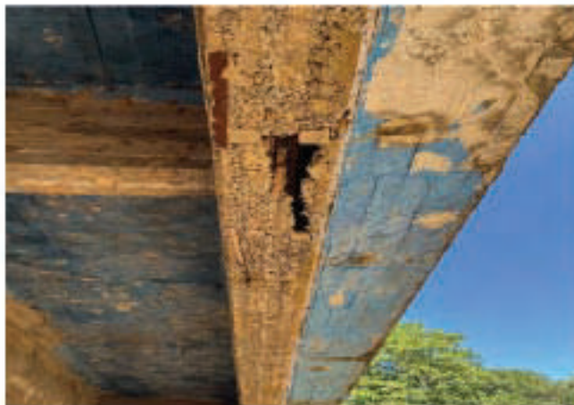
Figure A7.2: Very Poor concreting at the Girder
