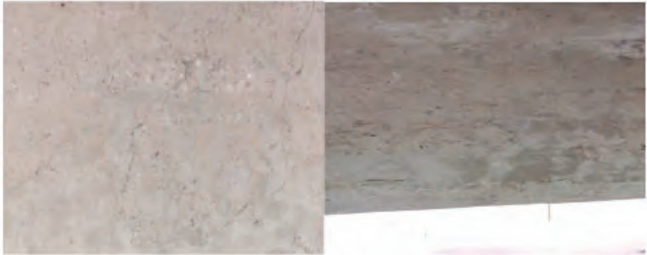
Figure A4.1: Girder Cracks
