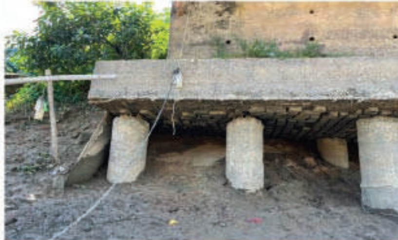
Figure A7.1: Scouring at Abutment and disintegrated Pile from Pile Cap
