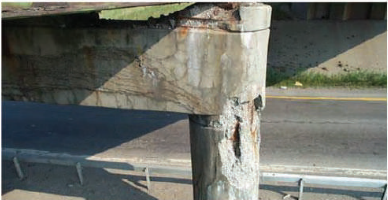
Figure 10.14: Pier Cap and Column in Need of Structural Rehabilitation
