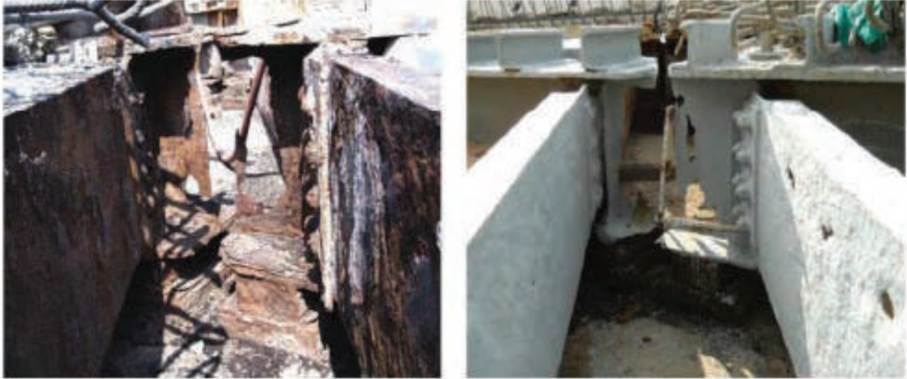
Figure 9.23: Corrosion Damage at Girder Ends (Concrete Deck has been Removed)
