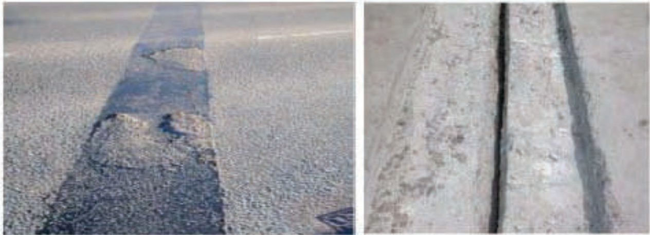
Figure 9.59: Damaged Asphaltic plug joint after removing Sealant of Asphaltic plug joint
