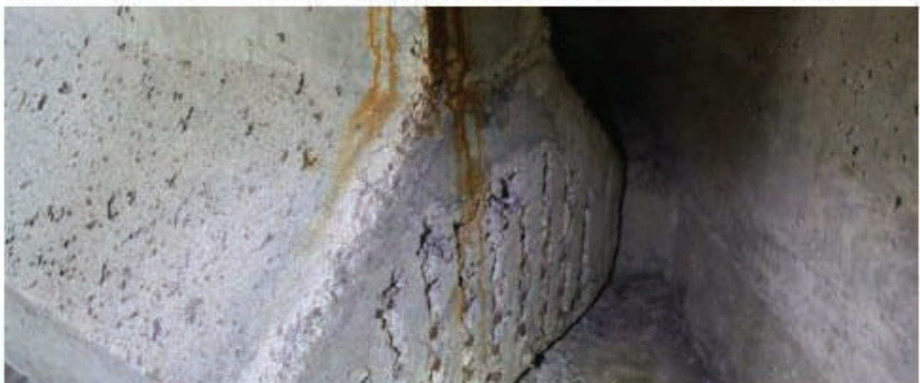
Figure 9.1: Exposed Strands on End of Precast Prestressed Concrete Girder
