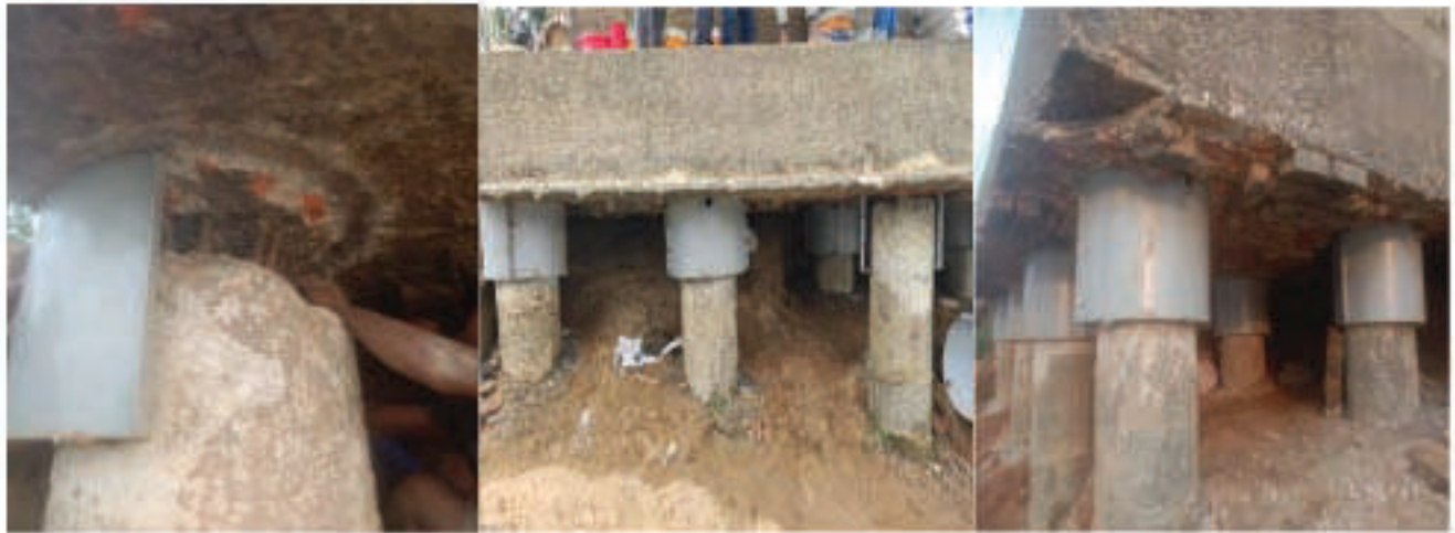
Figure A7.4: Damaged pile surface preparation and installed Casing
