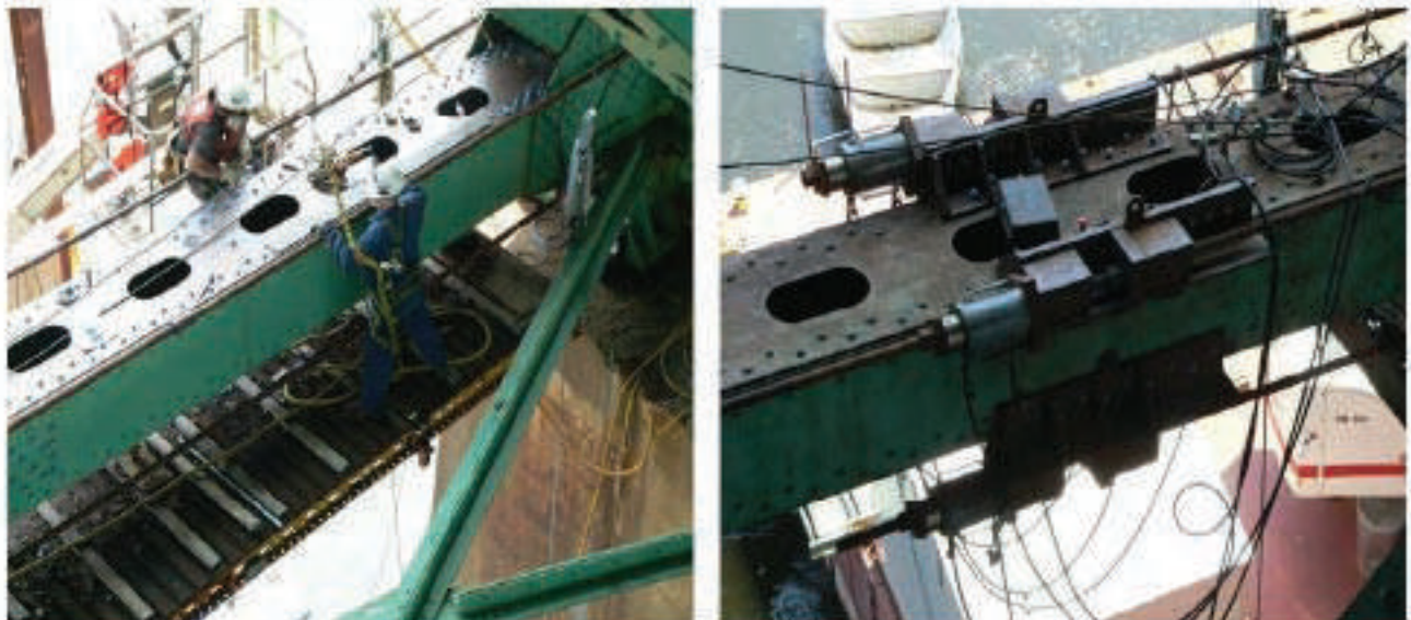
Figure 9.31: Repair of Bottom Chord Plate (left) Utilizing Thread Bars and Jacks (right)
