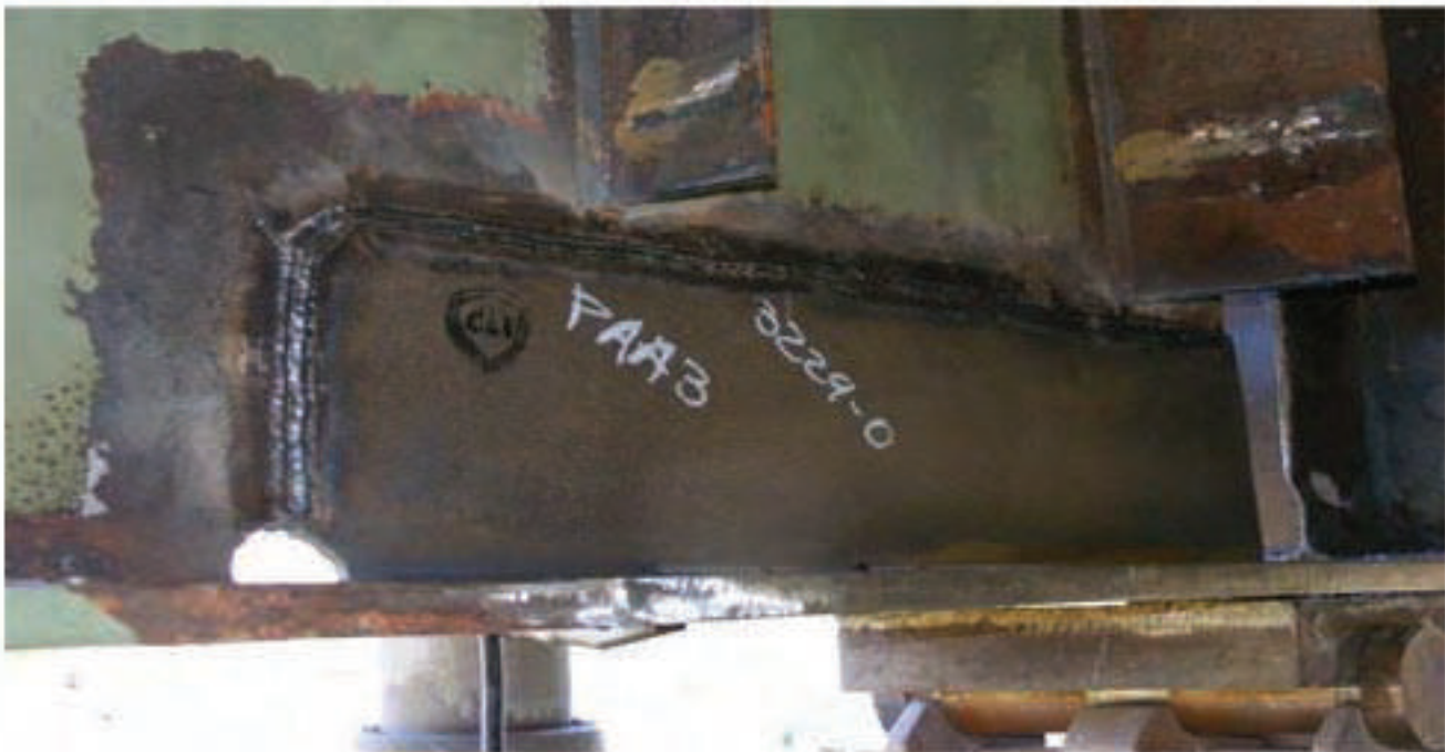
Figure 9.25: Repair in Progress using Tee – Section Cut Out Form a Matching W Section
