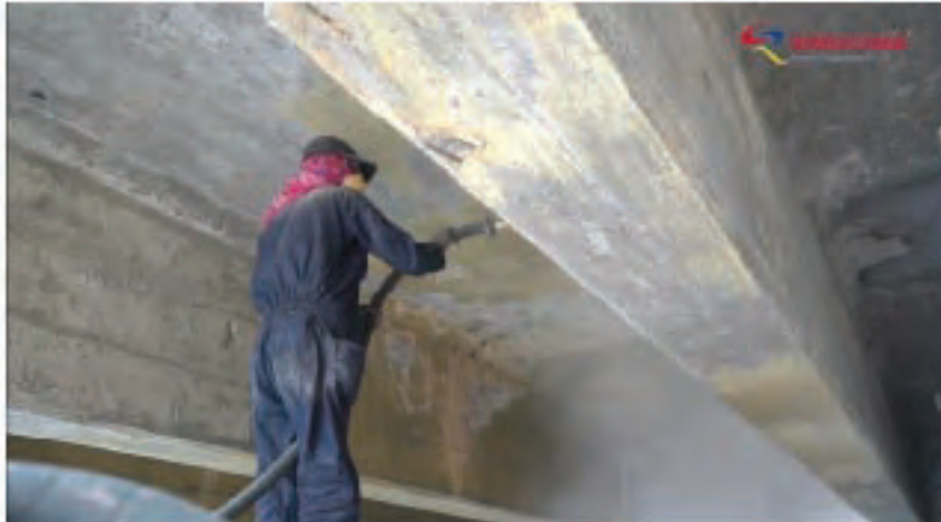
Figure A.8.10: Application of Water based cement paint in the Deck Slab Bottom
