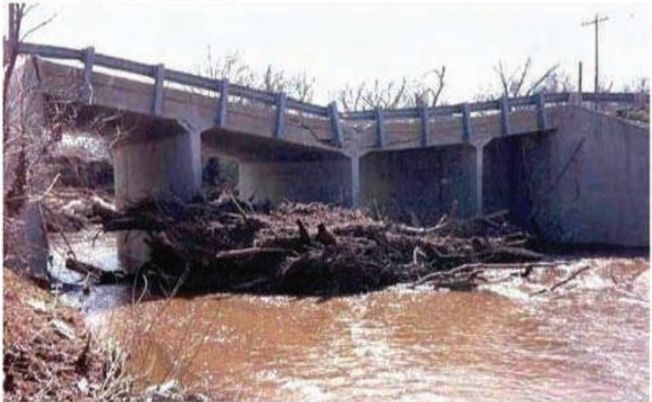
Figure 11.6: Increased Scour at Bridge Piers as a Result of Debris
