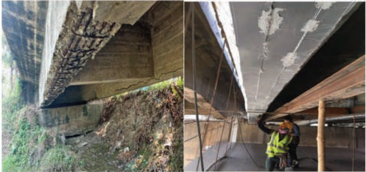
Figure A6.1: Deteriorated Reinforced Concrete Girder and Repair using Carbon Fibre Laminate
