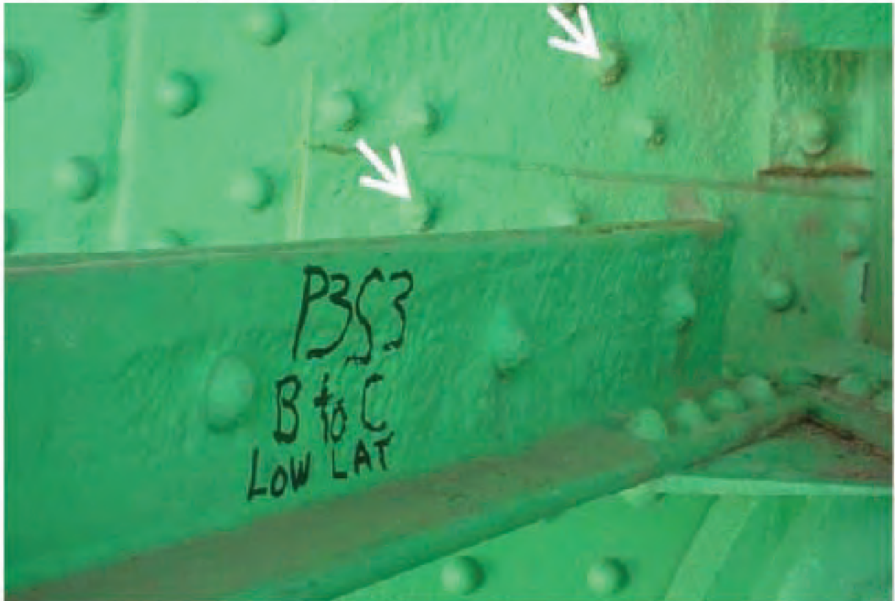
Figure 9.39: Rivet Heads Exhibiting Various Degrees of Corrosion
