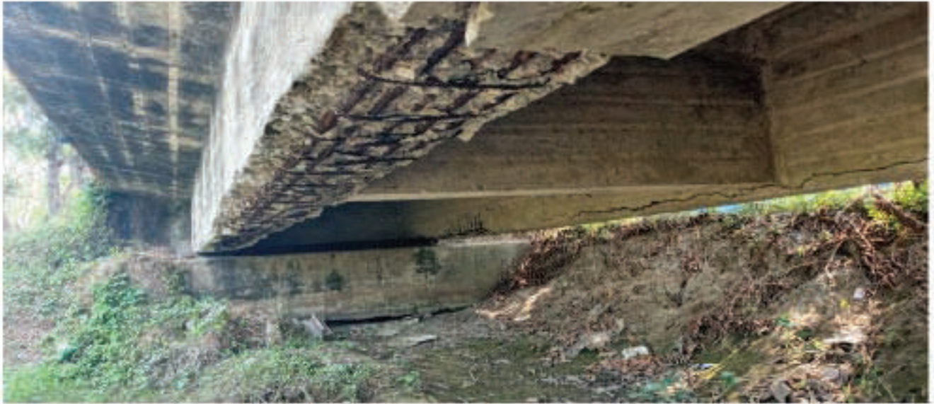
Figure 10.45: Exposed bar of bottom of girder
