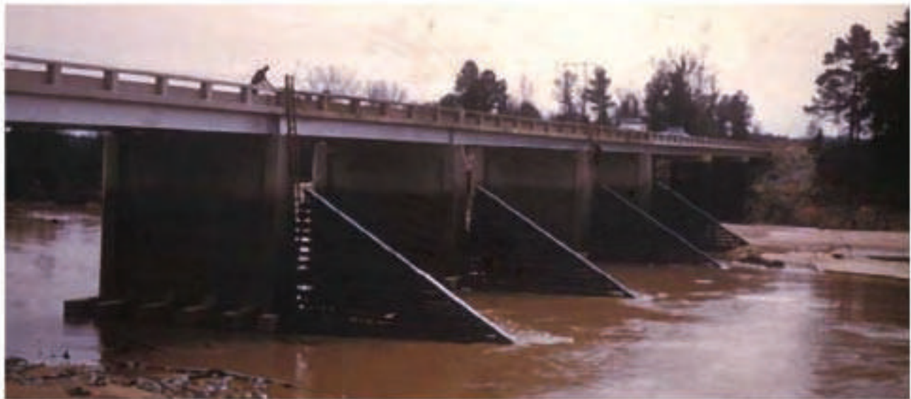
Figure 11.10: Timber Debris Fins with Sloping Leading Edge
