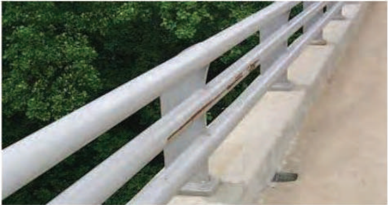
Figure 8.47: Galvanized Steel Rail
