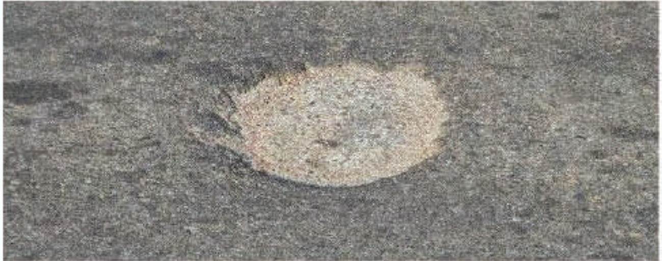
Figure 3.2: Potholes in wearing surface
