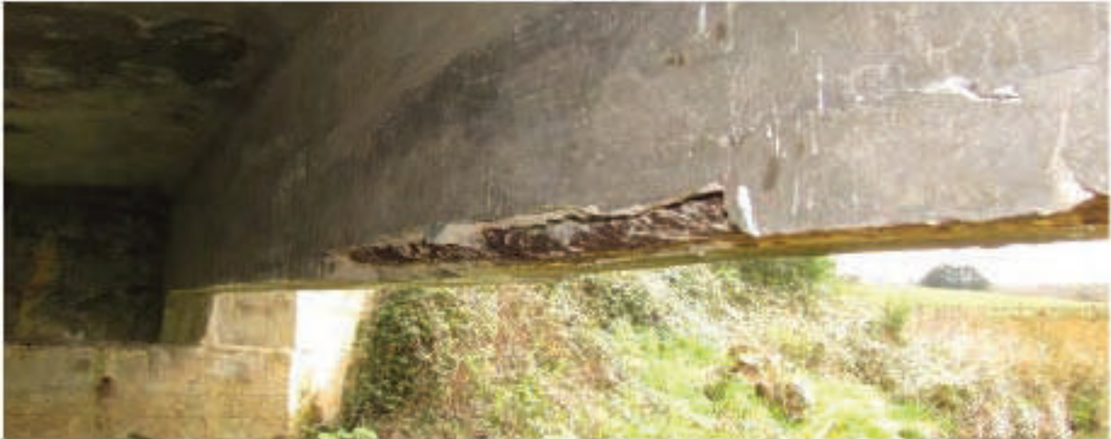
Figure 7.16: Severe corrosion of reinforcement
