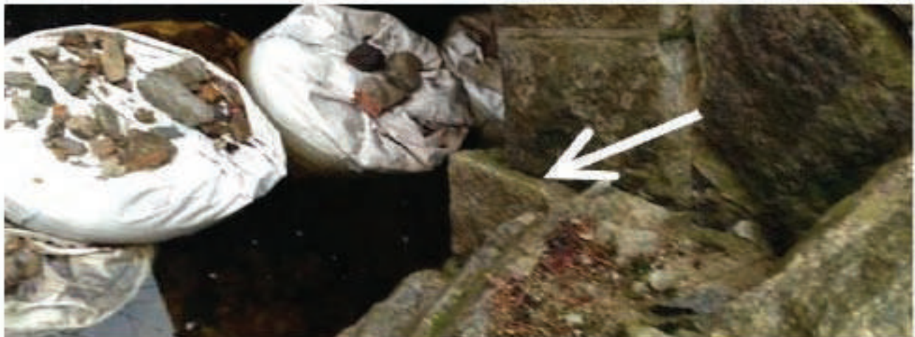
Figure 5.1: Mortar Deterioration (indicated by arrow)
