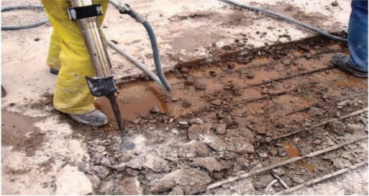
Figure 8.24: exposed reinforcing steel layers
