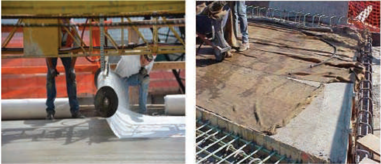
Figure 8.30: Concrete Wet Cure Examples. Wet Cure Blanket (left) and Burlap Sheets (right)
