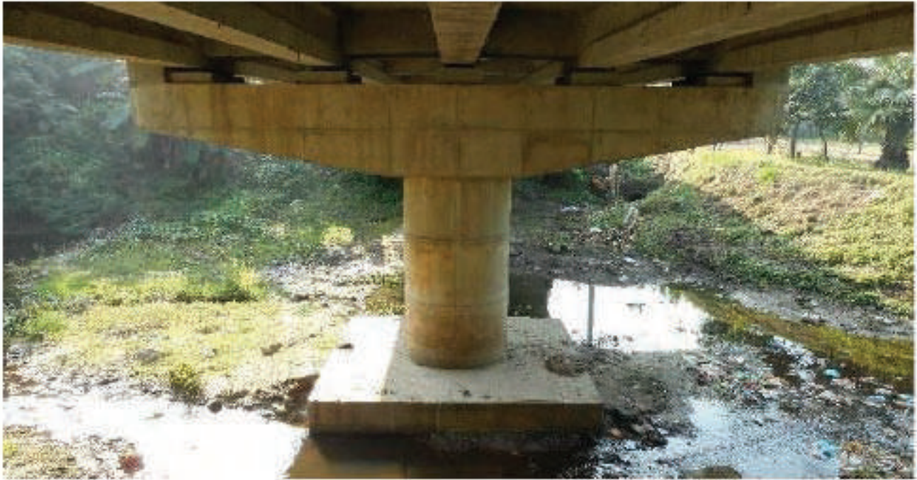
Figure 3.12: Scouring of bed materials
