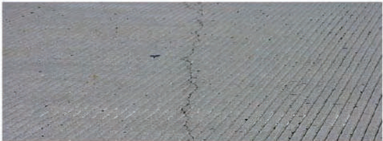
Figure 8.3: Typical Discrete Cracking Pattern on a Deck
