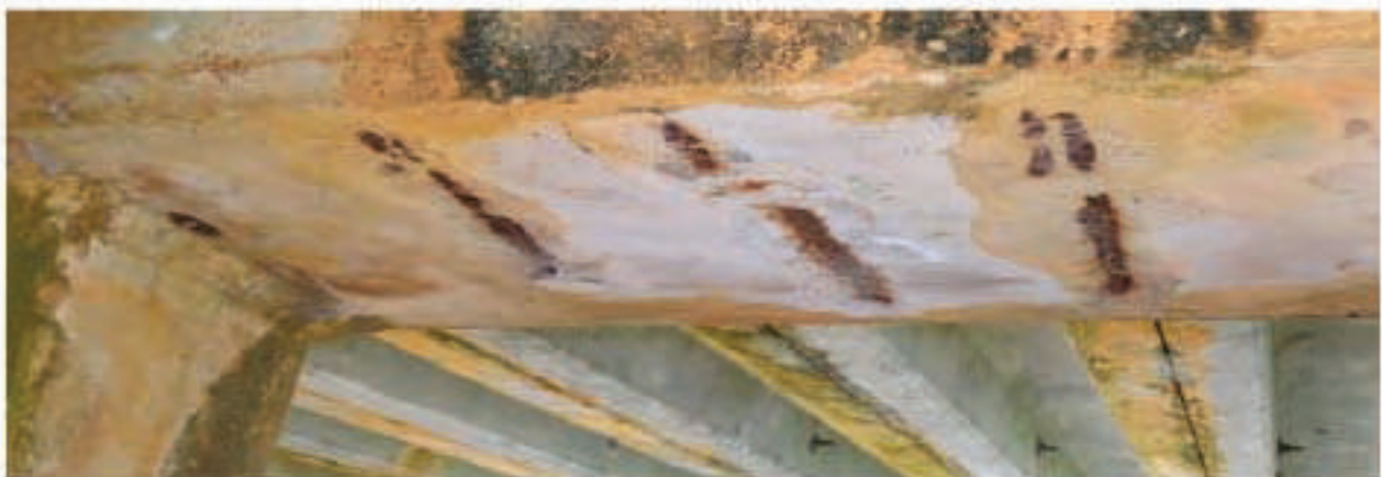
Figure 7.15: Reinforcement corrosion of concrete
