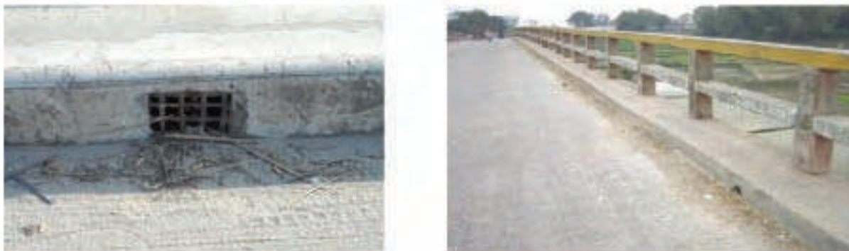
Figure 3.1: Blocked Drainage Inlets
