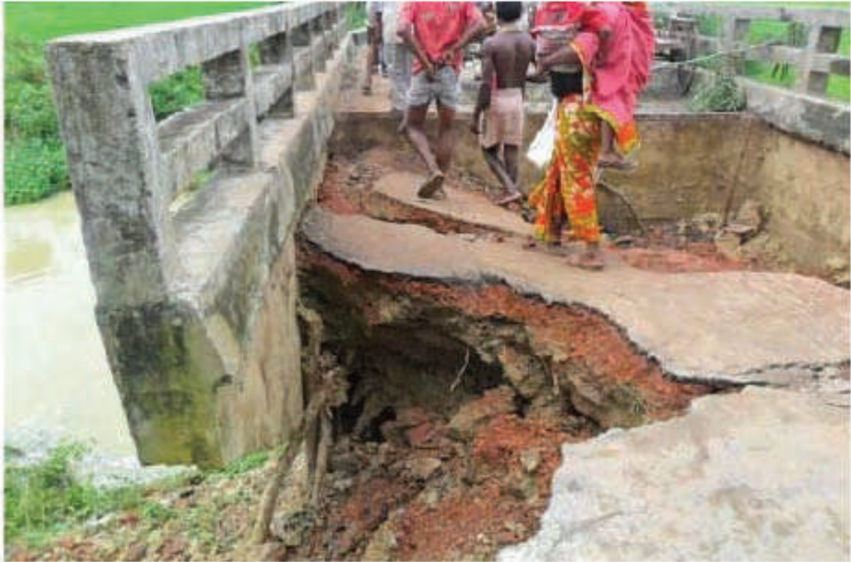
Figure 3.13: Settlement of approach embankment
