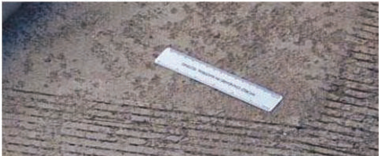
Figure 6.5: Scaling on a Bridge Deck
