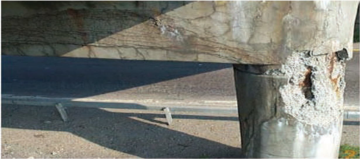
Figure 6.29: Severely Deteriorated Concrete Pier
