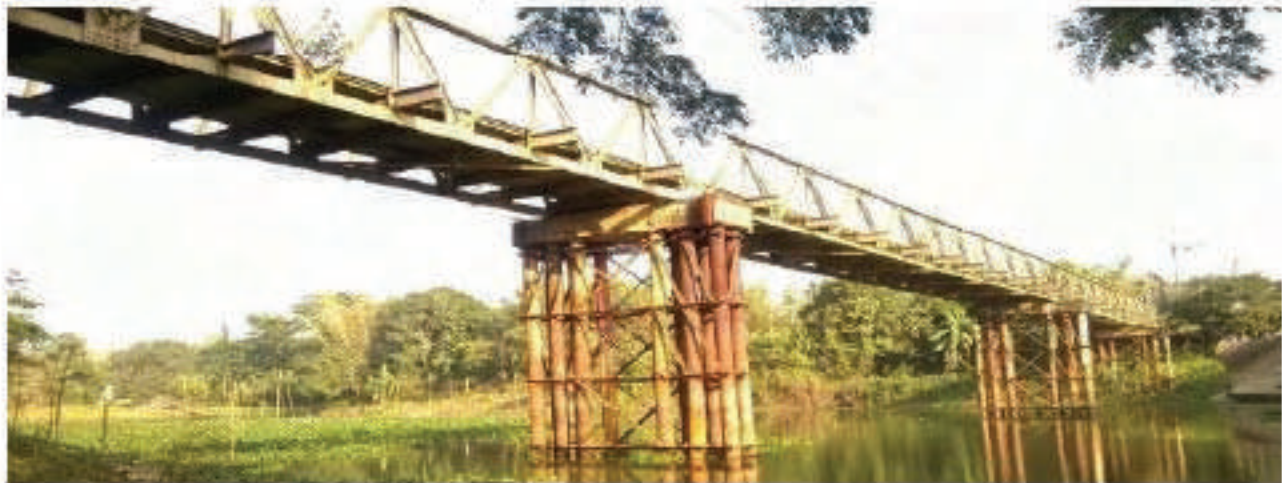
Figure 3.10: Steel member corrosion
