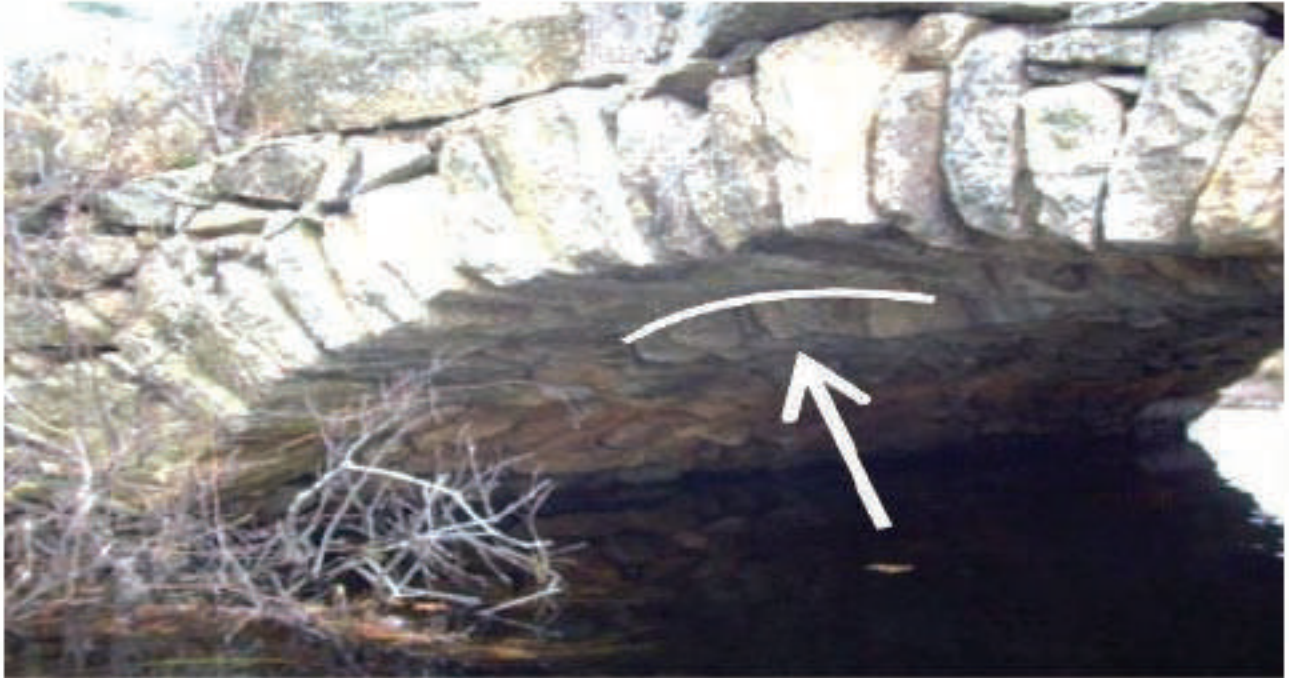
Figure 5.3: Multiple Slipped Stones
