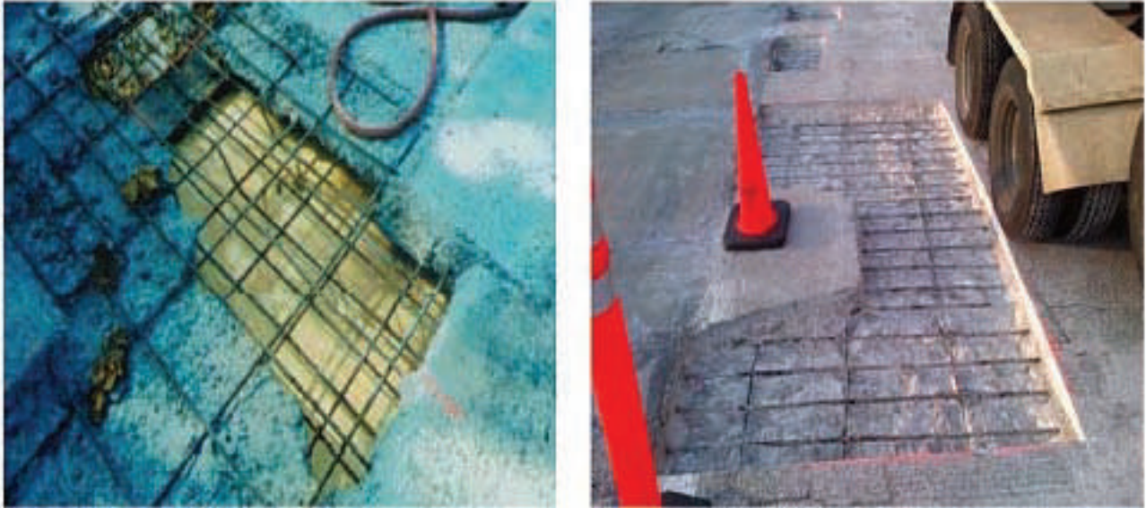
Figure 8.21: Concrete Repair Photos. Full Depth Repair (left) and Partial Depth Repair (right)
