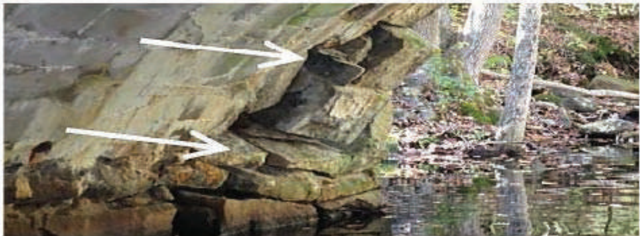
Figure 5.6: Arch Deformation caused by Masonry Displacement
