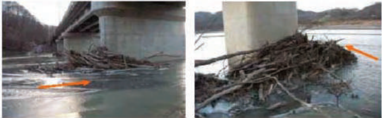
Figure 3.8: Pier with flow obstruction
