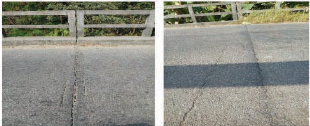
Figure 3.3: Cracks in the wearing surface
