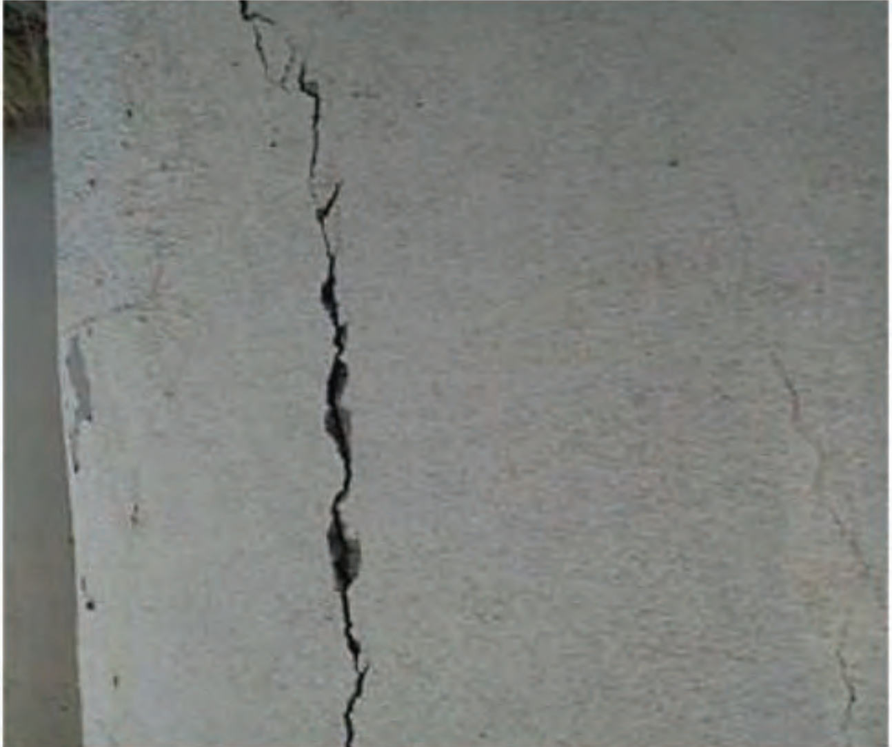
Figure 6.2: Vertical Crack on a Pier Column
