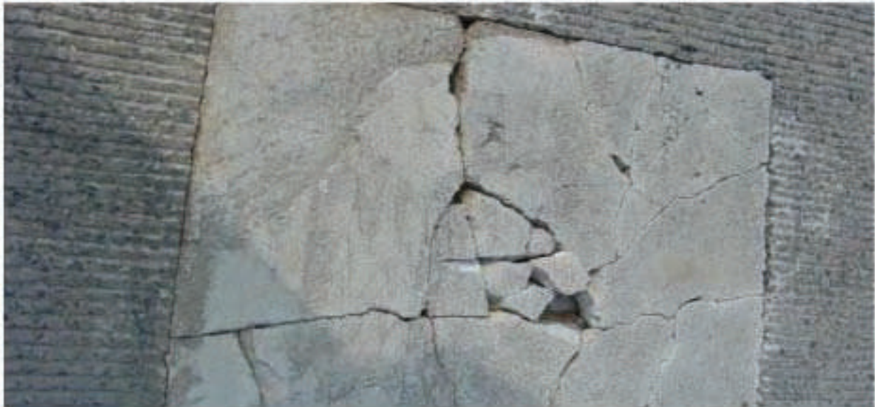
Figure 6.48: Failure of Rapid-Setting Mix
