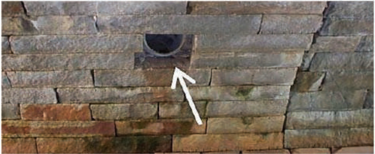
Figure 5.5: Missing Stones in a Masonry Arch
