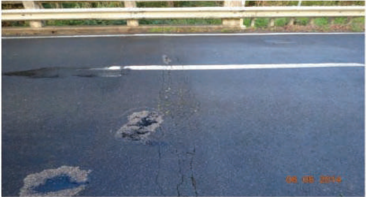
Figure 8.40: Potholes on the deck
