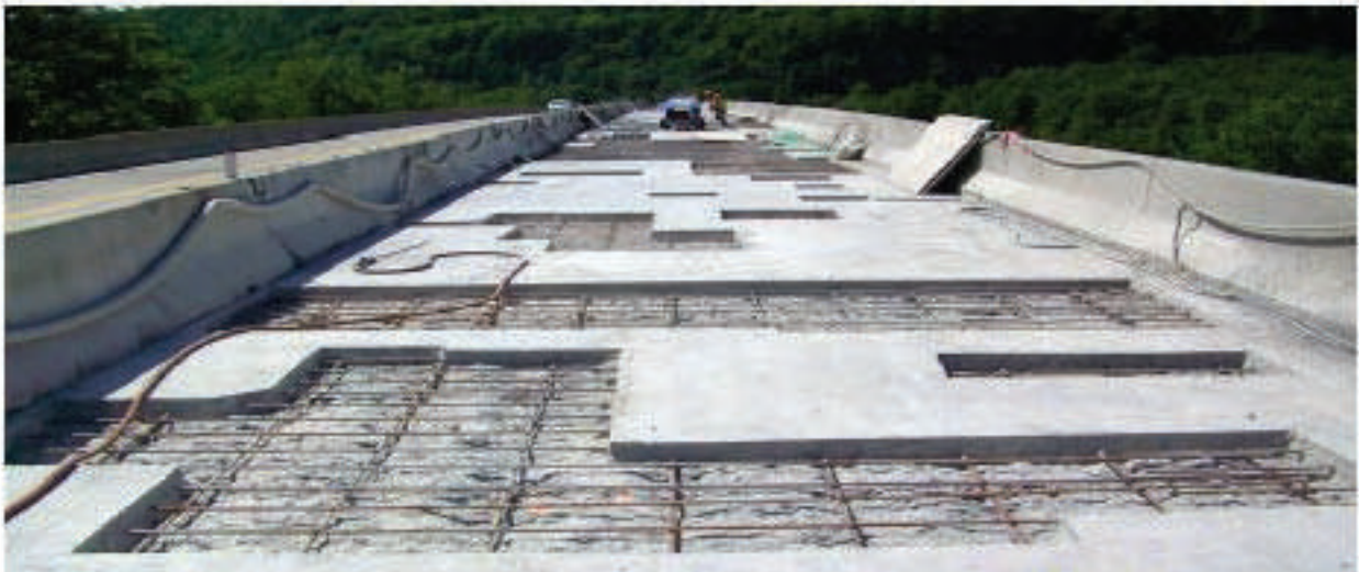
Figure 6.36: Extensive Patching on a Bridge Deck
