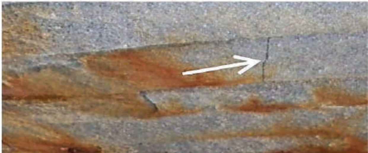
Figure 5.2: Transverse Crack in Stone Arch
