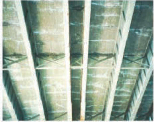
Figure 7.7: Cracking from Thermal Effects
