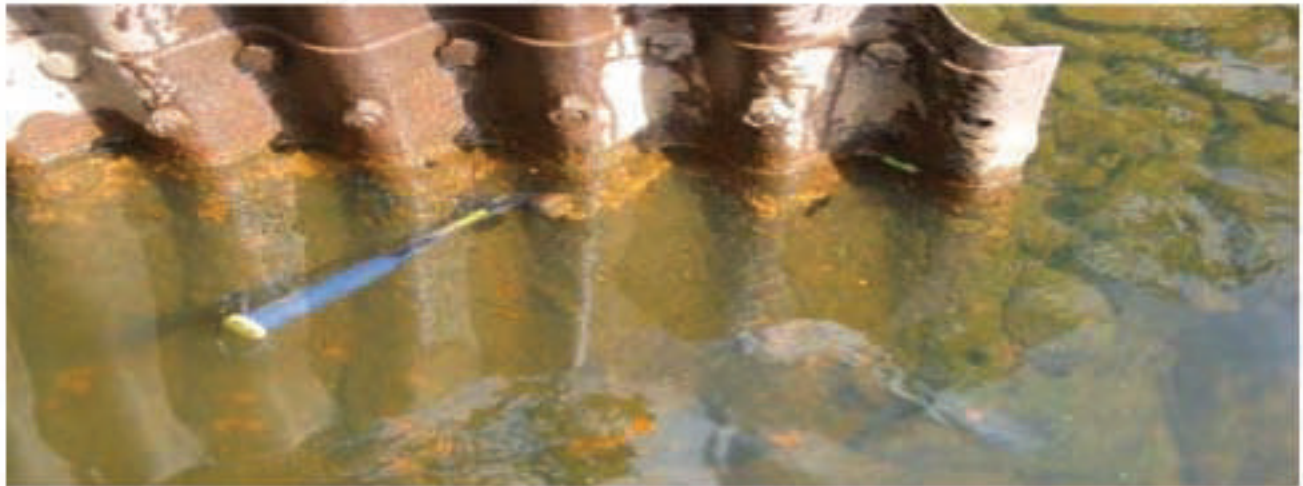
Figure 4.2: Corrosion in Plate Arch
