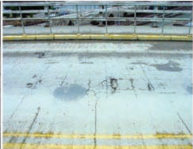
Figure 7.9: Spalls and Cracking
