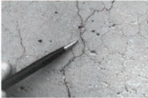
Figure 6.3: ASR Cracks in a Concrete Column
