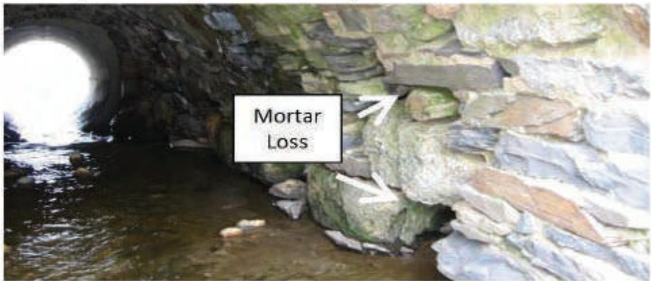
Figure 4.5: Mortar Loss in Bottomless Masonry Arch
