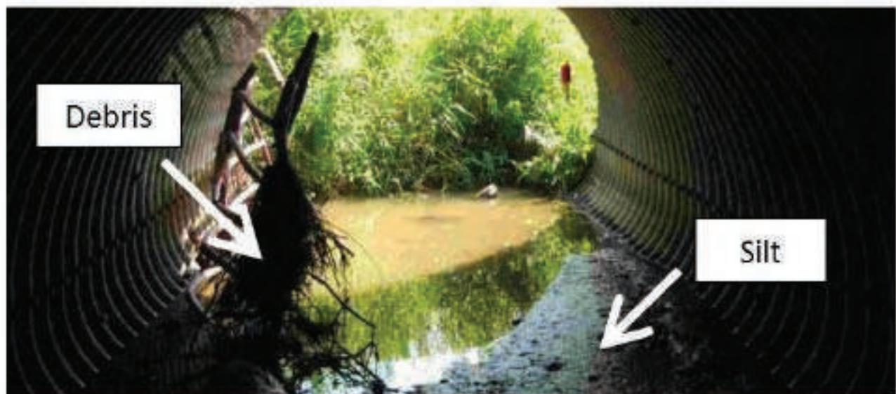
Figure 4.1: Debris and Silt in Corrugated Culvert
