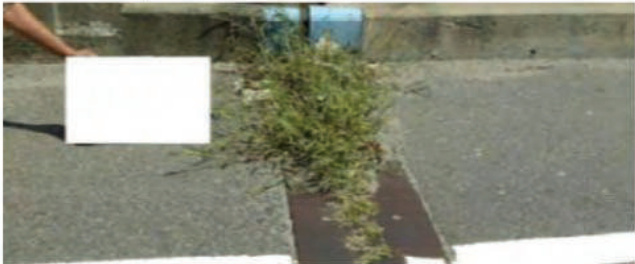
Figure 3.4: Blocked expansion joint
