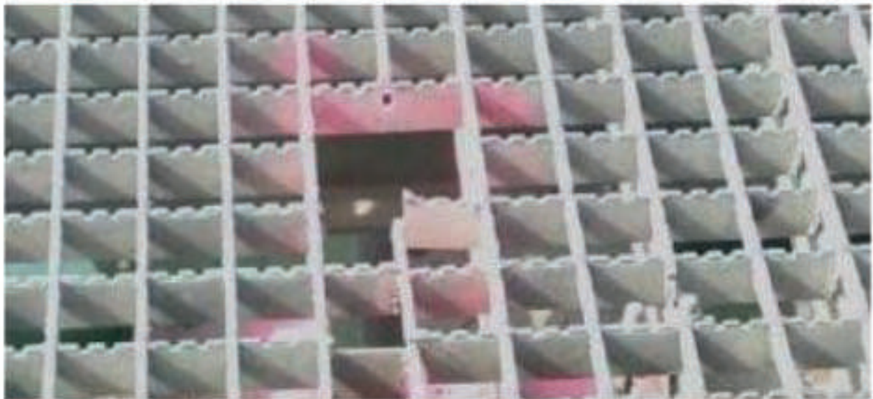
Figure 8.41: Typical Broken Grid Section
