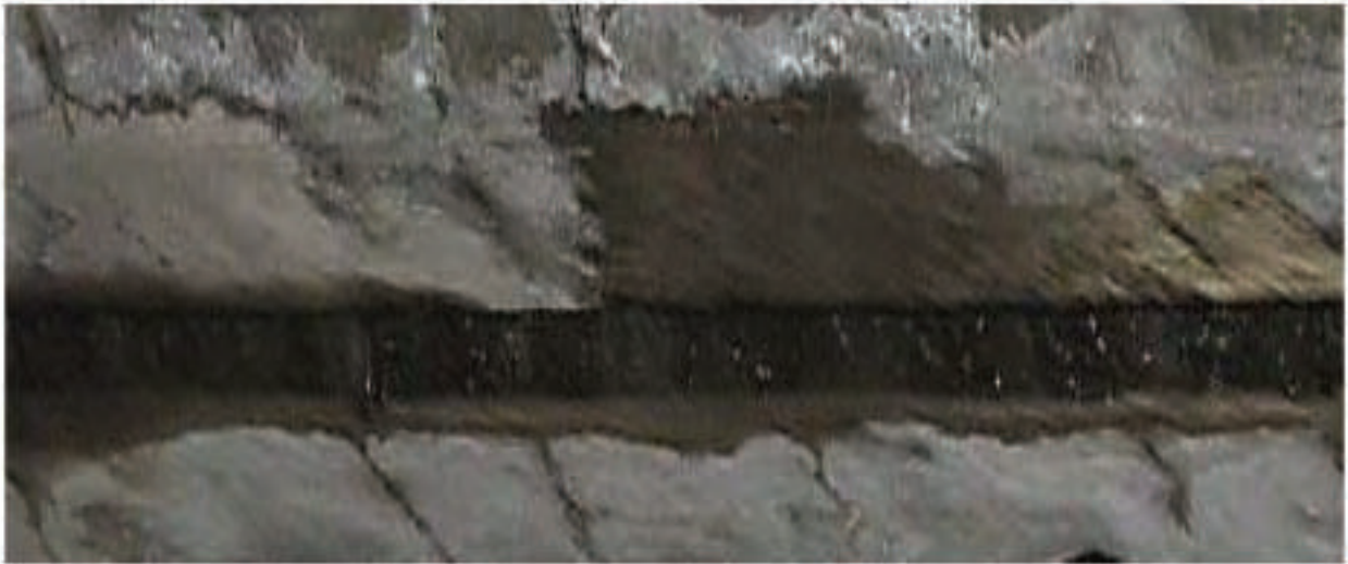
Figure 7.19: Shear key failure of U-Slab bridge
