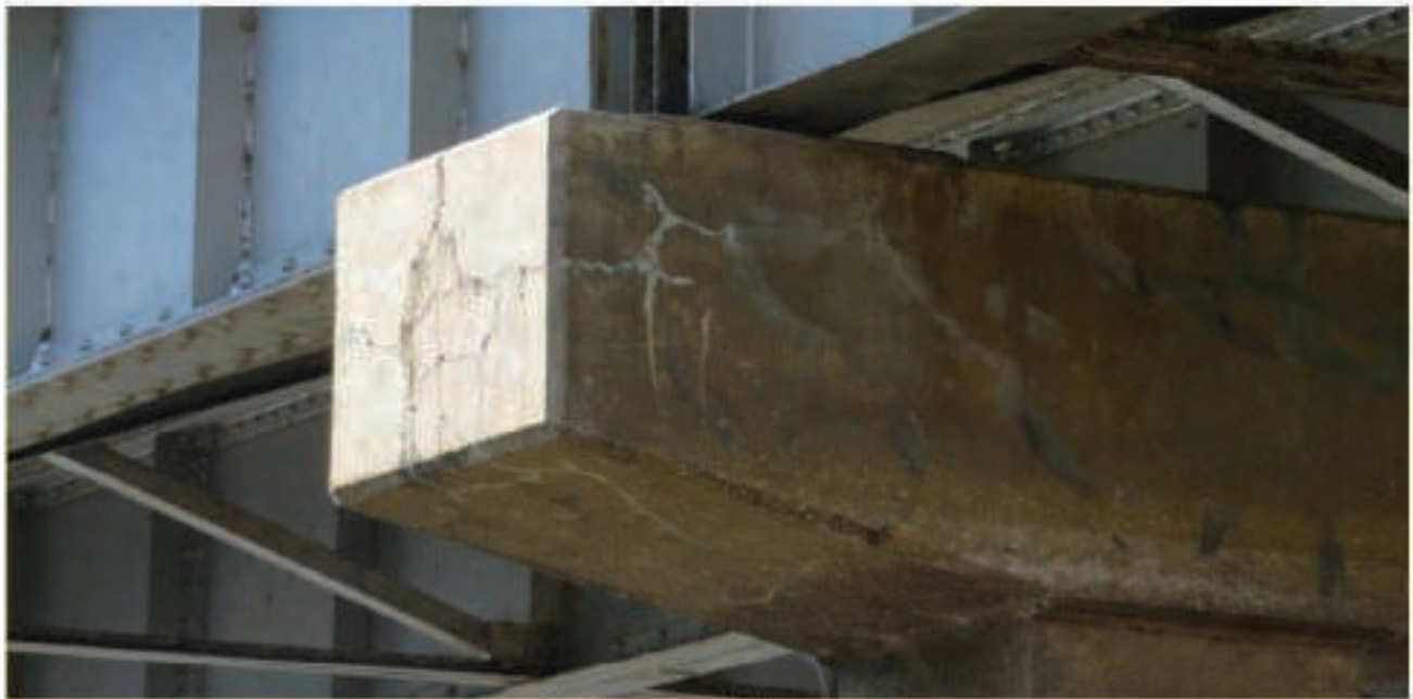
Figure 7.12: Cracks due to AAR
