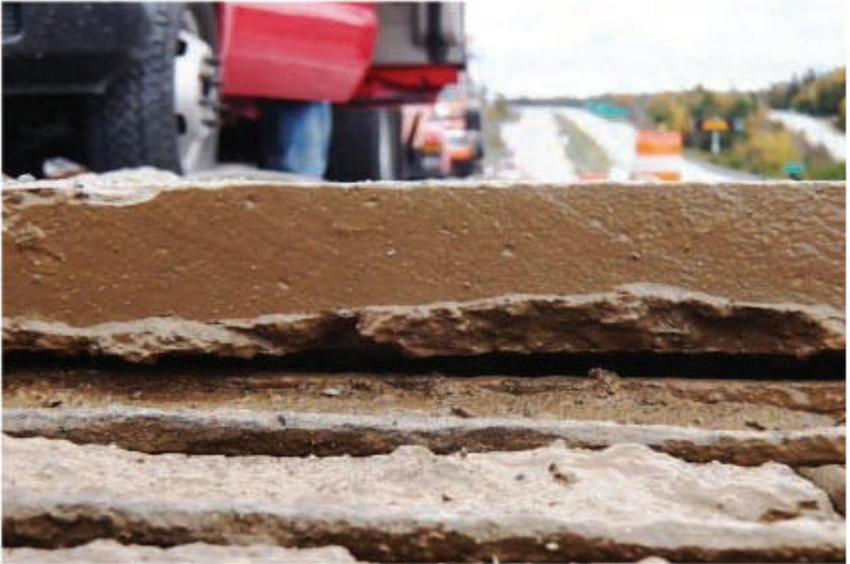
Figure 8.25: Delamination at Edge of Patch
