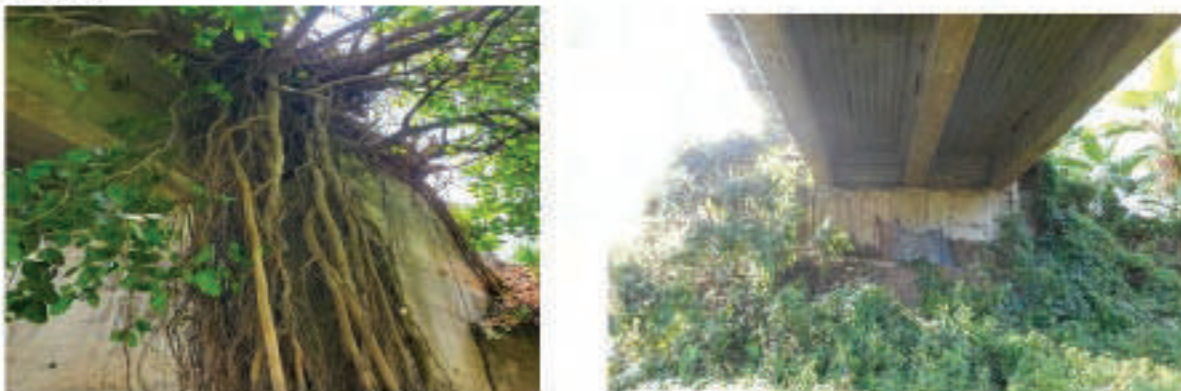
Figure 3.9: Vegetation growth that may damage the sub-structures and super-structure
