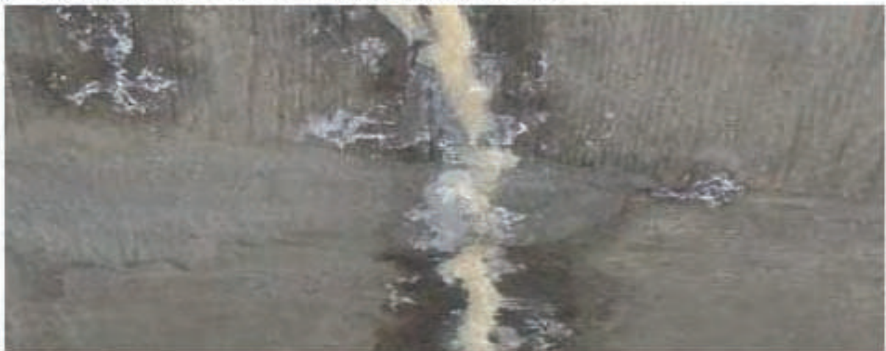
Figure 5.13: Typical Soffit Crack with Efflorescence
