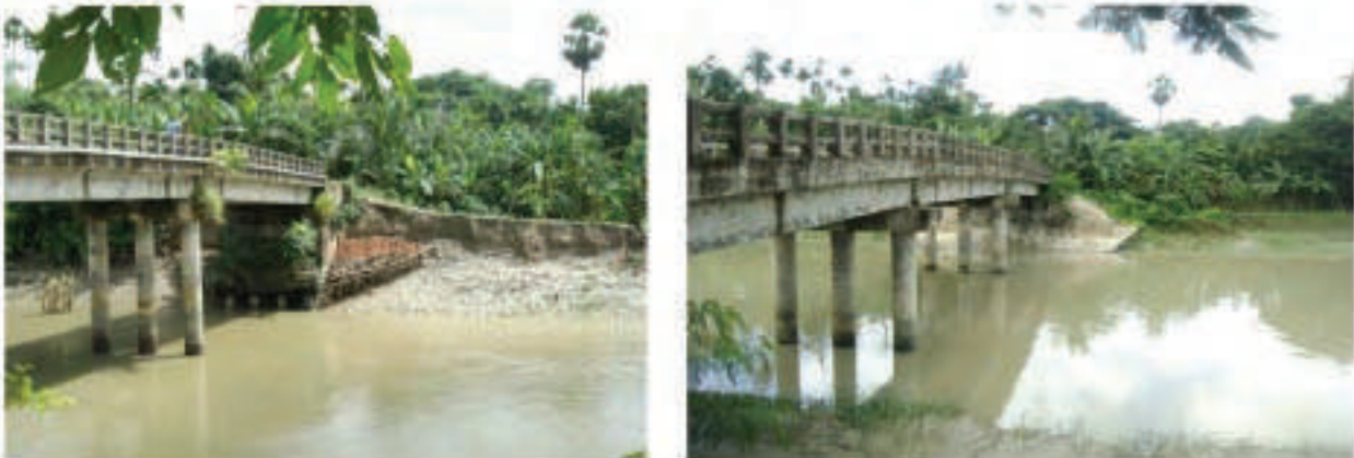
Figure 3.14: Scouring near the abutment (left), Scour prevention through maintenance (right)
