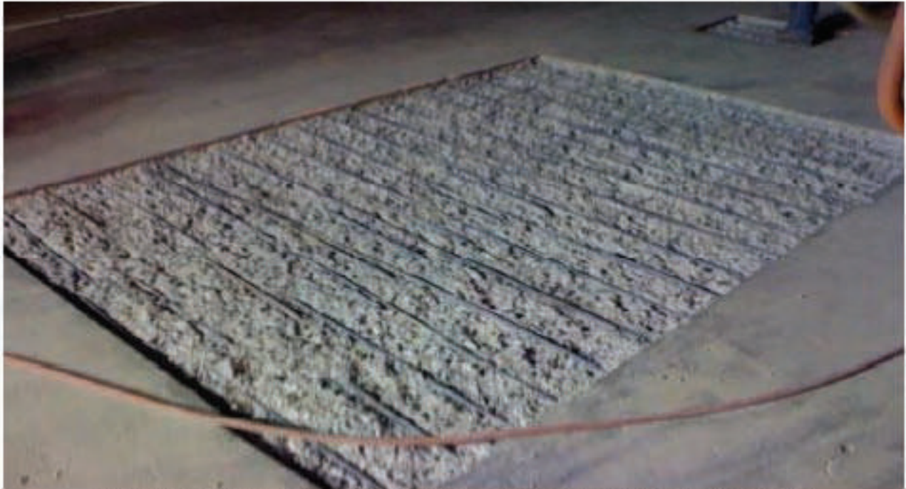
Figure 8.33: Sawcut, Chipped Out and Cleaned Concrete Removal Shown to the Top Mat Only
