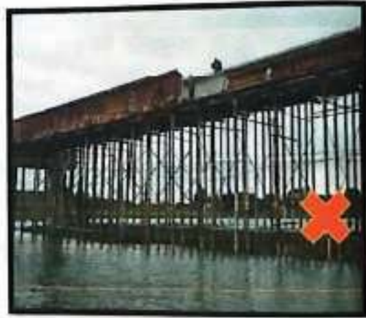
Scaffolding using Steel Prop but no Standard (Bad Practice)
