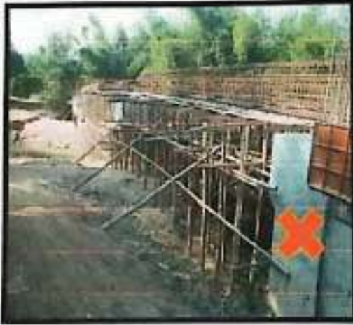
Scaffolding using Bamboo (Bad Practice)
