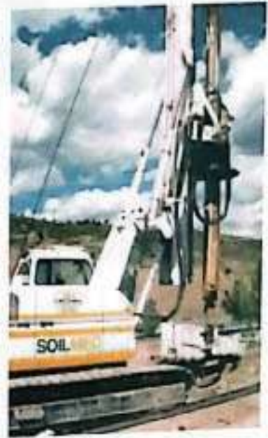
Hydraulic Powered Rig
