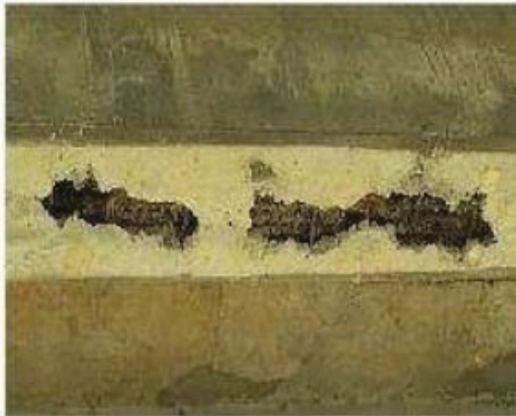
Fig 5.24.1: Girder side Require Maintenance
