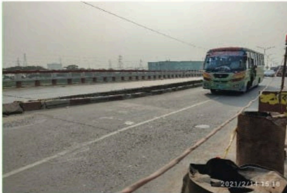
Fig 5.39.: Depression of deck
