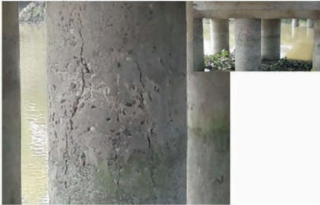
Fig 5.31.: Vertical Crack without Damage
