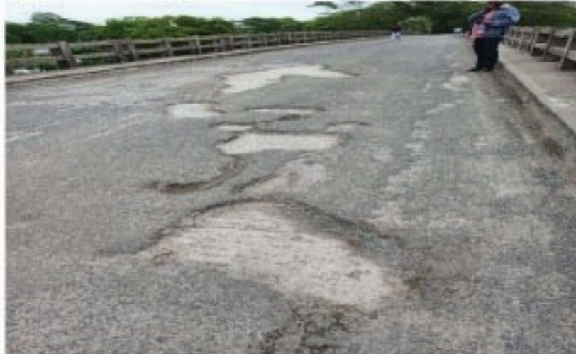
Fig: 1.18 Degradation of Deck Materials
