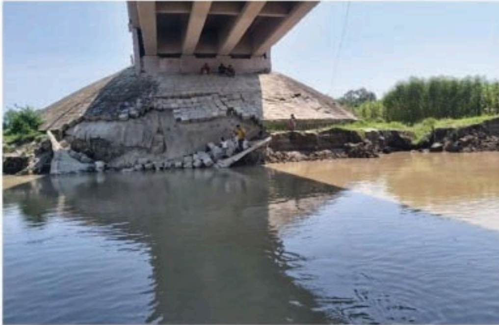
Fig: 1.15 Affected Bridge Protection work due to river bank erosion and scour
