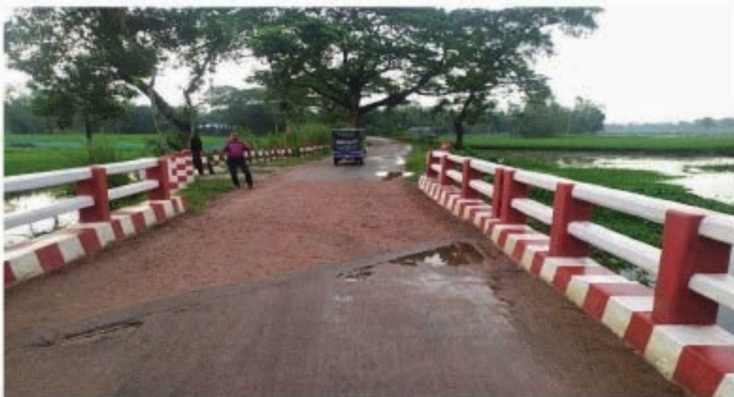
Fig: 1.17 Damage of Expansion Joint
