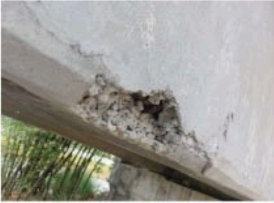
Fig 5.24.2: Concrete spalling from girder side and rebar exposed exposed.
