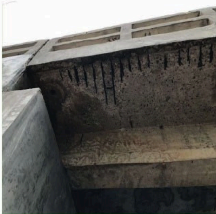
Fig 5.26.: Close view deteriorated deck slab
