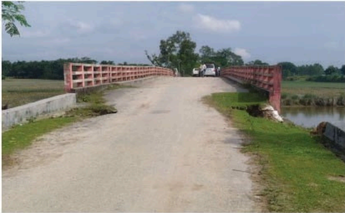
Fig: 1.16 Affected bridge approach due to precipitation
