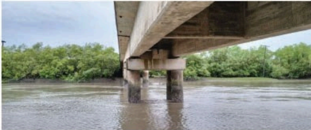
Fig: 1.13 Bridge Pier affected by Saline water
