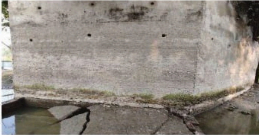
Fig 5.21.1 Concrete surface having fine honeycomb
