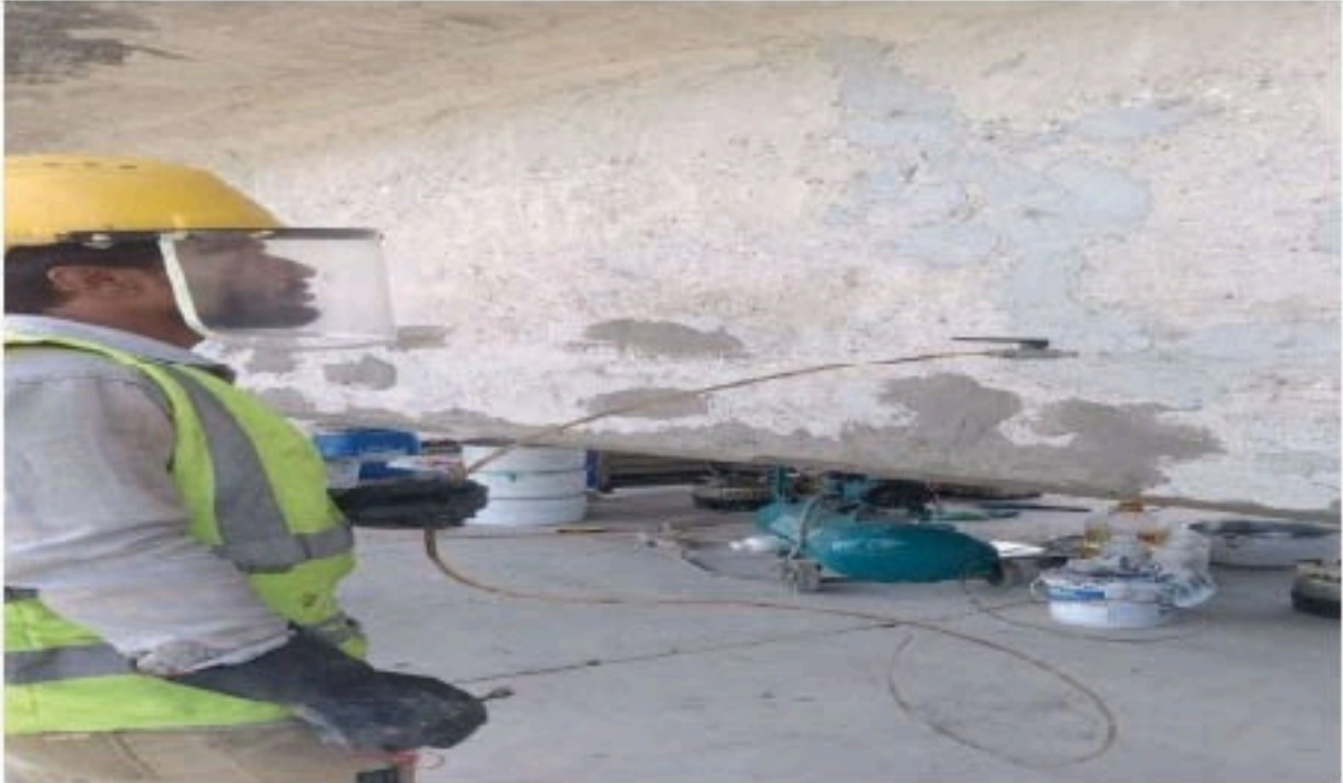
a) Micro Concrete: It is flowable high strength concrete. It is use where normal concreting is difficult. For maintenance work micro concrete is very effective. (Photo Attached)
