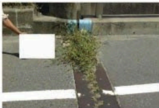
Fig.5.3 Blocked expansion joint
