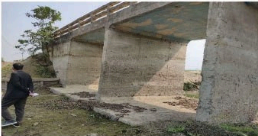
Fig 5.21.2 Concrete surface having fine honeycomb
