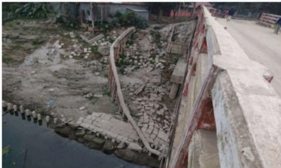
Fig: 1.8 Bridge Protection work affected by Flood.
