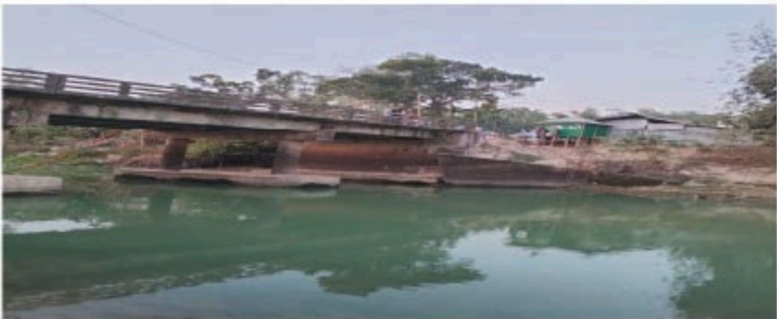
Fig: 1.2 Bridge affected by River bank Erosion
