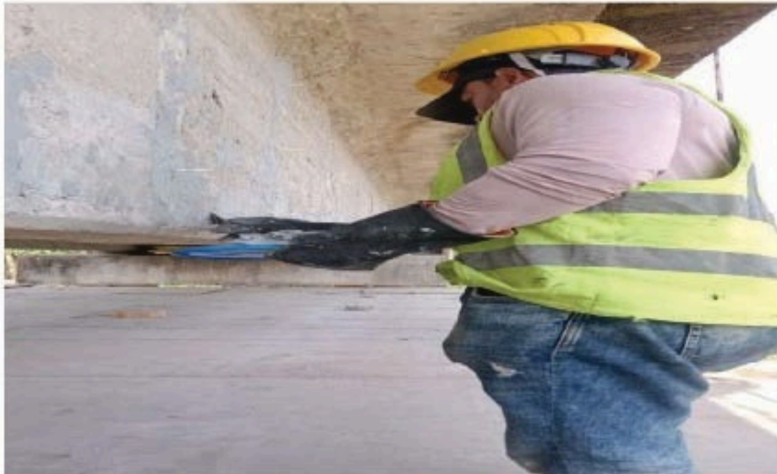
b) Injected epoxy resin: Epoxy resin injection using pressure injection machines to seal crack and prevent further deterioration. (Photo Attached)
