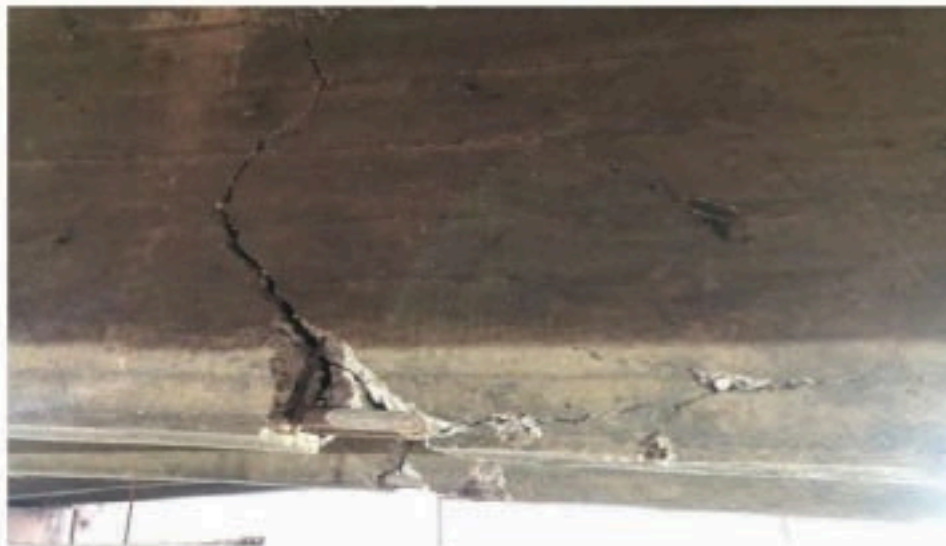
Fig 5.40.: Flexural crack of girder
