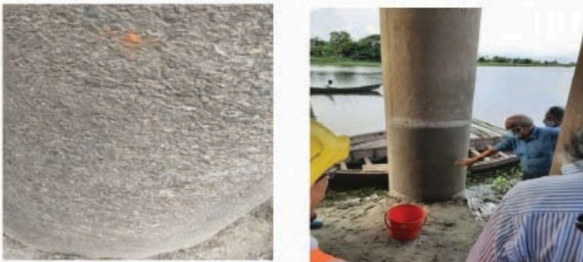
Figure 5.12.: Polymer Mortar Application before and after condition
