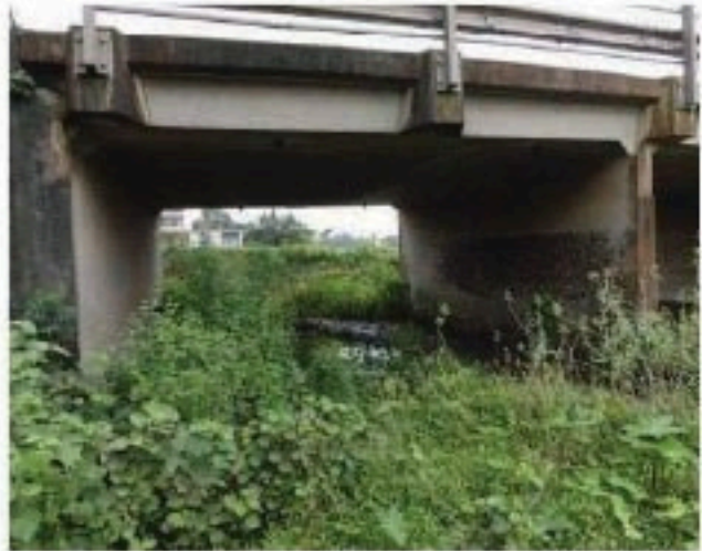
Fig. 5.10. Harmful weed under the bridge
