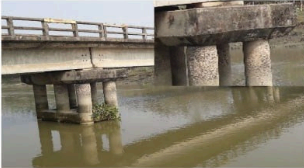
Fig 5.29.: Corroded concrete pier without exposed rebar
