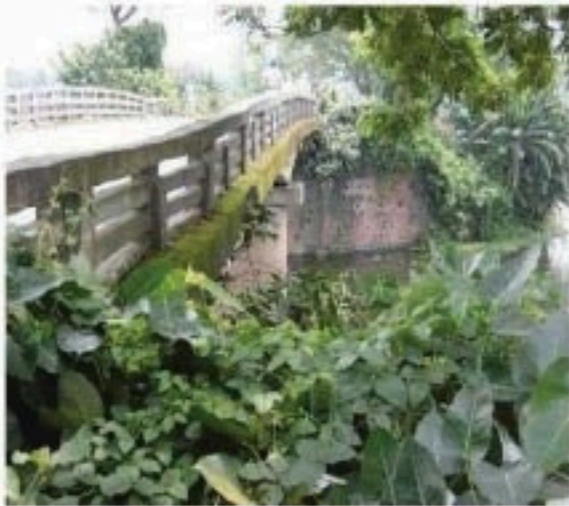
Fig.5.9. Harmful weed around the bridge
