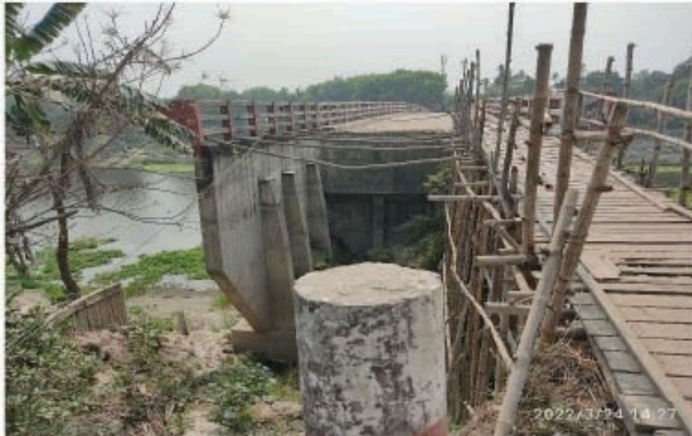
Fig: 1.14 Landslides in bridge approaches due to heavy rainfall
