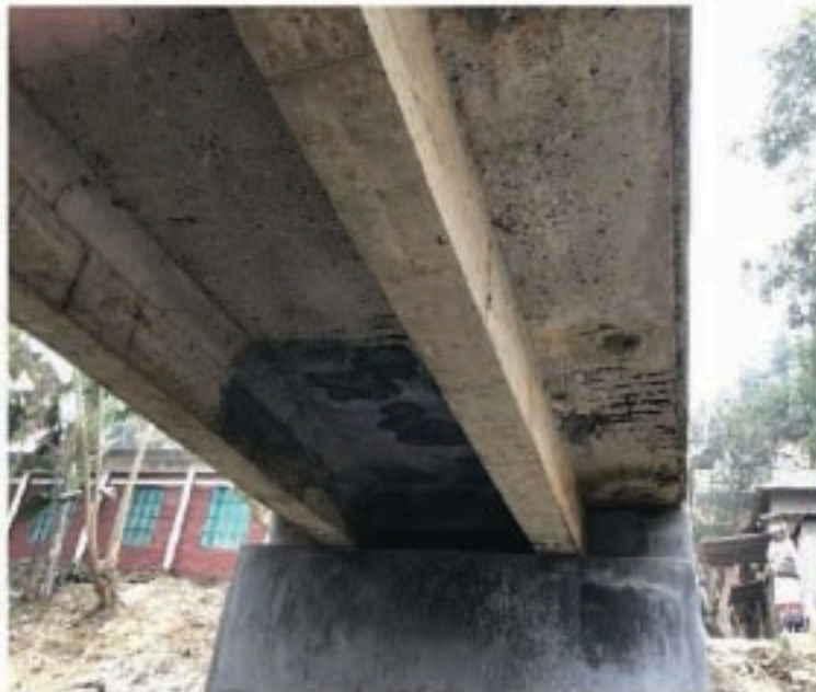
Fig 5.25: Deteriorated deck slab
