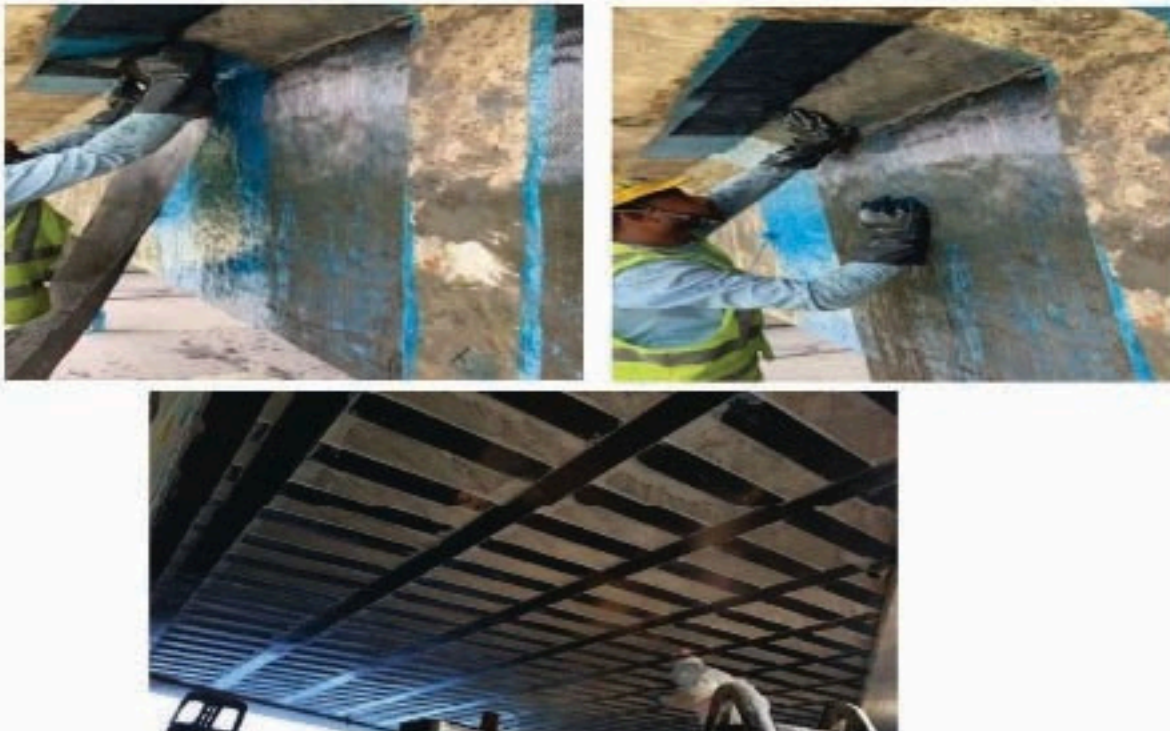
Fig: 5.14 Apply epoxy putty at the bottom face of the girder and place Carbon laminate without any air gap
