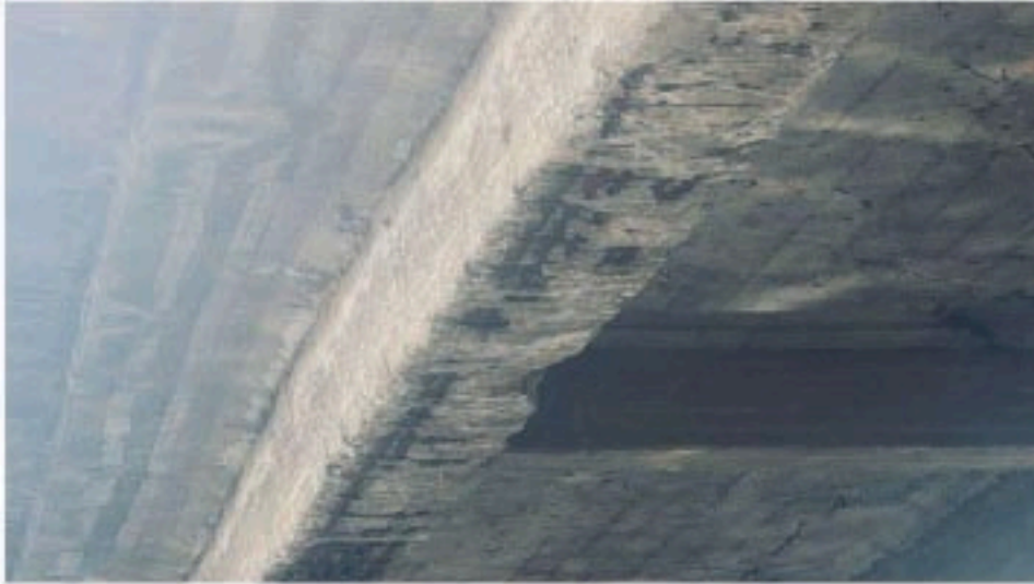
Fig 5.36.: Rebar Exposed In Girder
