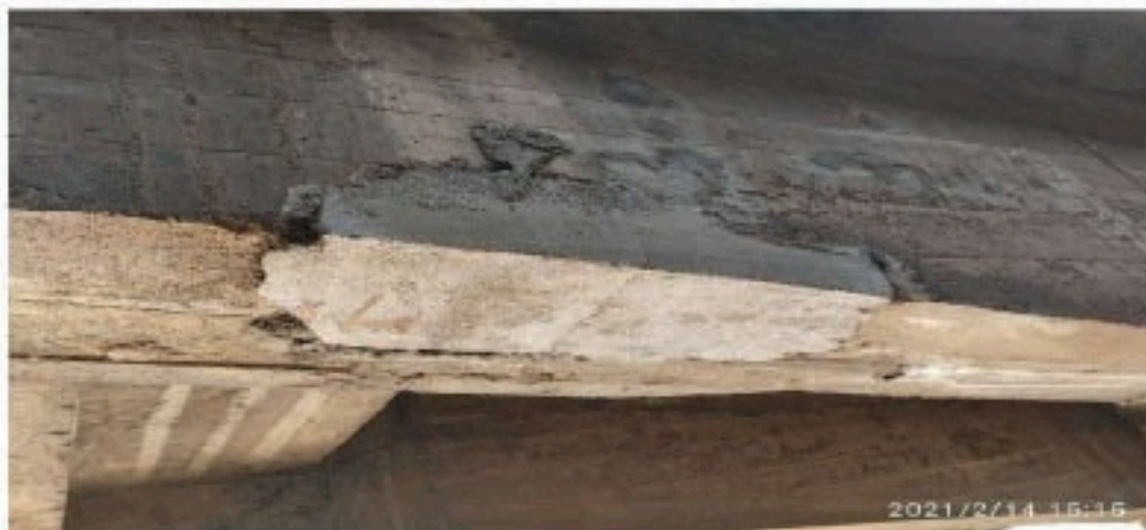
Fig 5.41.: Concrete cavity filled by micro concrete and epoxy injection apply epoxy putty at the bottom face of the girder and place Carbon laminate without any air gap.
