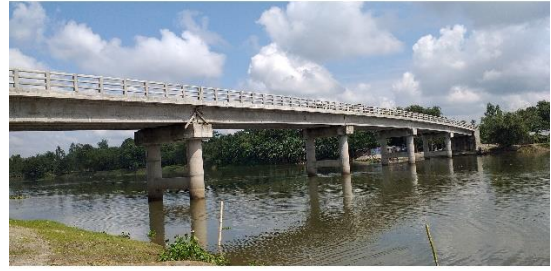
Construction of 135 m PC Girder Bridge on Uharla River (Ghat-Fulbari Upazilla HQ. Via Boshpechai C/tnohel Road (Road ID-152554155) at Chainage-400m, under Sadar Upazilla, District Lalmonirhat.
