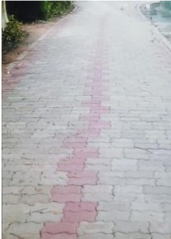
Rehabilitation of Sreefaltala UP Bou Bazer Road from Ch. 00m - 420m (e-tender/LGED/Khul/GOBM/22-23/W-50) Road ID: 247754045
