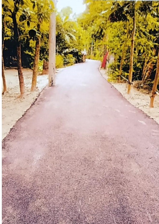
Improvement of Alipur Moin Sikder house - Sheraj Sikder house road from Ch. 600m - 1183m (KBS-RIDP / KHUL/VR-15.4/18-19) Road ID: 247755259
