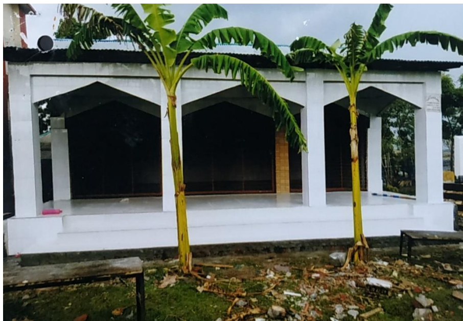
Improvement of KaminibashiaK.G.V.J Shommeeloni Girls school Mondir Under Tildanga Union, Dacope upazila (GSID-2/KLN/DW-26)
