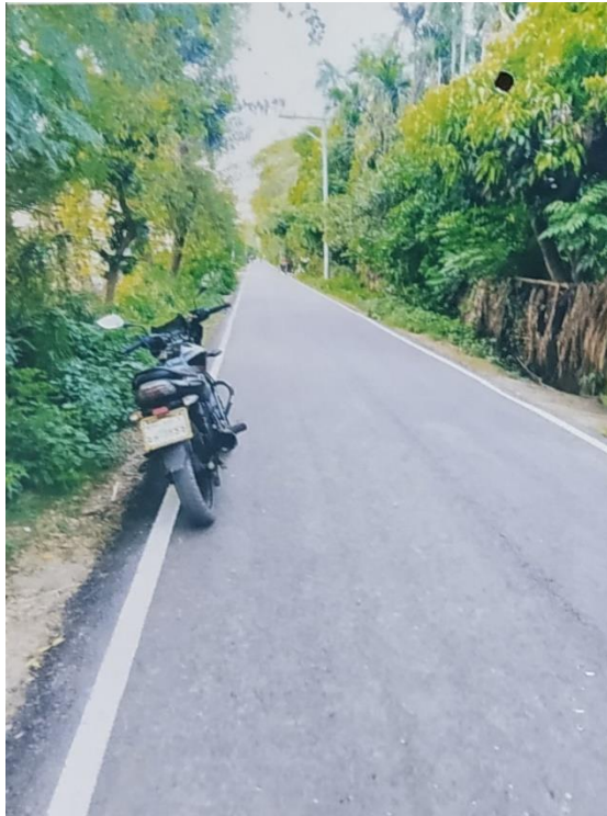
Road ID- 247942004 Rehabilitation of Abduler more R & H-Majhigati GC via Kola Bazar Road Terokhada portion) Road from Ch. 00-6080m Under Terokhada Upazila (CAFDRIRP/Khul/UZR/W-16/2022-23)
