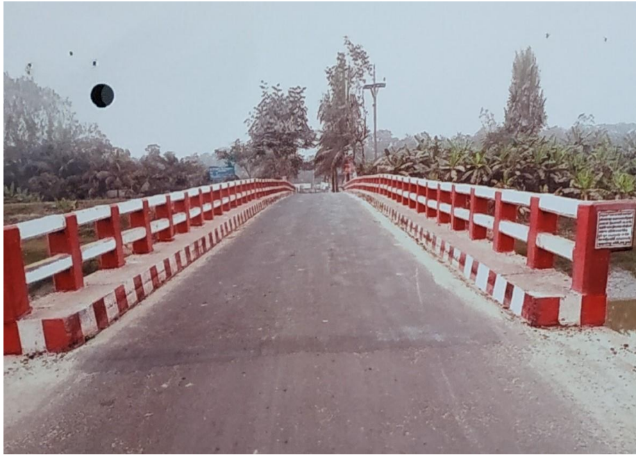
Major maintenance of 42.7m long RCC Girder Bridge on Thana H/Q-Alaipur hat-Sheikhpura GC (Rupsha Portion) at ch 1784m [SupRB/Khul/Maint/21-22/W-266]
