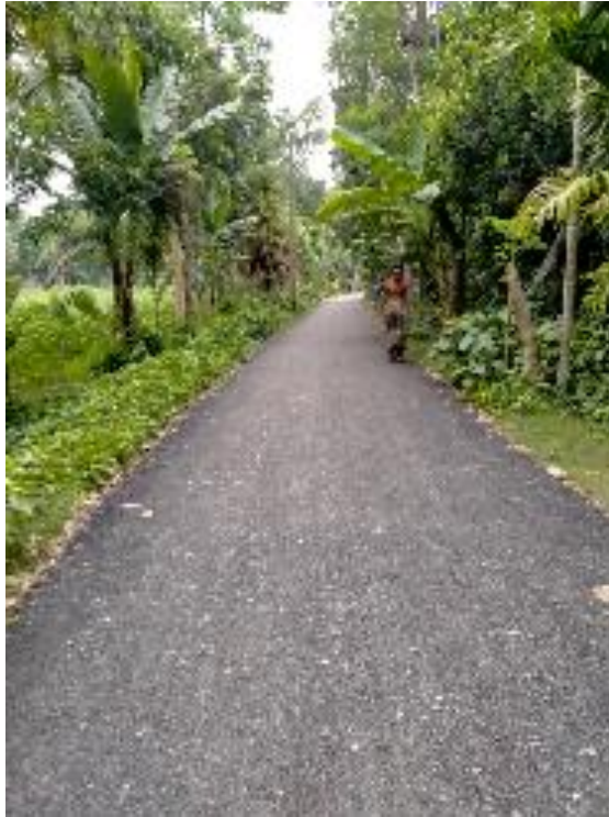
Improvement of Kashimnagor shop of Amjad BC road-Ramnagorvia house of Yeakub & house of Radha Saduat (Ch.1000m-3000m) Road ID: 247644060 (IRIDP-3 DW-27)
