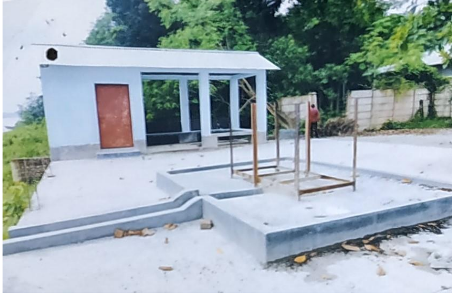
Improvement of Gilatala Dakhin Para Thakur Ghat Shosan under Atra Gilatala Union, Phultala Upazila (GSID-2/KLN/DW-50)
