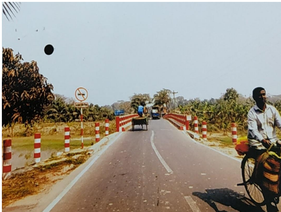
Major maintenance of 42.7m long RCC Girder Bridge on Thana H/Q-Alaipur hat-Sheikhpura GC (Rupsha Portion) at ch 1784m [SupRB/Khul/Maint/21-22/W-266]
