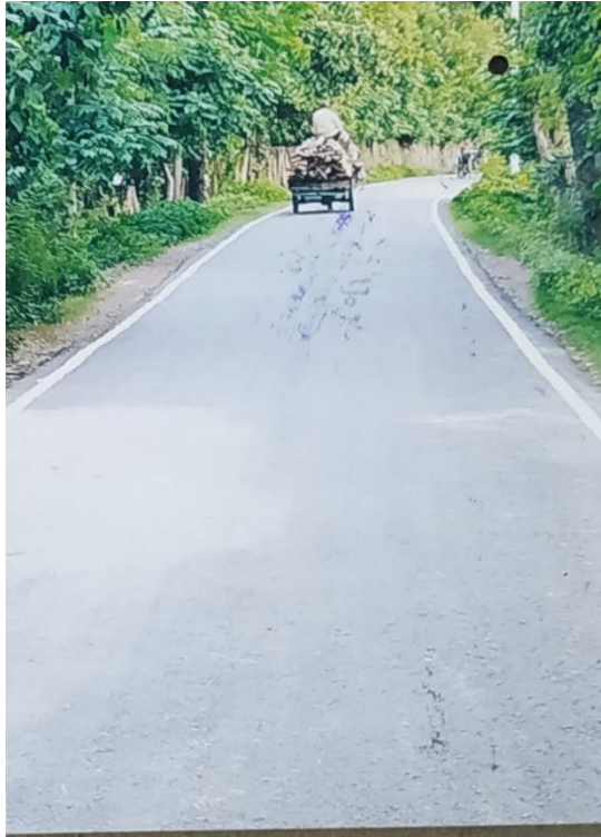
Road ID- 247942004 Rehabilitation of Abduler more R & H-Majhigati GC via Kola Bazar Road Terokhada portion) Road from Ch. 00-6080m Under Terokhada Upazila (CAFDRIRP/Khul/UZR/W-16/2022-23)
