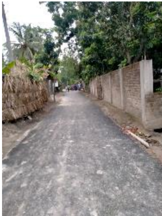
Improvement of Kashimnagor shop of Amjad BC road-Ramnagorvia house of Yeakub & house of Radha Saduat (Ch.1000m-3000m) Road ID: 247644060 (IRIDP-3 DW-27)
