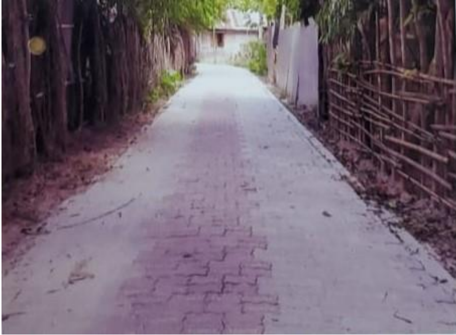
Rehabilitation of Paygram kashba judge Rd road from Ch. 00m - 1250m (e-tender/LGED/Khul/GOBM/22-23/W-40) Road ID: 247694026
