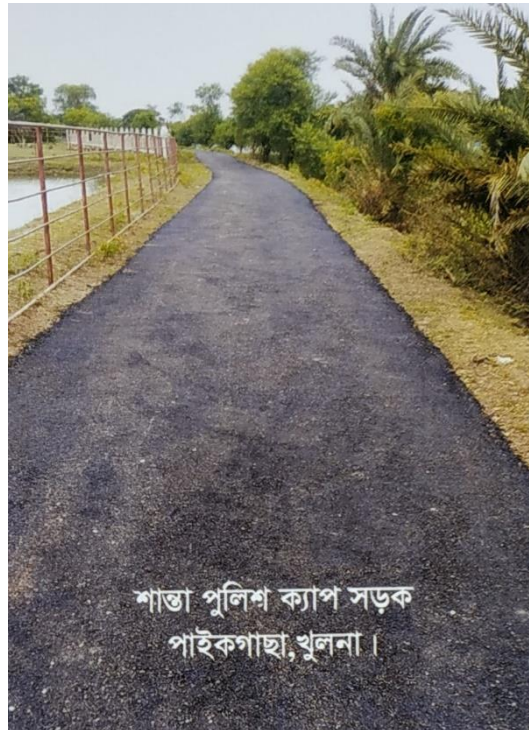
Improvement of Santa Bazar-Khatalata bridge via Bainbaria High school & Police camp Road at Ch. 5300 - 6800m (KBS-RIDP / KHUL/VR-17.1/19) Road ID: 247644044
