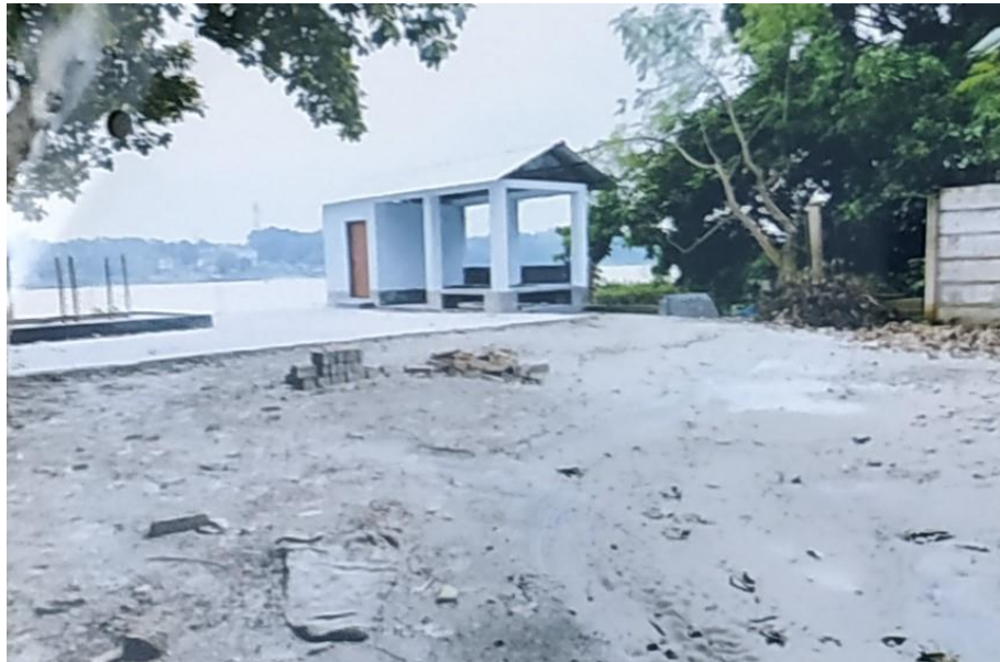
Improvement of Gilatala Dakhin Para Thakur Ghat Shosan under Atra Gilatala Union, Phultala Upazila (GSID-2/KLN/DW-50)
