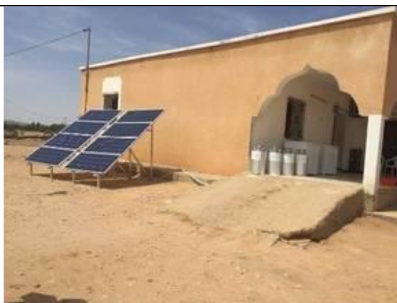
Solar milk chillers in Tunisia
