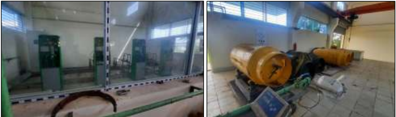
Figure 69: Chemicals stored safely and dispensed using automated meters (BWTP).
