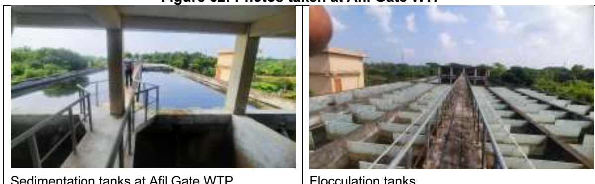
Figure 62: Photos taken at Afil Gate WTP
