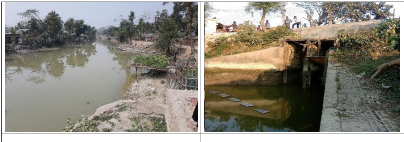
Figure 3.34 Site Condition of Labonchara 2 Khal (upgrading of outlet gate and a new PS)
