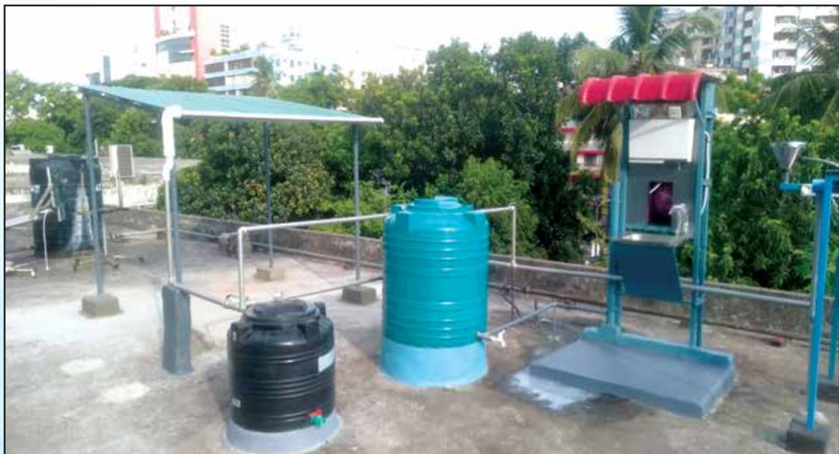
3. Rain Water Harvesting System
