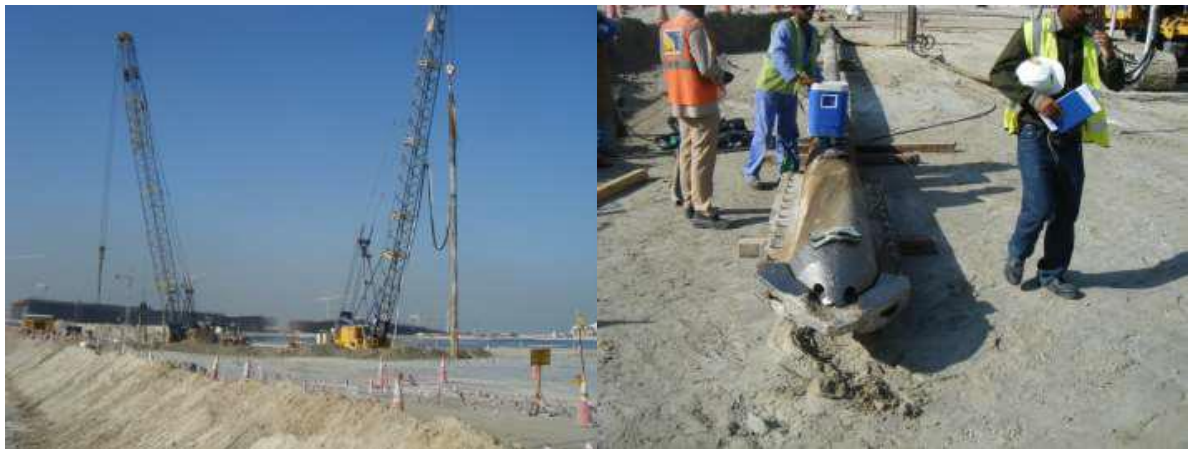
Vibrio Compaction - Fill behind Quay
