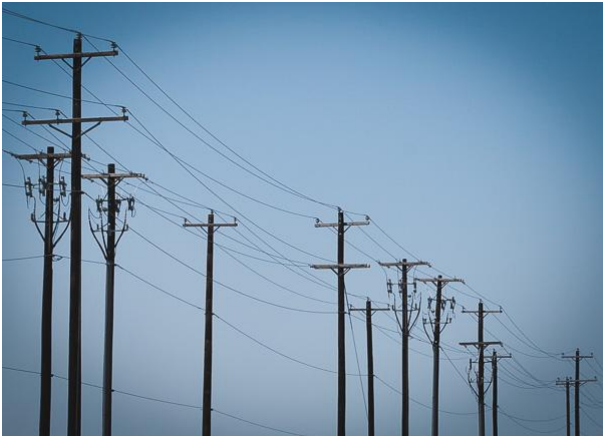
Figure 66: Distribution lines through a countryside of Bangladesh
