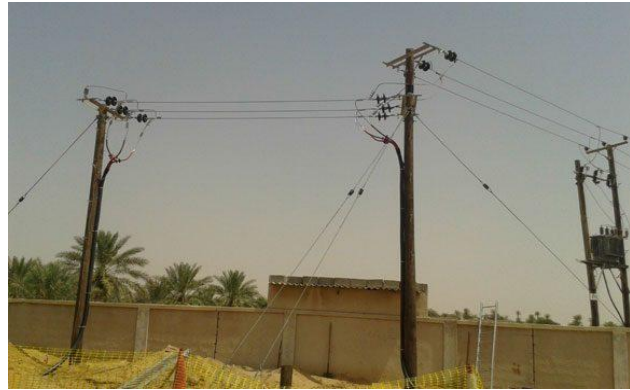
Figure 100: Electric Power Distribution Line
