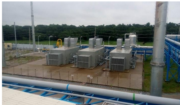
Figure 25: Gas Booster Compressor
