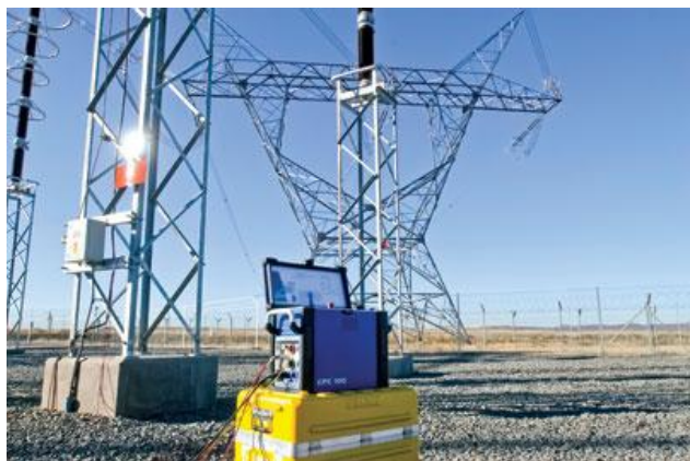
Figure 48: Transmission Line Testing
