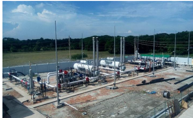
Figure 24: Regulating and Metering Station (RMS)
