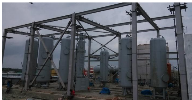
Figure 33: Water Treatment Plant
