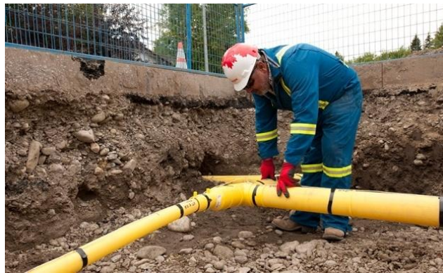
Figure 101: Gas Distribution Line
