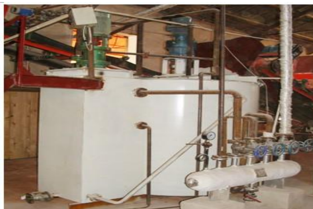
Figure 86: Urea Melt Spraying Machine
