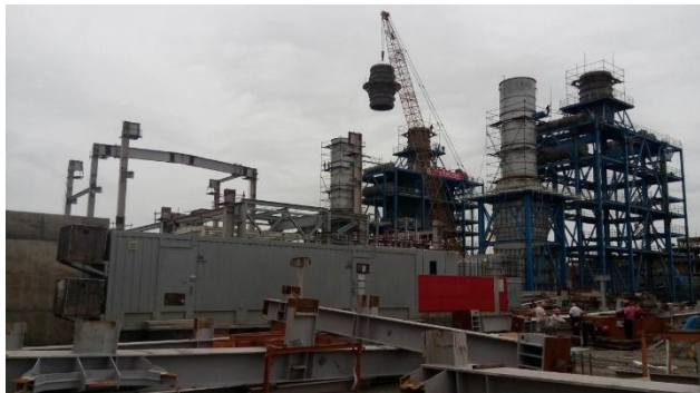
Figure 30: 60 Meter Height Main & Bypass Stack
