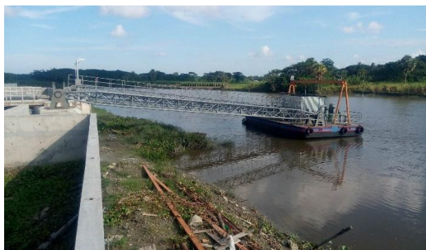
Figure 32: Water Intake Station at River
