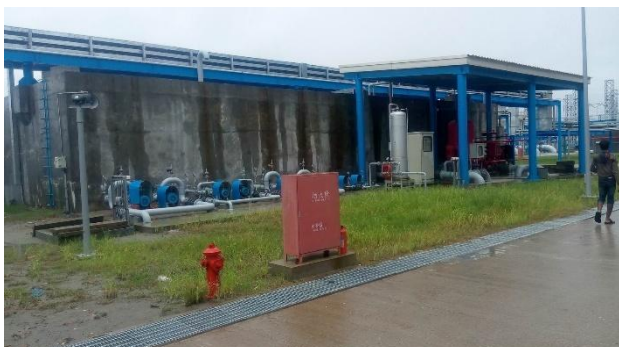
Figure 35: Firefighting station & Hydrant
