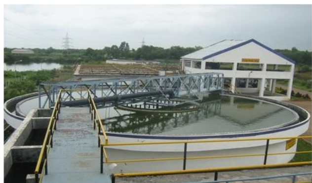
Figure 104: Central Effluent Treatment Plant
