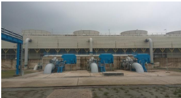
Figure 34: Mechanical Draft Cooling Tower
