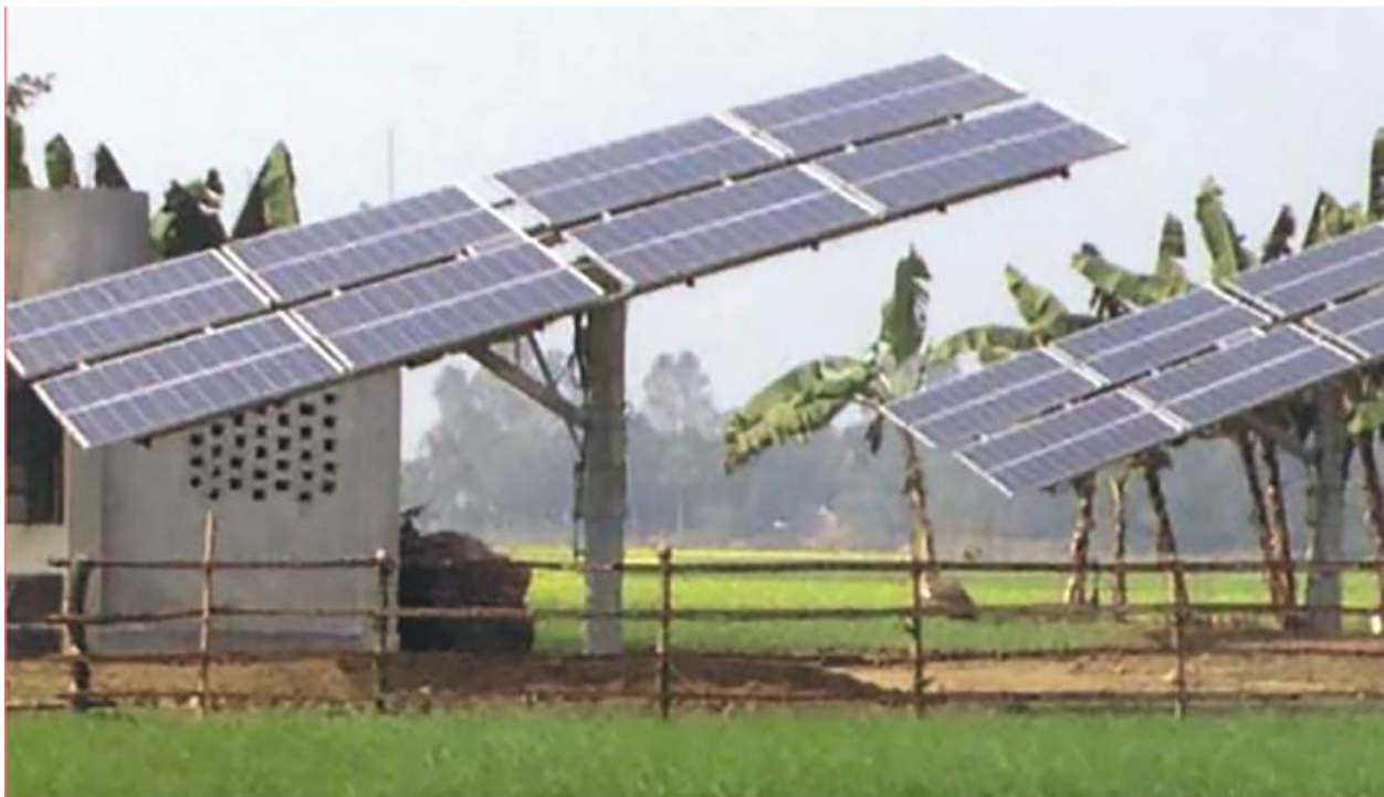
Double-axis tracking. Solar irrigation pump systems using manual double-axis tracking standers (photo provided by Asian Development Bank consultant).
