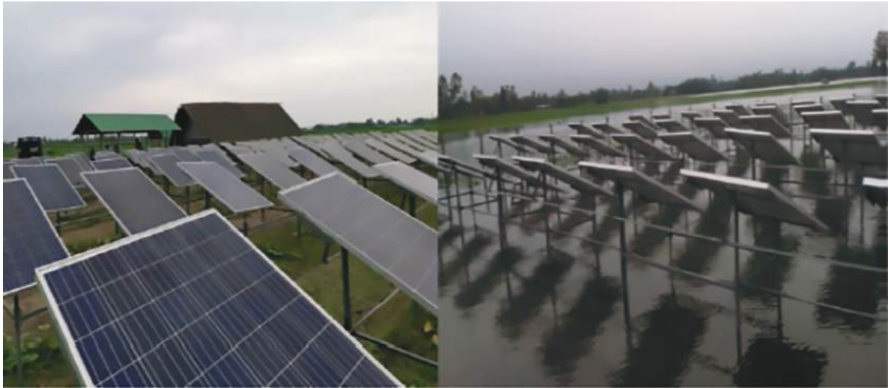
Single-axis tracking. Solar irrigation pump systems using manual single-axis tracking standers (photos provided by Asian Development Bank consultant).
