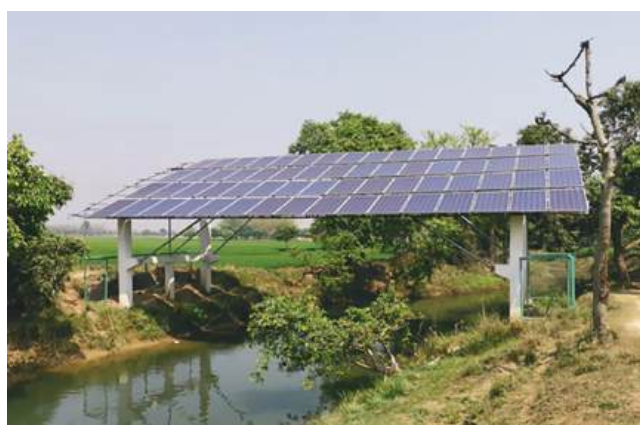
Photovoltaic module over water storage. A photovoltaic module array of a pump system in the Barind region (photo provided by Asian Development Bank consultant).
