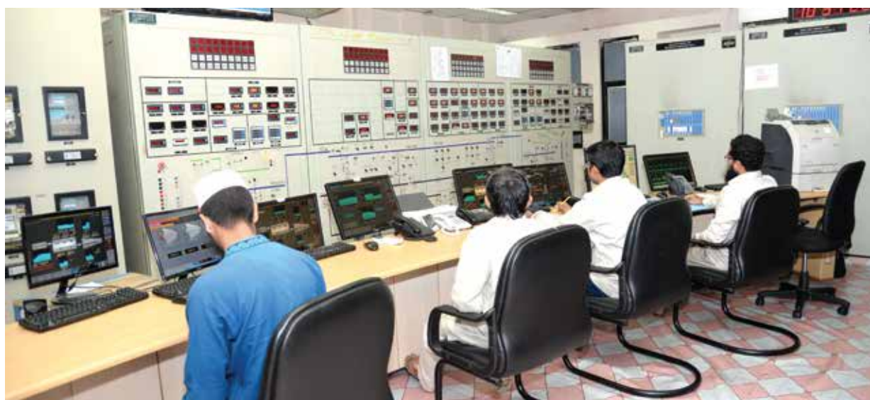
Control Room of Siddhirganj 2x120 MW PPP
