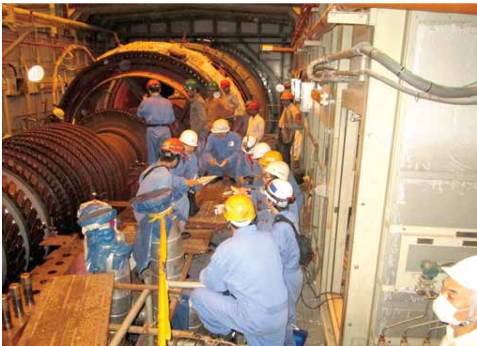
Gas Turbine Rotor Run out Checking
