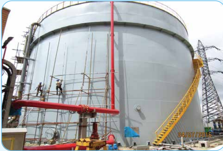
Clarified water storage tank (paint working)
