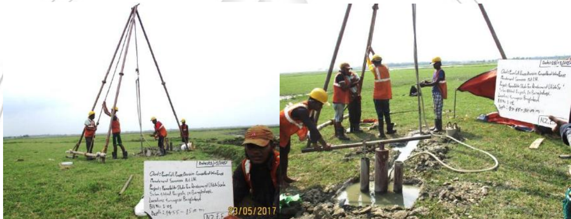
FIG-2. Soil exploratory boring for the Feasibility Study for Development Utility Scale Solar & Wind Projects at Sonagazi near Choto Feni River in Bangladesh.
