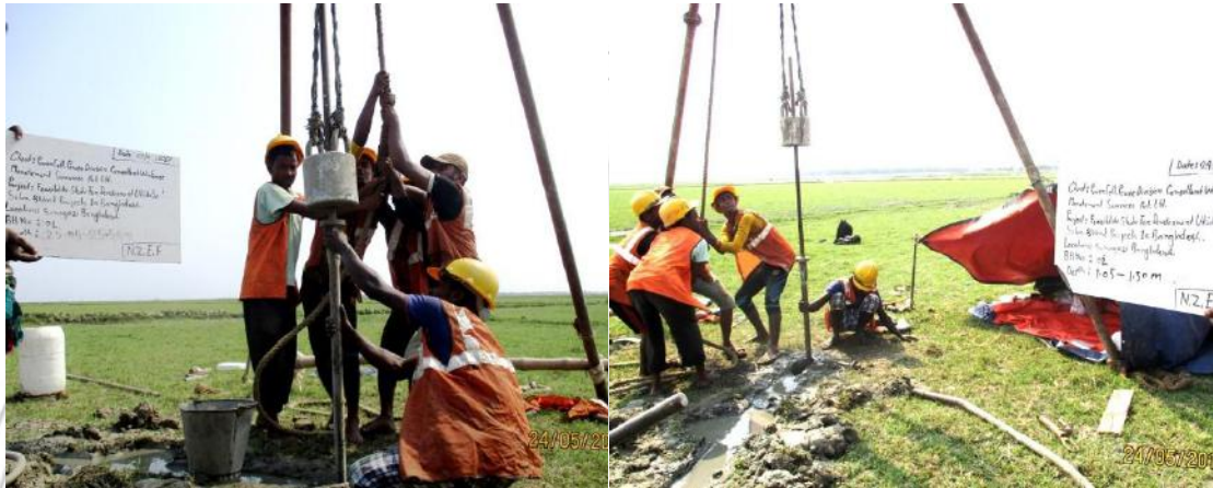
FIG-3. Standard Penetration Test for the Feasibility Study for Development Utility Scale Solar & Wind Projects at Sonagazi near Choto Feni River in Bangladesh.
