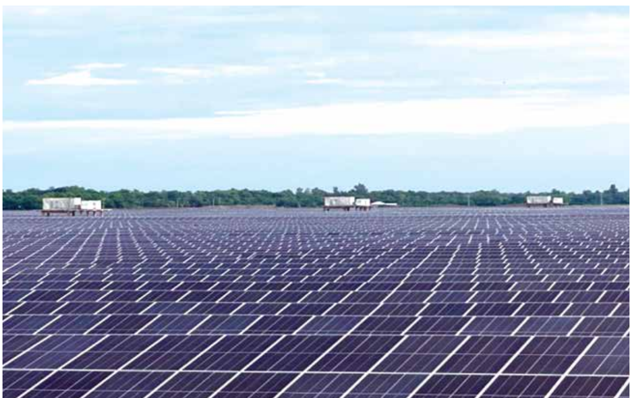
PV panels at Sonagazi 75 MW Solar Power Plant Construction Project
