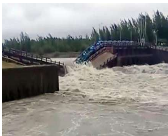
Figure 4.20: Damaged Musapur Regulator.
