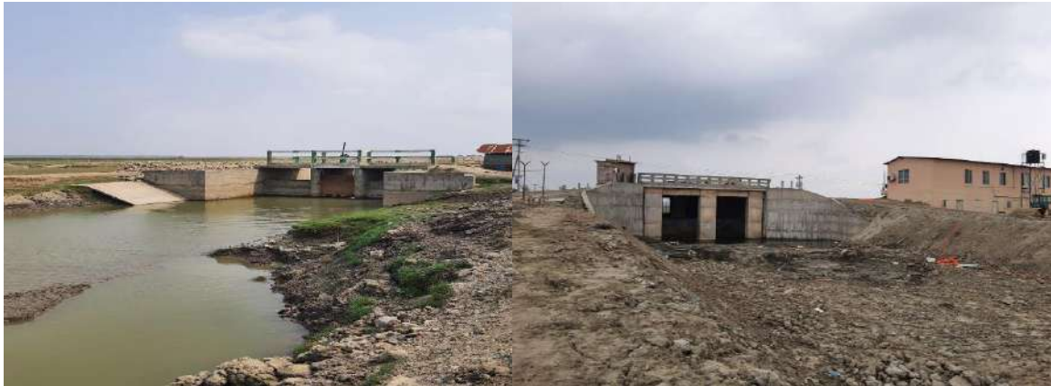
Figure 4.22: Sluice Gate on Masjid Khal, Purbo Baradhali mauza, Char Chandia.
