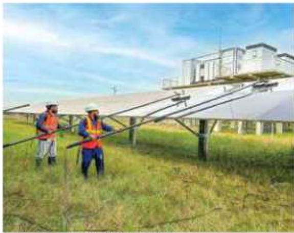
Solar Panel Cleaning
