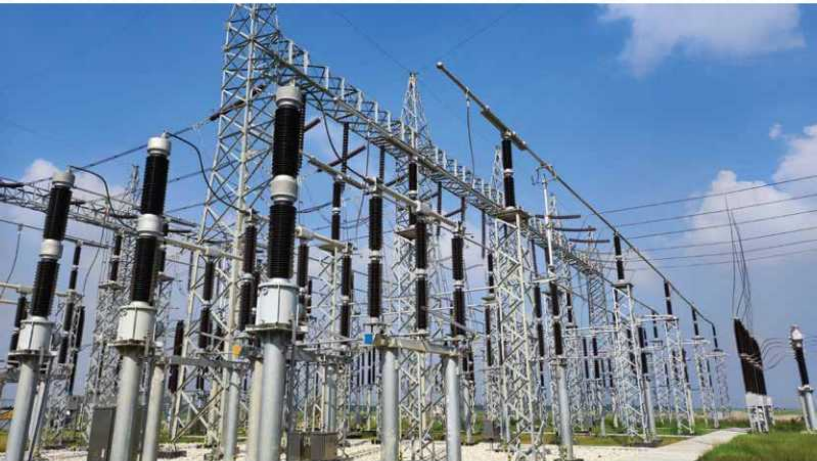
Grid Substation at Sonagazi, Feni
