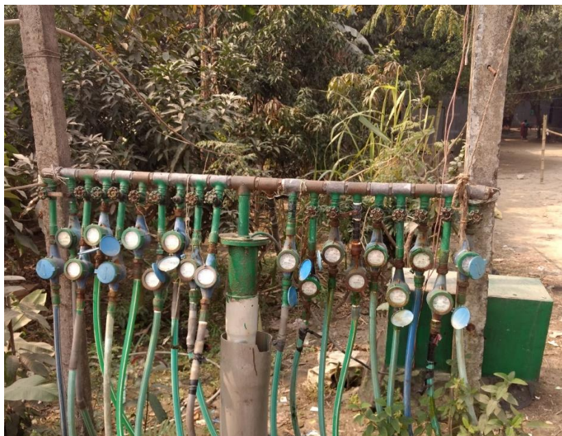
Figure 4: Community Pump with Spaghetti Pipes (at Nasirabad)
