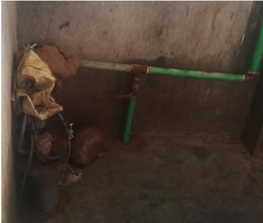
Figure 3: Motor Pump in a House at Alubdi Area of Harirampur Union
