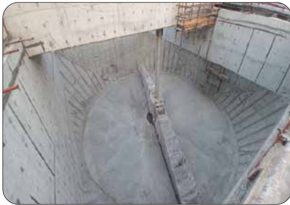
Figure 7: W20_Densadeg Sedimentation Chamber
