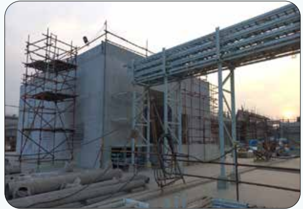
Figure 14: W81_Main Electrical Building
