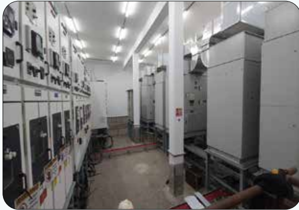
Figure 13: W81_Main Electrical Panels
