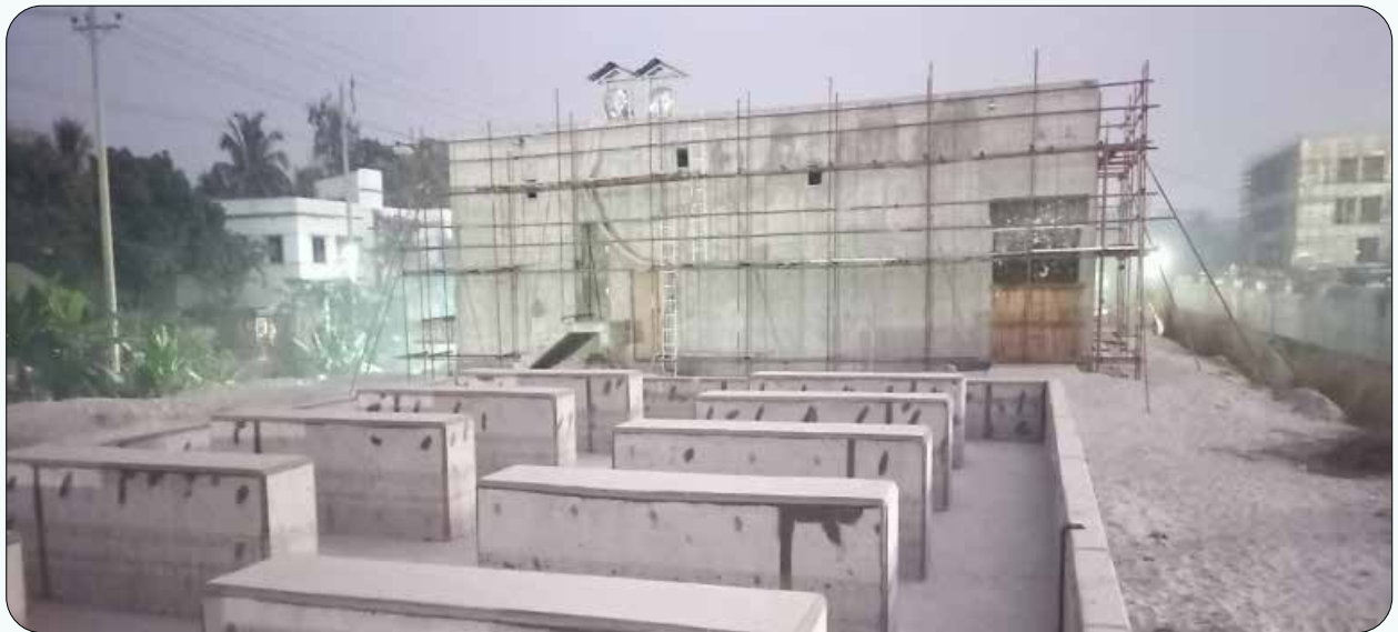
Figure 15: W82_Generator & W83_Fuel Storage
