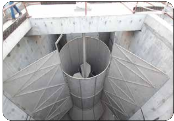
Figure 8: W20_Densadeg Flocculation Chamber
