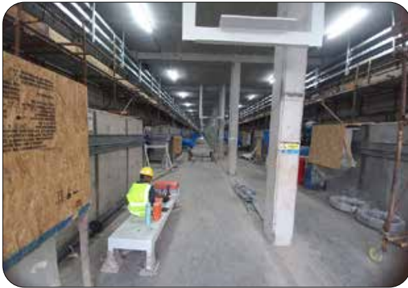
Figure 1 : W30_Gravity Filter Pipe Gallery
