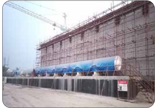
Figure 20: W45_Pump House With Delivery Discharge Pipe
